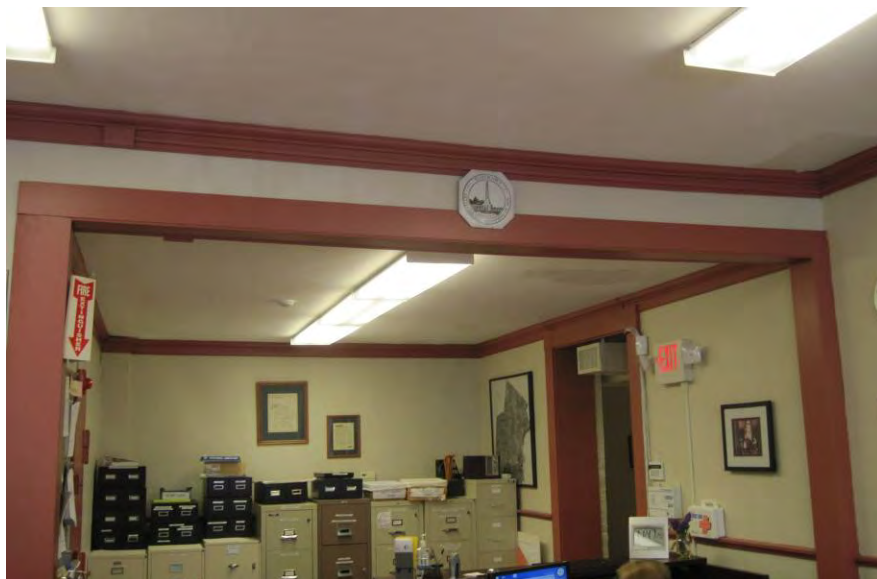
Figure 48. Bowing header beam at Town Clerk's office
