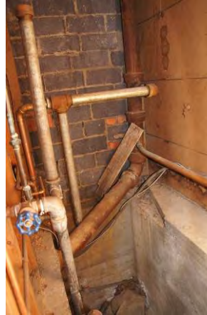
Figure 62. Plumbing pipes behind south stairs.
