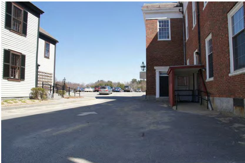
Figure 73. North driveway and asphalt butts right up against the building.
