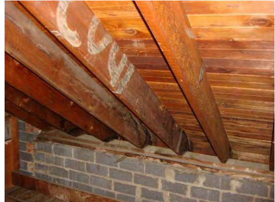
Figure 19. Roof rafters at north and south wings bear directly on blocking and cinder block exterior wall.
