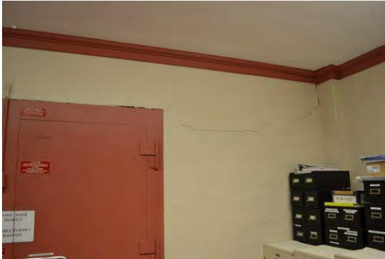
Figure 56. Cracked plaster at vault wall at Town Clerk.
