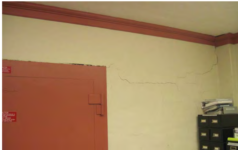
Figure 3-Plaster Cracks at First Floor Vault
