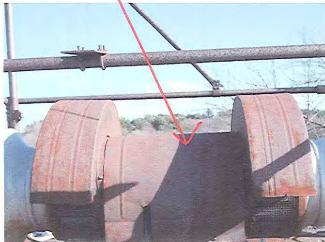
SIREN HORN & PIPING ATOP CHIMNEY
