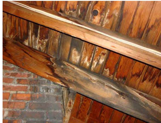
Figure 30. East chimney showing signs of water infiltration.
