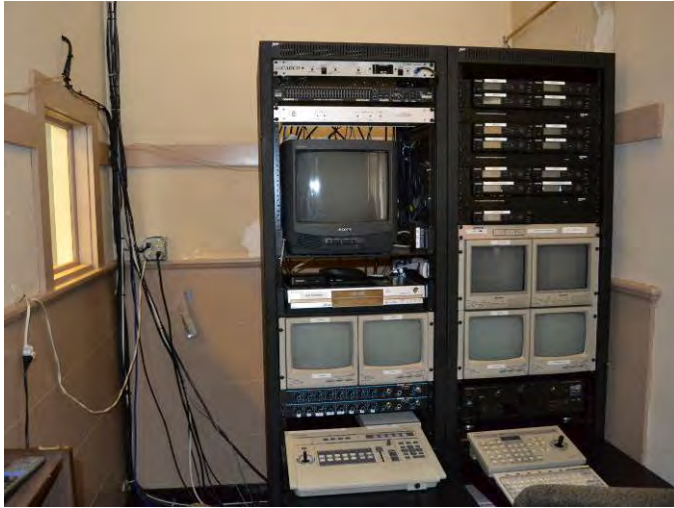
Equipment rack in Cable Studio
