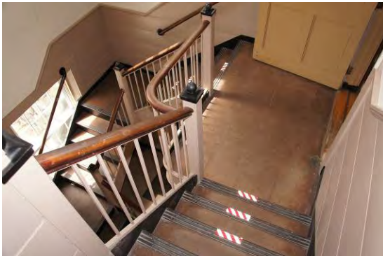
Figure 79. Possibly asbestos tile at south wing stairs.
