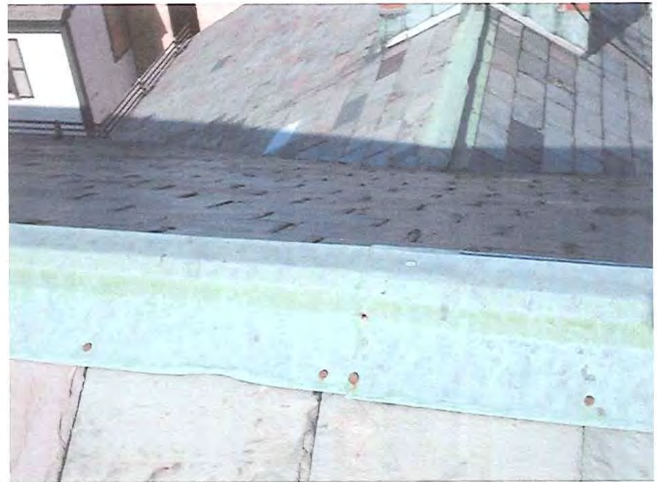
VEIW OF COPPER RIDGE VENT W/COMMON ROOFING NAILS
