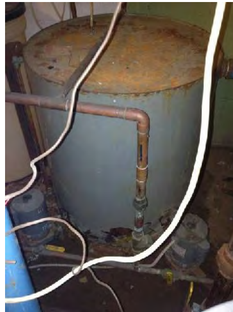
Figure 2- Existing Cond. Receiver
