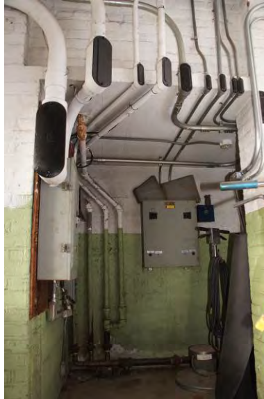
Figure 68. Existing electrical room in basement.
