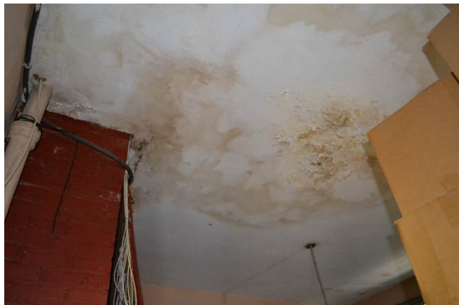
Figure 60. Water damage at Historical Society office in north wing.
