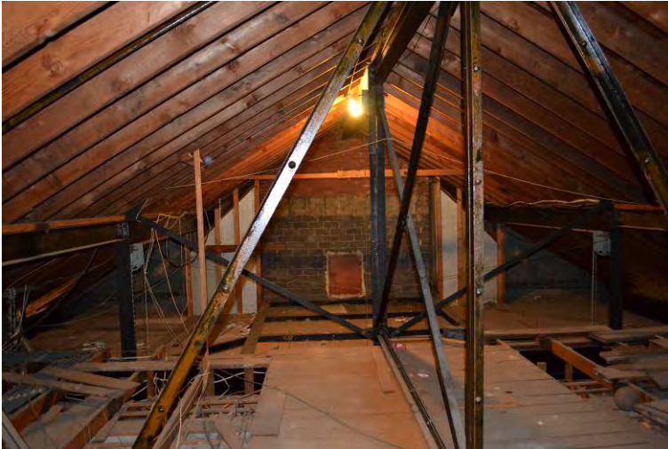
Figure 17. View of roof steel trusses, steel beams, wood rafters and cinder block chimney beyond.
