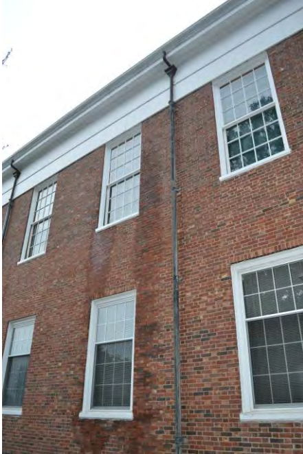
Figure 24. Leaking south copper gutter.
