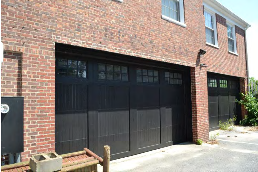
Figure 26. Damaged brick at lintel of garage door.
