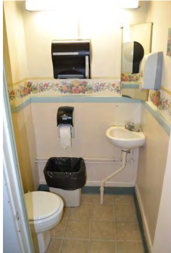
Non-code compliant 2 nd floor restroom
