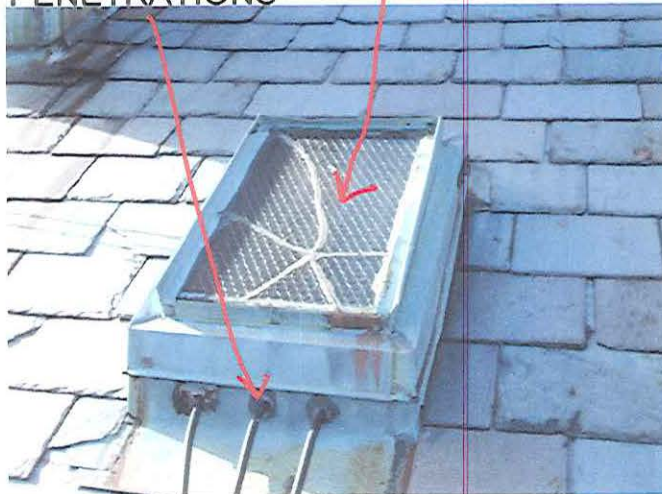
SKYLIGHT; CRACKED LENSE, LOOSE PENETRATIONS
