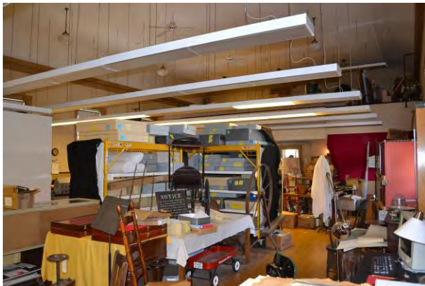
Figure 69. Strip florescent lighting in auditorium
