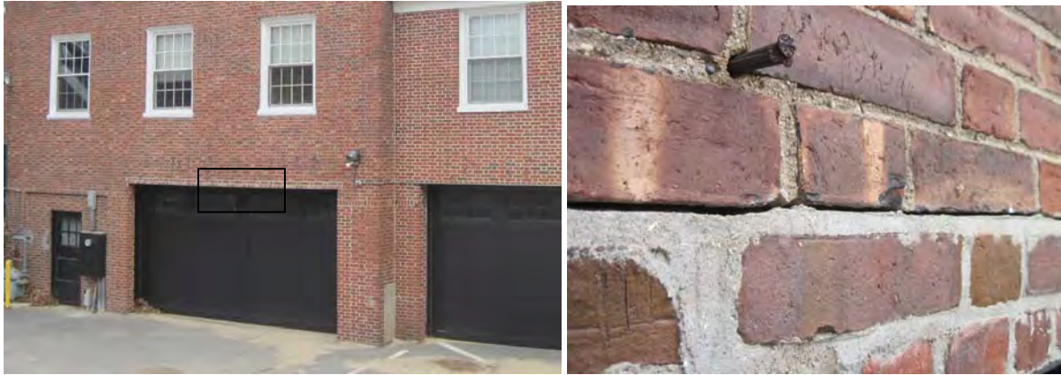
Figure 2-Expanded Fire Station Door and Masonry Separation
