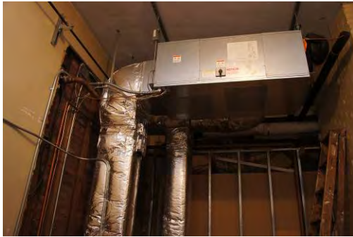
Figure 65. Air conditioning for Town Clerk's office.
