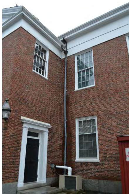
Figure 25. Leaking downspout at north wing.
