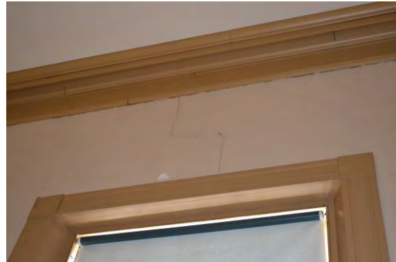
Figure 57. Stepped crack in plaster above window in auditorium.
