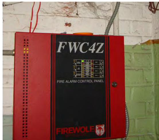
Figure 71. Fire alarm equipment
