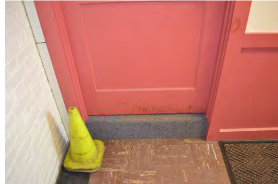
Figure 80. Possible asbestos tile at 1955 addition entry hall.
