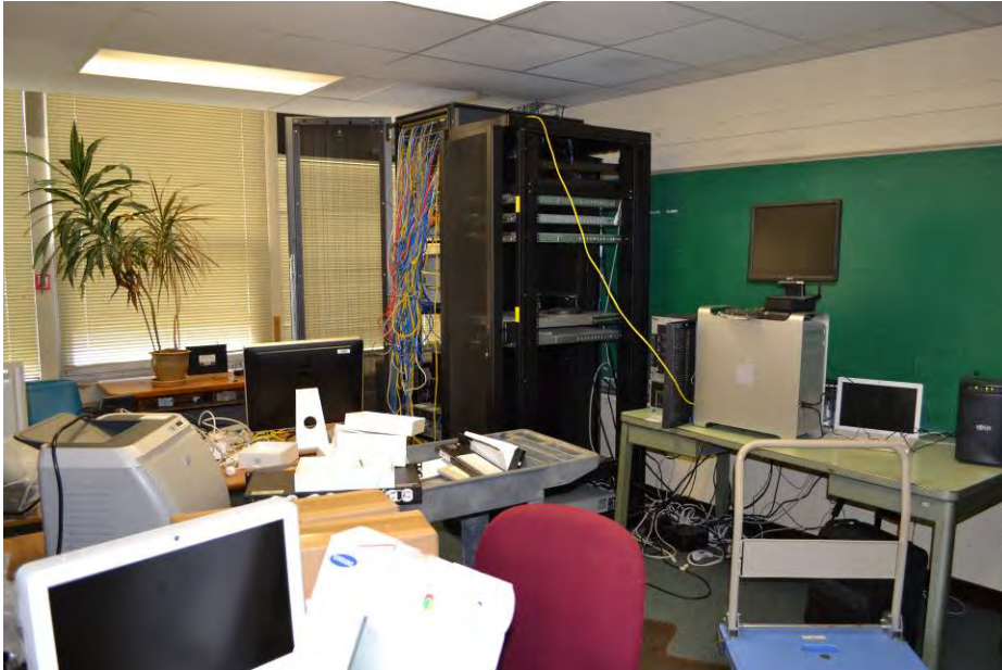
Server and work area
