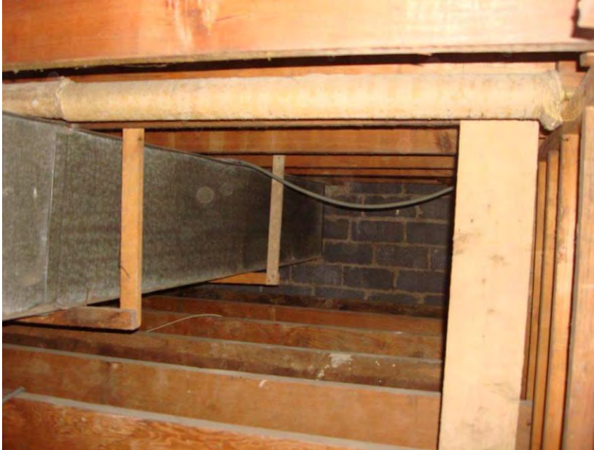
Figure 14. First floor ceiling framing below and second floor stage framing above with a duct in the plenum space that runs to the east exterior wall.
