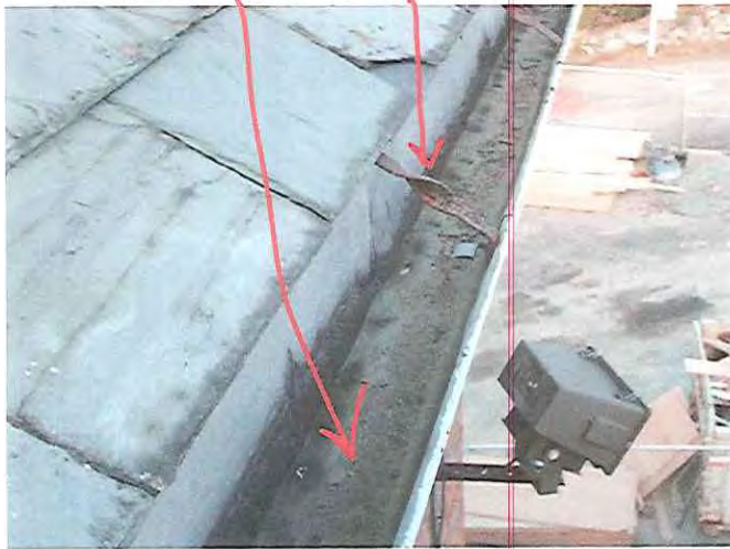
VIEW OF LEFT REAR GUTTER; [COPPER] LINED W/TAR, RUSTED STEEL HANGER
