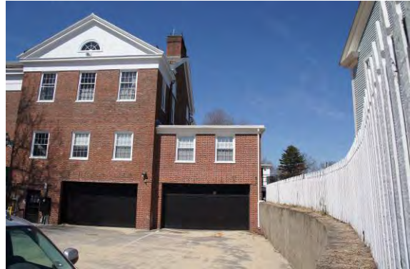
Figure 75. Concrete retaining wall at south side of Town Hall next to Loring Parsonage.
