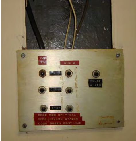
Figure 70. Fire alarm equipment
