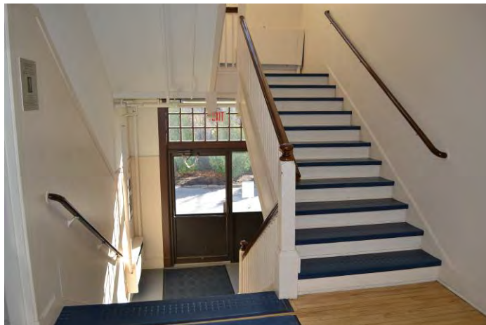
Non-continuous handrails that is not high enough to be a guardrail
