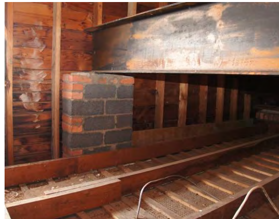
Figure 16. Steel beam in attic supported on brick and cinder block pier. This condition should be thoroughly reviewed in the next phase of work.
