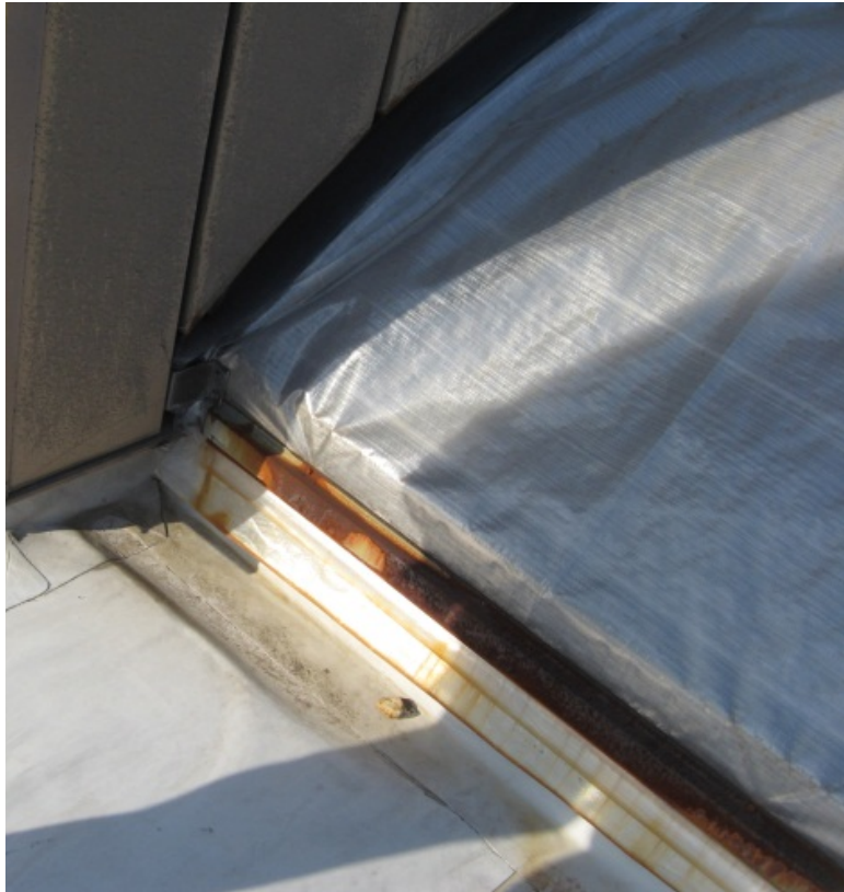
The roof continues to deteriorate.
