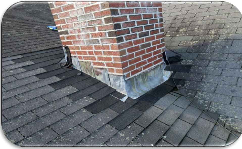
FIRE STATION 2 CHIMNEY, DETERIORATED FLASHING, PATCHED SHINGLES
