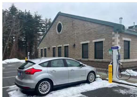
Electric vehicle charging station
