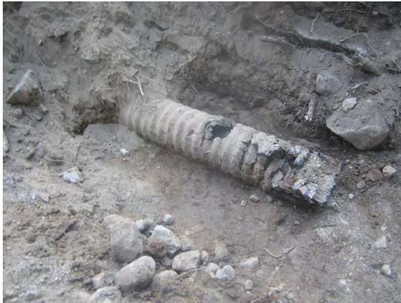
Example of a corroded metal pipe
