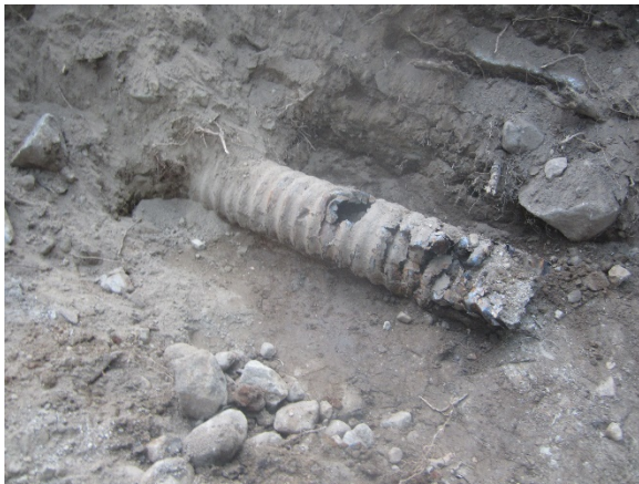
Example of corroded metal pipe.
