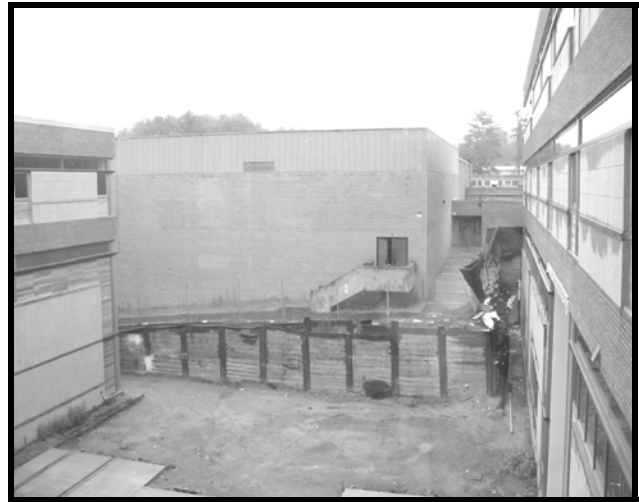
A view of the new and old LSRHS. (Photo Courtesy of Timothy Coyne)
