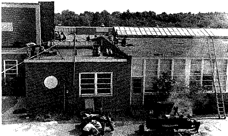
The roof at Peter Noyes School gets several thousand dollar's worth of first aid as workers pour on tar; gravel came later. (Town Crier photo)
