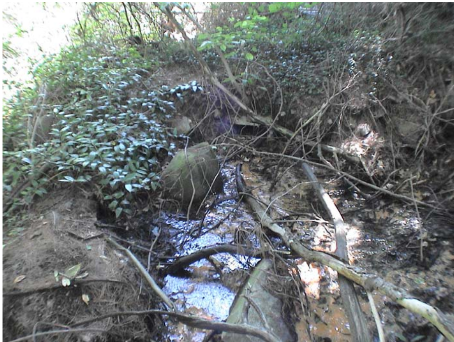
Figure 8: Seepage and Iron Algae Staining on Left Abutment
