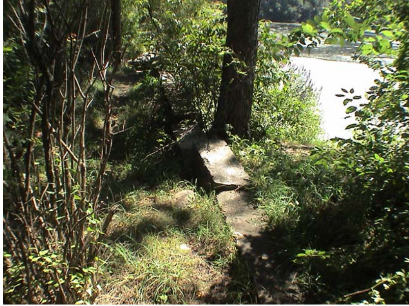
Figure 4: Displaced and Cracked Walls on Left Abutment (Note: trees and vegetation around walls)
