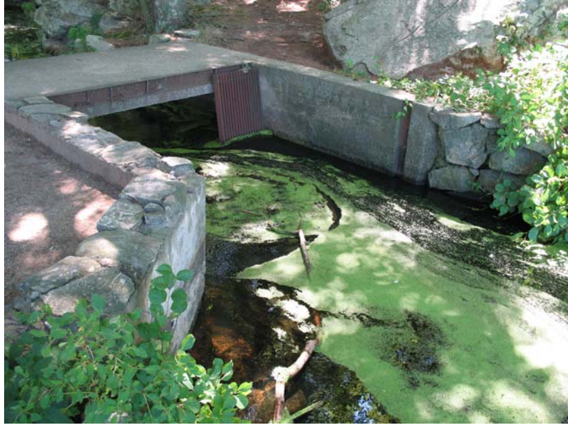
Figure 8: Sluiceway Intake and Trash Racks
