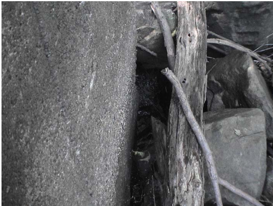
Figure 8: Seepage around Left Abutment at Hager Pond Dam
