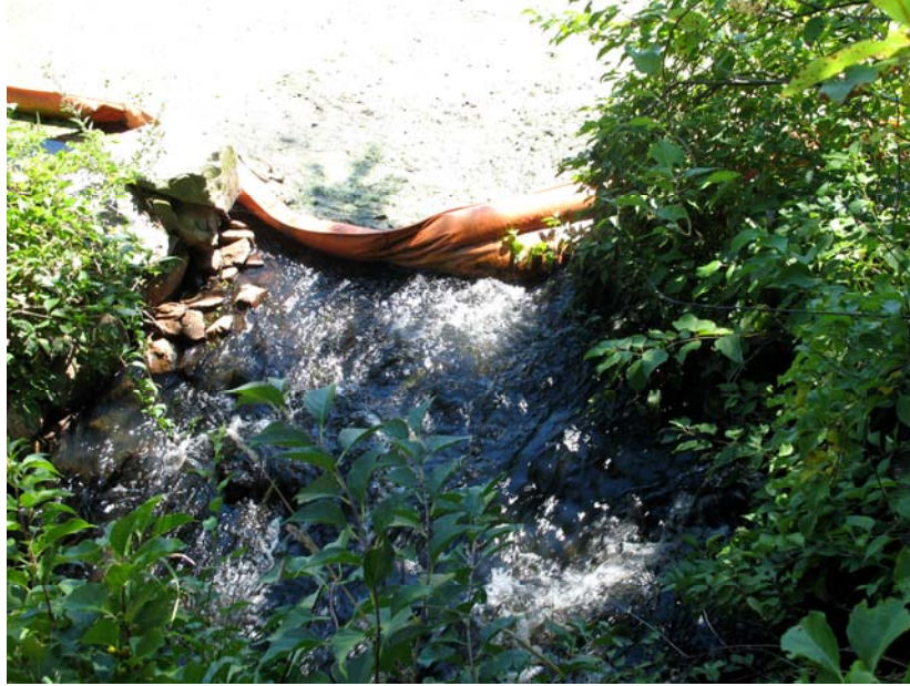
Figure 6: Inlet for Uncontrolled Spillway (Note: Erosion and vegetation around inlet)
