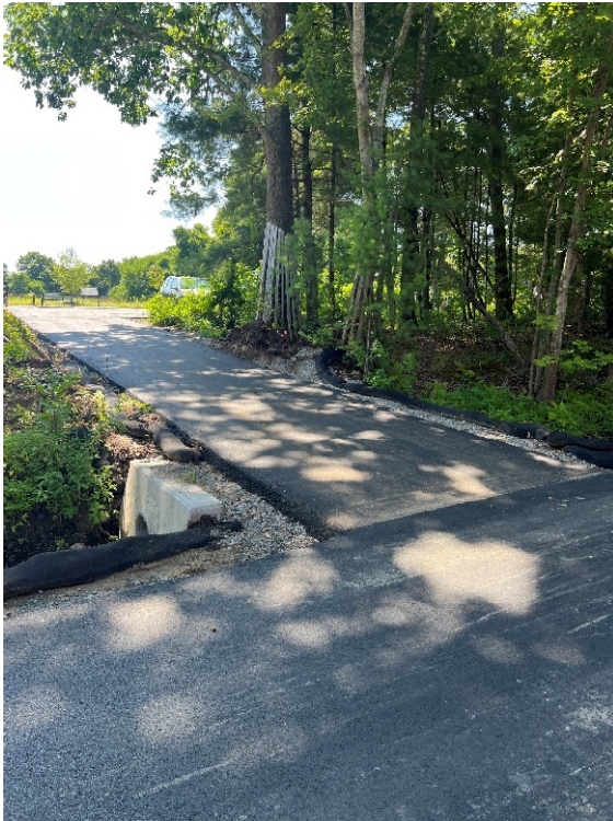
Photo 13: Looking at the paved spur path between the trail and the Morse Road parking lot.
