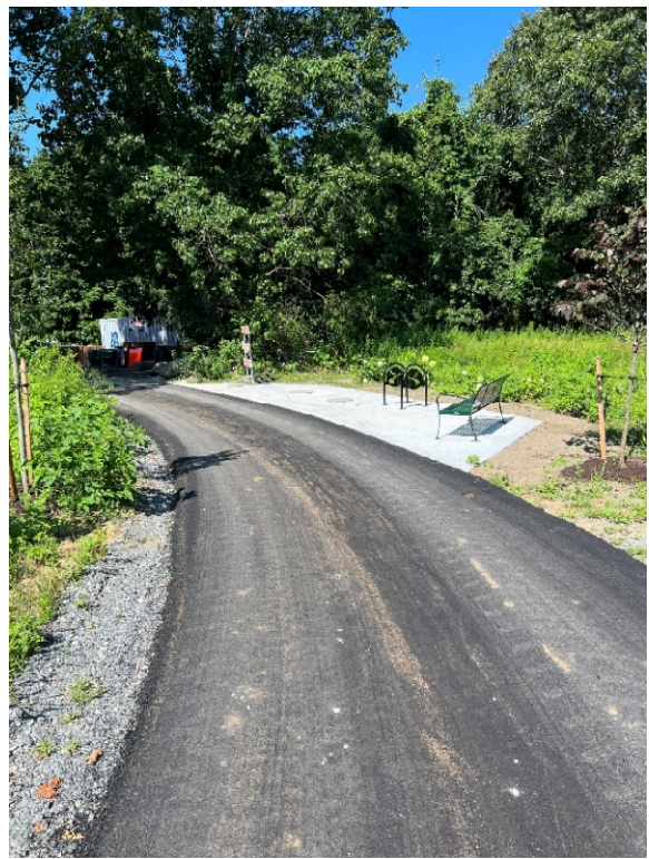
Photo 12: Sta. 1001+50 looking at the rest area along the Parkinson's Lot spur path.
