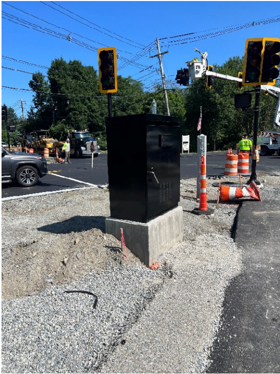
Photo 9: Looking at the newly installed traffic control cabinet south of Hudson Road.
