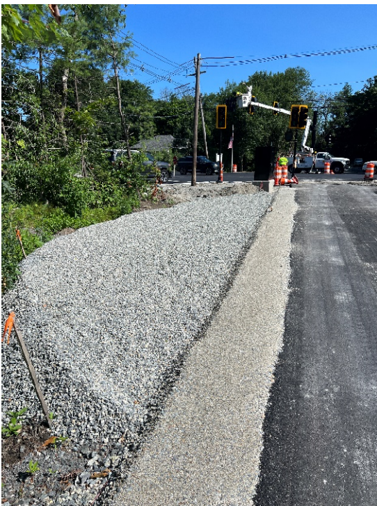
Photo 7: Sta. 174+00 looking at the gravel borrow subbase for the proposed rest area south of Hudson Road.
