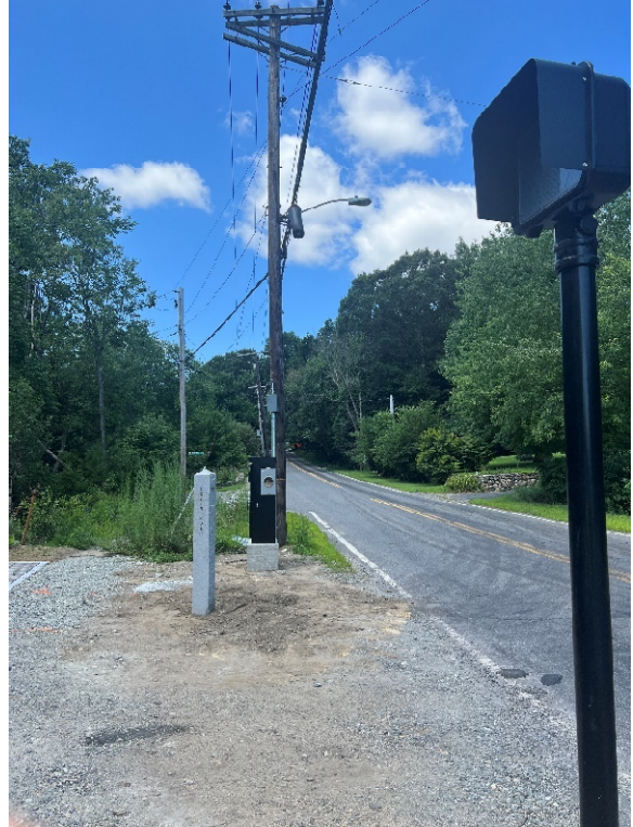
Photo 18: Sta. 307+50 looking at the pedestrian signal head and the traffic controller cabinet.
