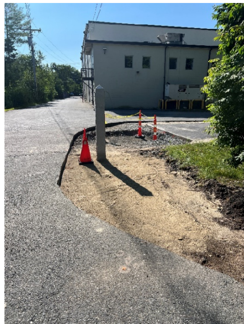
Photo 4: Sta. 108+50 looking at the sawcut pavement and sawcut trail in preparation for the pedestrian curb ramps and splitter island at the 71 Union Driveway.
