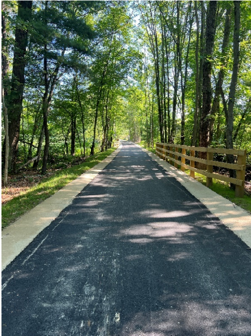
Photo 1: Sta. 103+00 looking at the paved surface course and the dense graded crushed stone shoulder.
