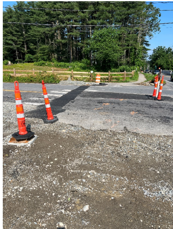
Photo 6: Looking at the trench where proposed conduit was installed to connect two pull boxes across Peakham Road.
