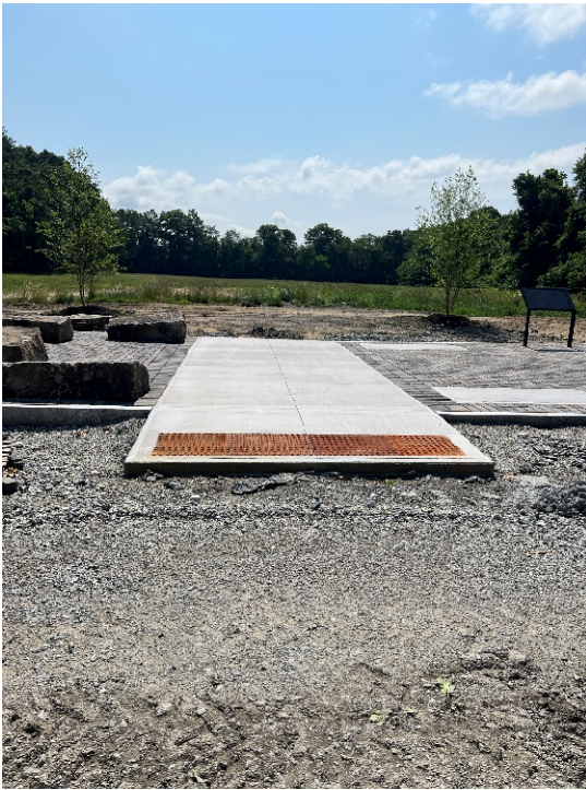
Photo 13: Looking at the pedestrian curb ramp and rest area in the Morse Road parking lot area.
