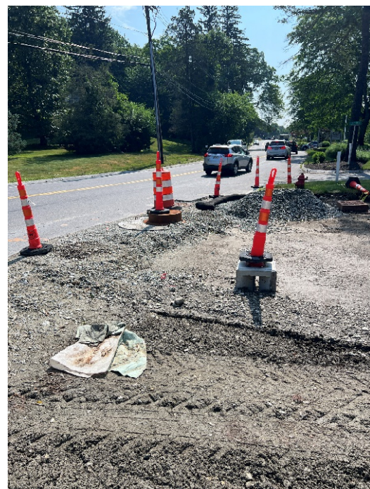
Photo 8: Looking at the concrete signal post foundation. All other foundations have been constructed but are not seen in this image.
