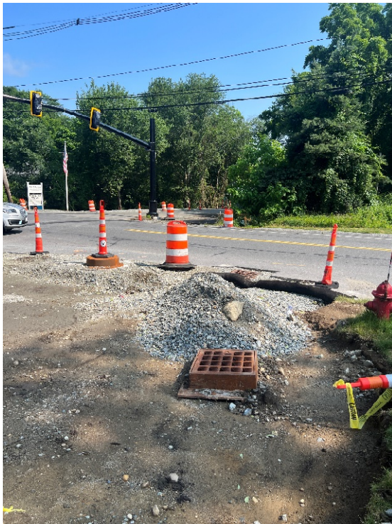
Photo 5: One staged catch basin, one staged manhole, and one catch basin that was installed in Hudson Road.
