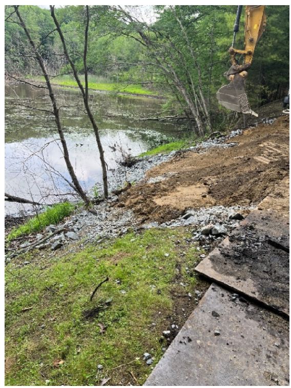
Photo 20: Sta. 332+00 looking at the new pipe and grading efforts north of Fairview Farms.
