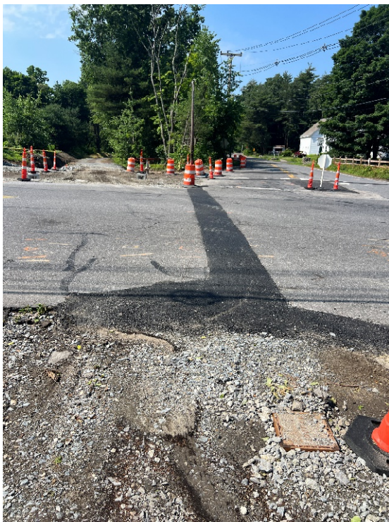
Photo 11: Looking at the pull box and conduit trench north of Hudson Road.
