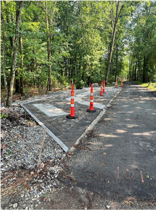
Photo 1: Sta. 101+00 looking at the rest area at the beginning of the project.
