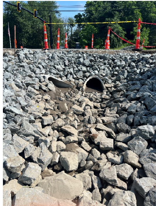
Photo 4: Sta. 174+50 looking at the two reinforced concrete pipes and flared ends south of Hudson Road.
