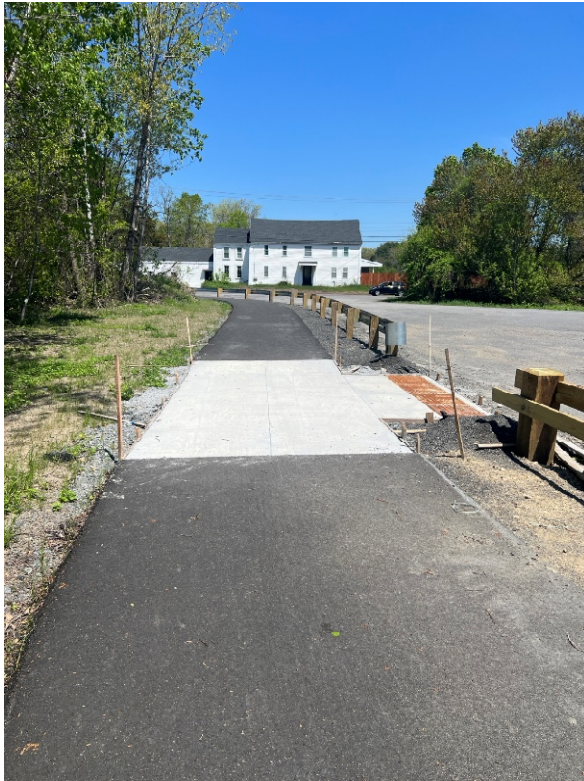
Photo 5: Sta 1106+50 looking at the constructed concrete work in the Davis Field parking lot.
