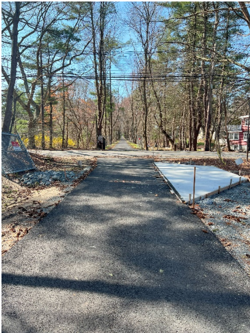
Photo 3: Sta. 144+00 looking south towards Old Lancaster Road and the proposed rest area.
