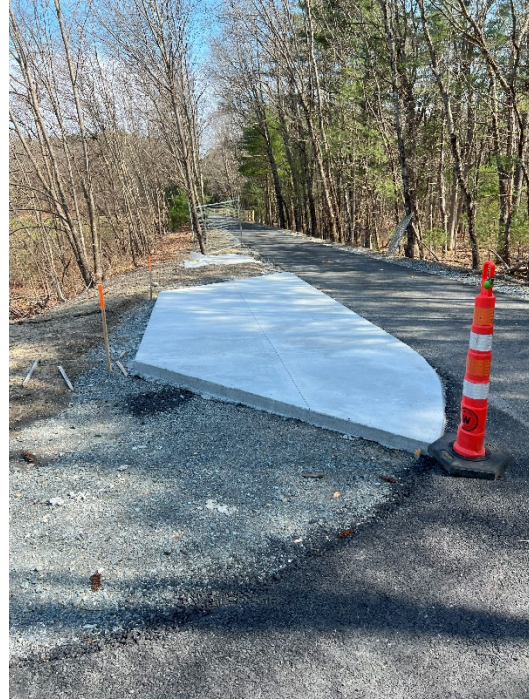
Photo 6: Sta. 184+50 looking north at the concrete rest area and the concrete pad for future art installation.
