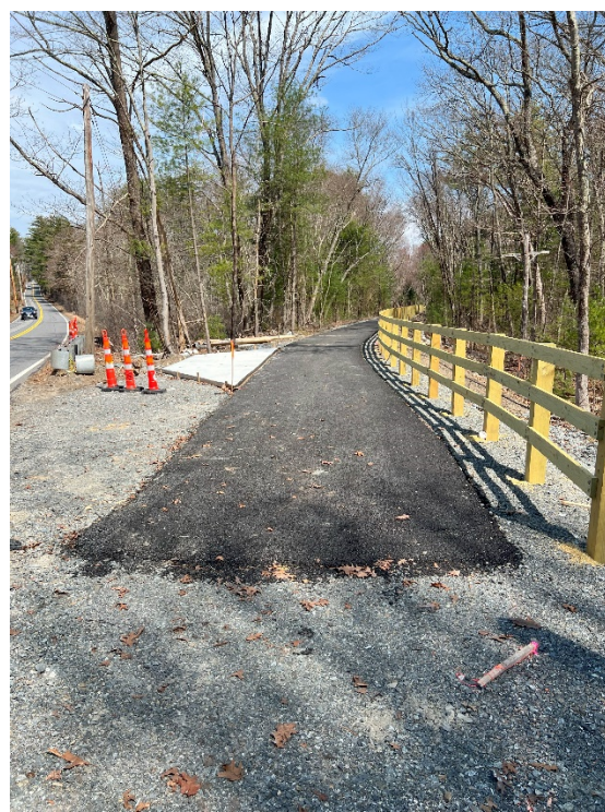
Photo 12: Sta. 284+50 looking at the fencing and concrete rest area north of Pantry Road
