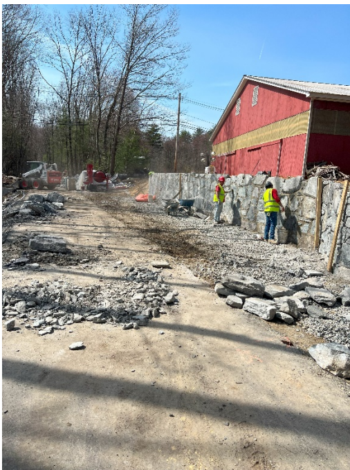
Photo 7: Sta. 217+50 looking south at the retaining wall construction for the Morse Rd rest area.
