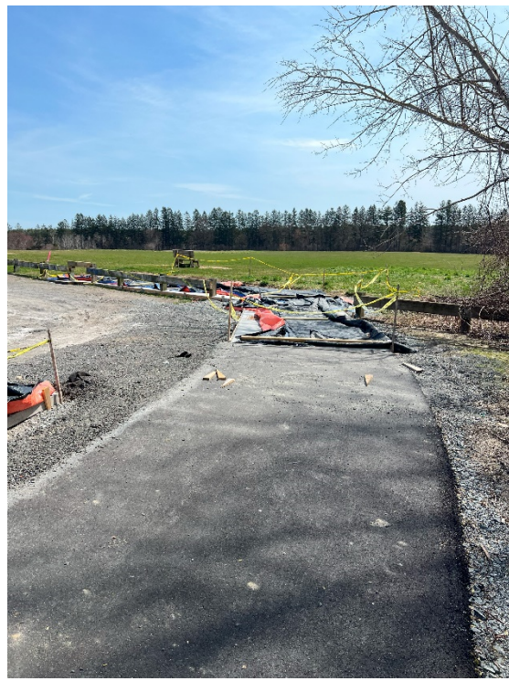
Photo 14: Sta. 1107+00 looking at the rest area at the end of the Davis Field spur path.
