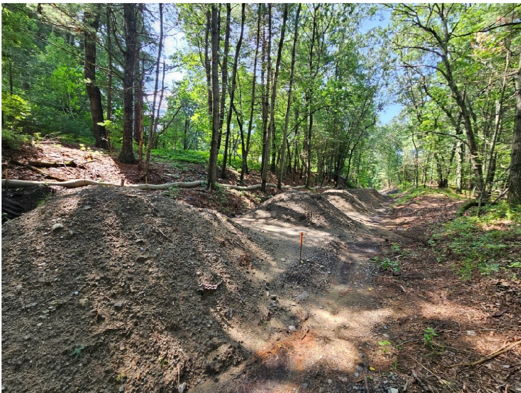
Photo 2: Excavated material located on BFRT, north of Old Lancaster Road looking south.
