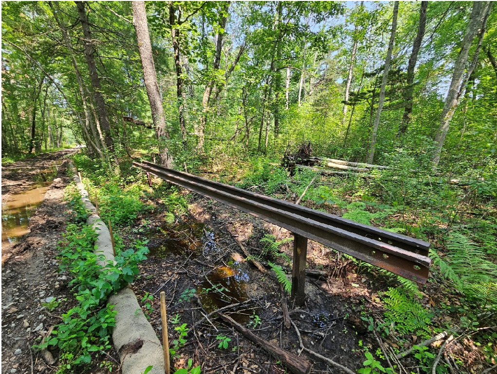
Photo 14: Two segments of existing rail placed on existing rail rests. Approx Sta. 303+15 RT
