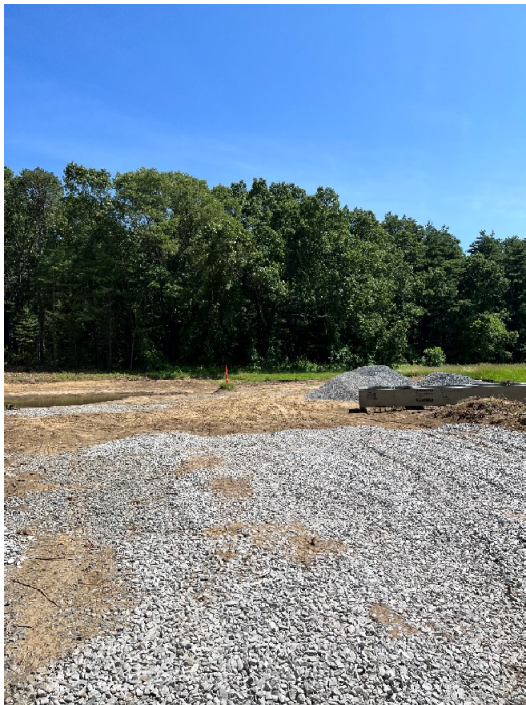
Photo 7: Sta. 215+60 looking north towards the proposed parking lot, standing at Morse Road
