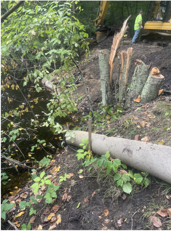
Photo 9. STA 332+00 looking North in between wetland pond area and western limit of proposed trail. Approximate location of the inlet for hydraulic connection.
