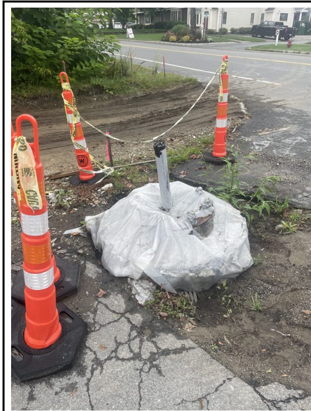
Photo 3: STA 175+50. Signal foundation installed at Ti Sales Driveway is coned off and covered to protect from vehicle damage.
