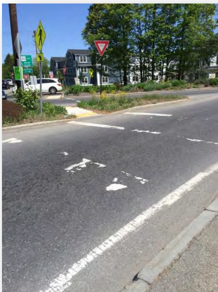
Faded pavement markings along eastbound channelized right turn lane.
