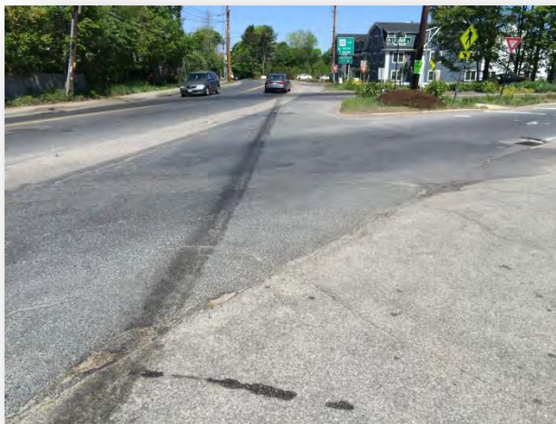
Poor pavement conditions along Boston Post Road.
