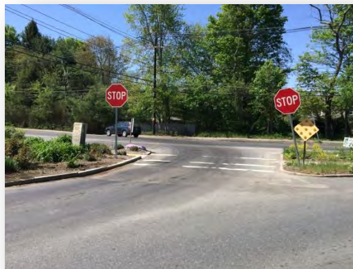
STOP sign on the right has been hit and it tilting into the roadway.
