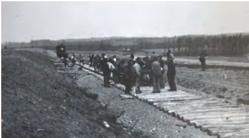
Laying rails on a railbed along the Central Mass. line in 1903. Note cutting of the original ground surface for the rail bed (Boston & Maine Hist. Society, 2008).
