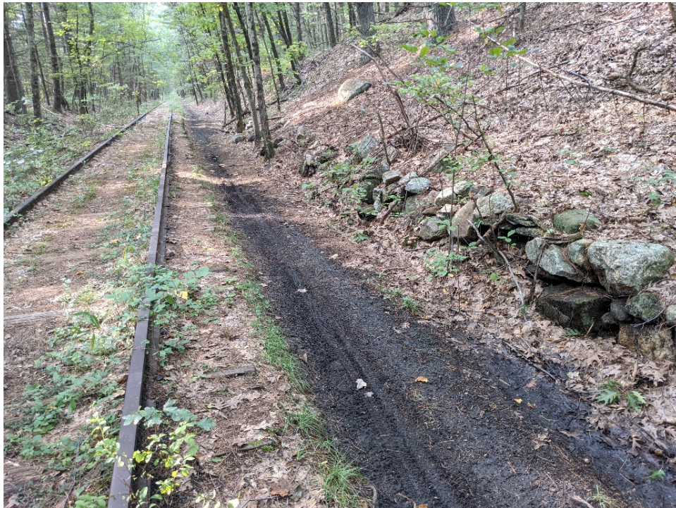
Photo # 21 Stone retaining wall at MP 23.95 along the north side of the rail corridor, view west
