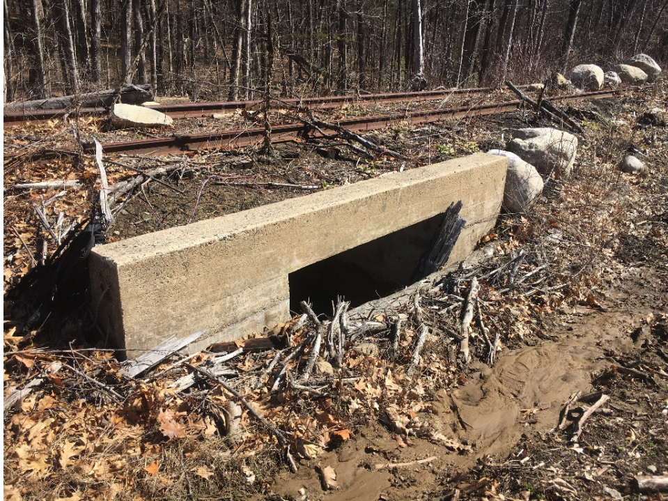
Photo # 16 Cattle pass at MP 25.83, south side, notice mud and debris dam that has formed, covering most of the opening, view north
