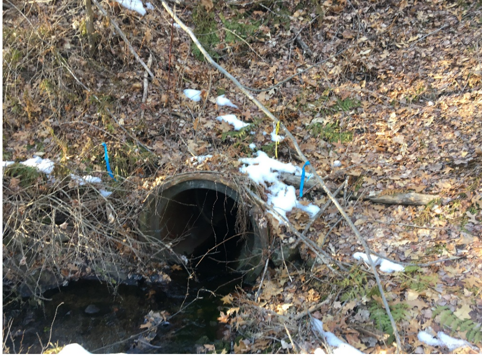
Photo # 14 Culvert 132A at MP 26.12, north end with collapsed headwall, view north
