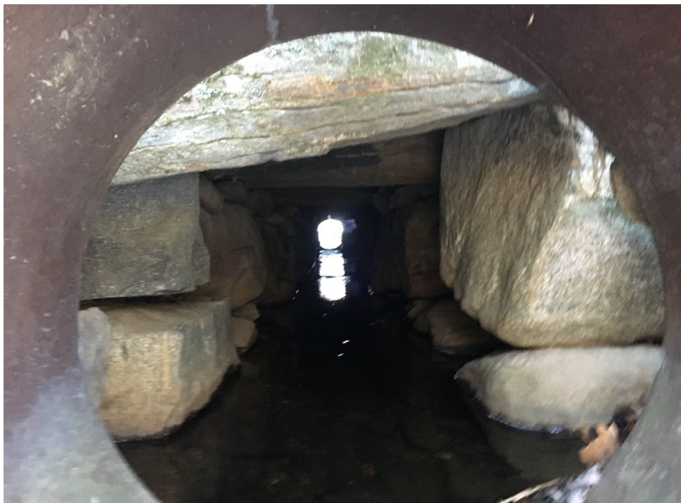
Photo # 15 Culvert 132A at MP 26.12, stone box in center of culvert, view south
