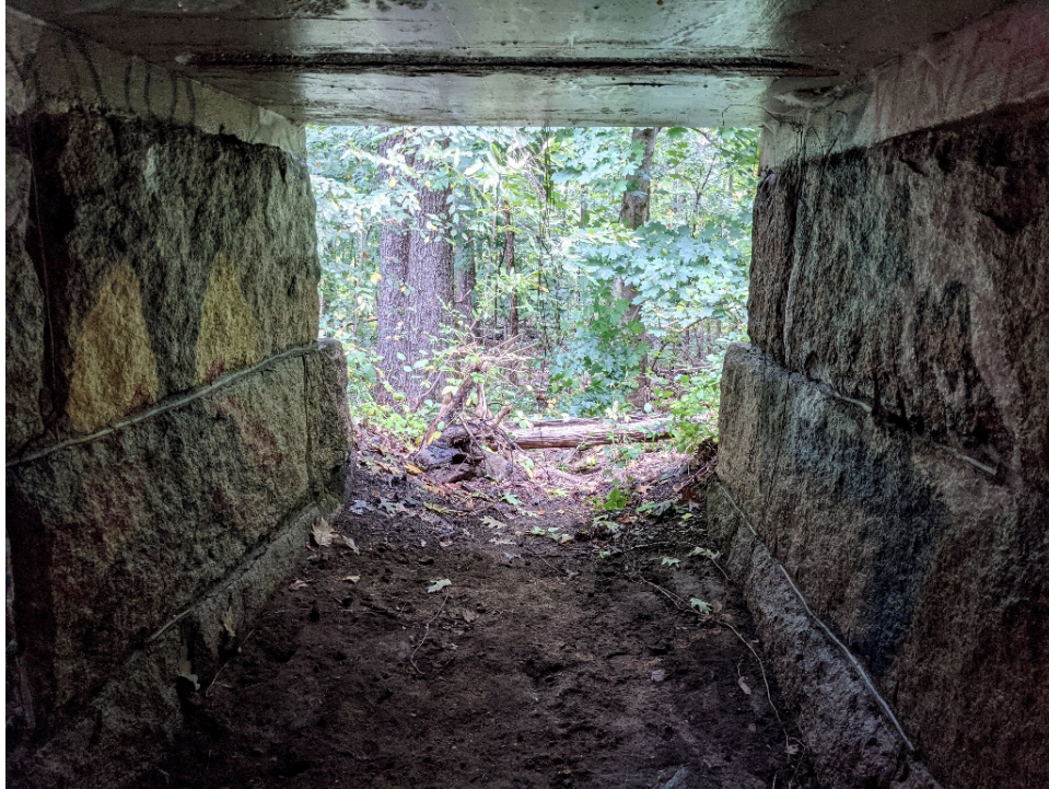
Photo # 18 Cattle Pass at MP 25.83, view of the interior of the cattle pass toward the north side opening, view north
