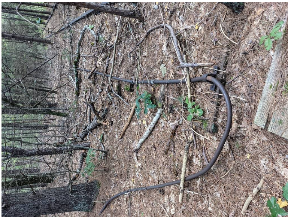
Photo # 25 Conduit for pipe-connected derail switch at MP 23.33, view east
