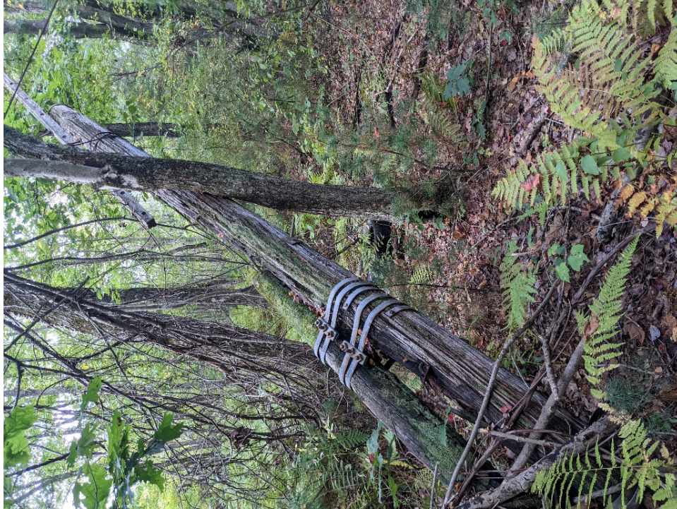
Photo # 44 Telegraph Pole at MP 23.06, view S
