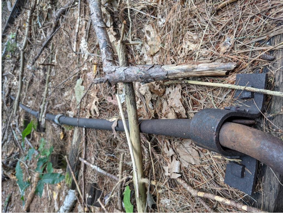
Photo # 24 Conduit for pipe-connected derail switch at MP 23.33, view east
