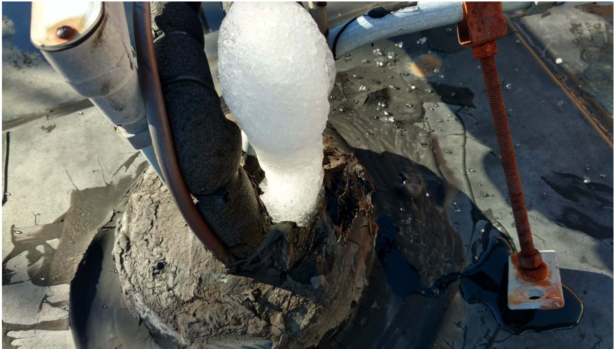
Haynes Kitchen Equipment Refrigeration Line Leaks
