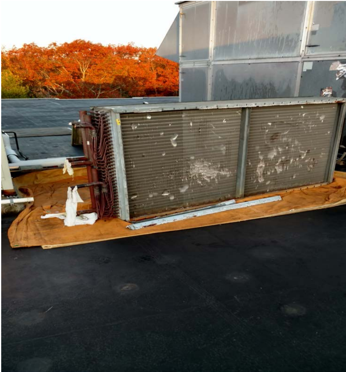
Existing Curtis Rooftop HVAC Unit
