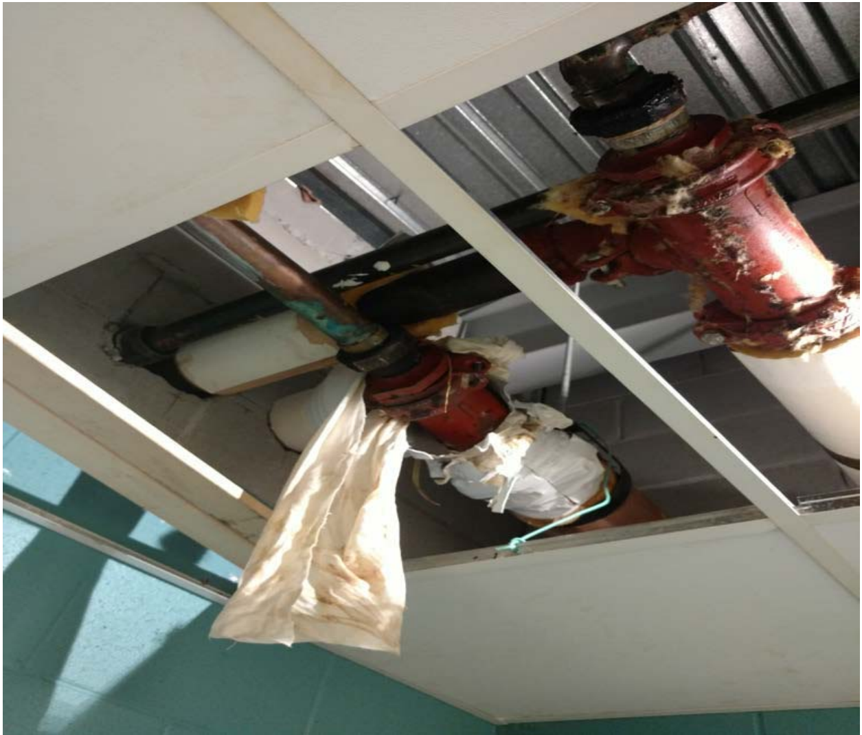
Curtis Heating and Valves
