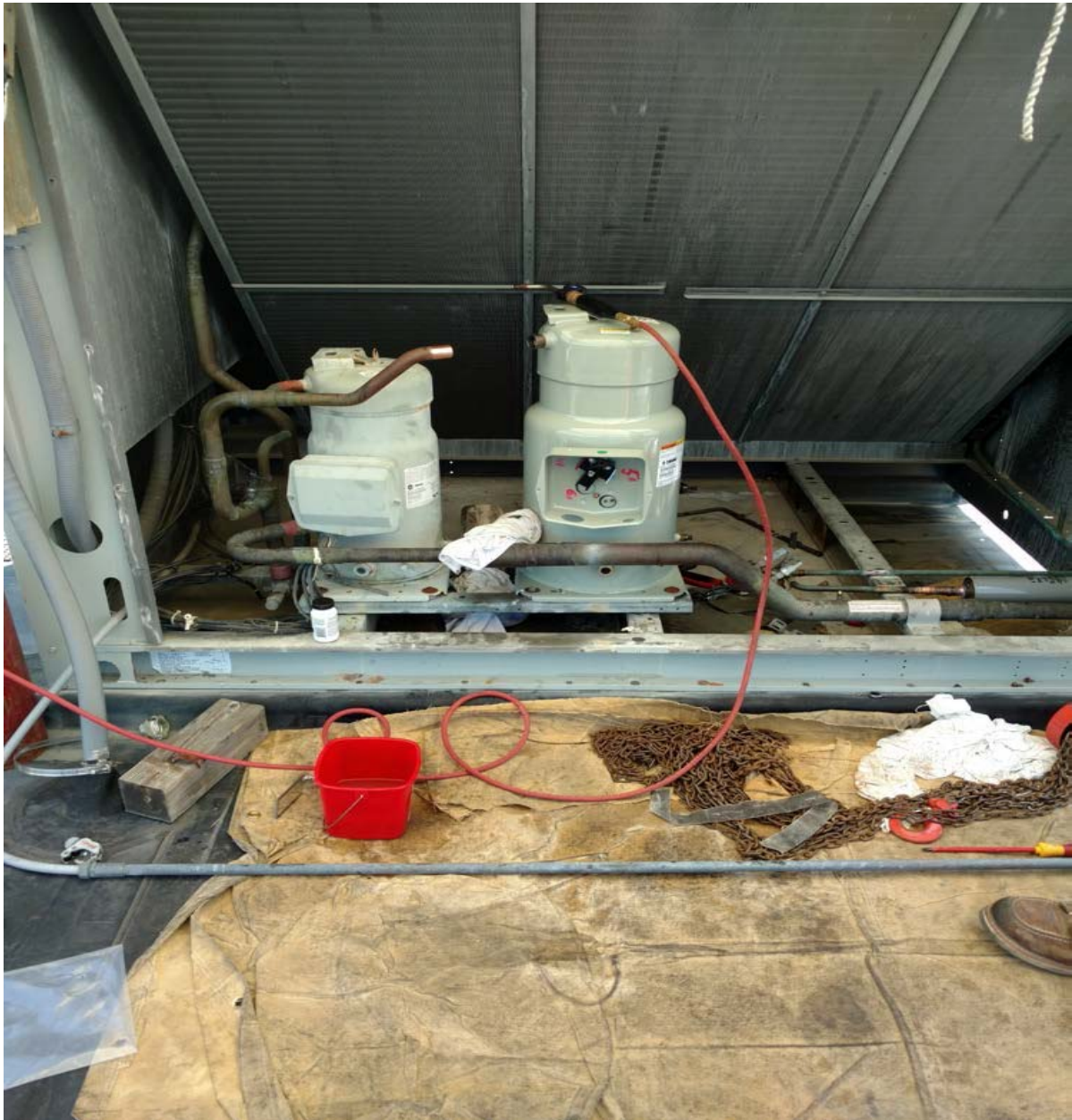
Existing Curtis Rooftop HVAC Unit Interior
