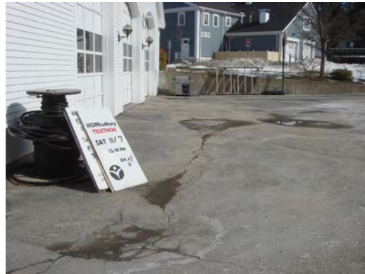
Asphalt driveways are failing
