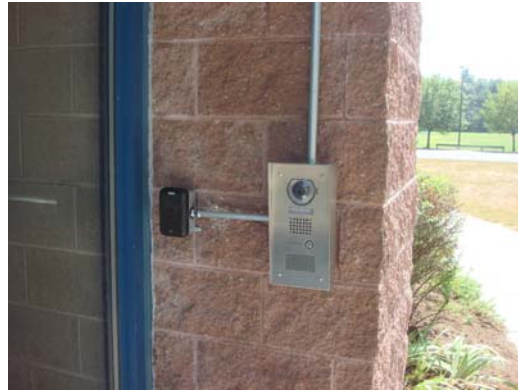
New card access controls for doors
