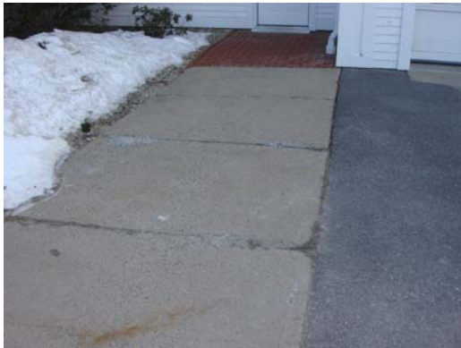
Sidewalks need replacement
