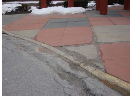
Concrete is deteriorating
