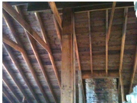
saw cut rafters visible in the attic attest to the gable roof being much newer (19th century) than the still visible posts and dragon trusses of the earlier (18th century) hip roof of the Parsonage.
