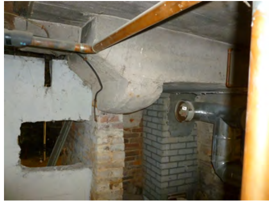
Copper piping from the existing boiler and the vent from the boiler to a modern brick connection to the historic chimney are visible in this view.
