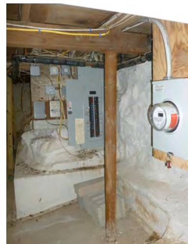
The electrical meter box and the main breaker box bracket one of the historic beams shored by a steel column with a corroded base.
