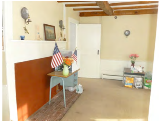
Exposed framing in the southeast office. The fireplace has been closed in.
