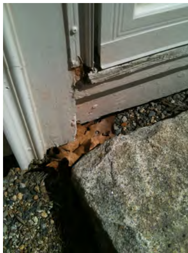
Water damage at sill and door framing.
