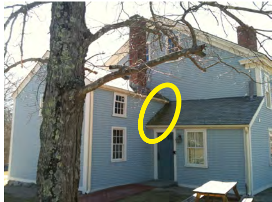
Water staining at the shed roof intersection with the east ell.
