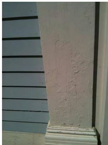
Moderate paint failure at pilaster at main entry.
