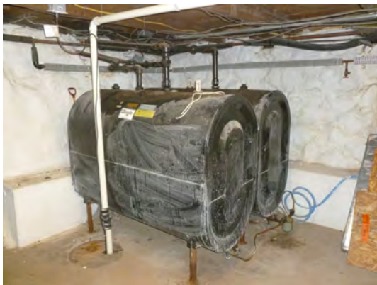
New oil tanks.
