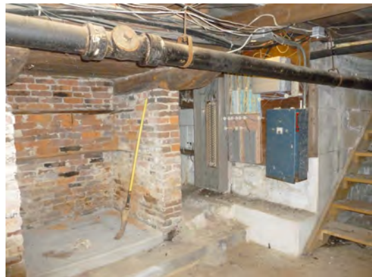
In this view the opposite side of the historic chimney breast from the photo above is visible along with largely redundant telephone switch gear, the waste line from the kitchen and areaway steps.
