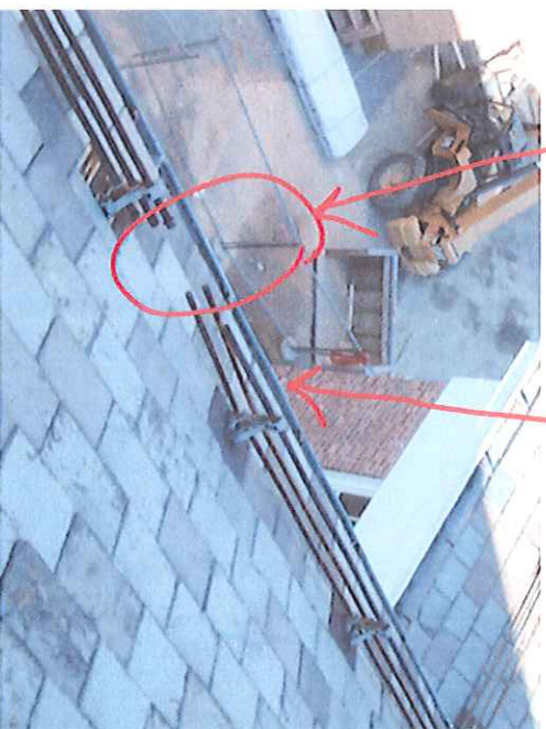
LEFT SIDE SNOW RAIL, SEPERATION & DAMMAGED PIPE
