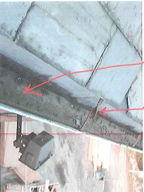
VIEW OF LEFT REAR GUTTER; [COPPER] LINED W/TAR, RUSTED STEEL HANGER
