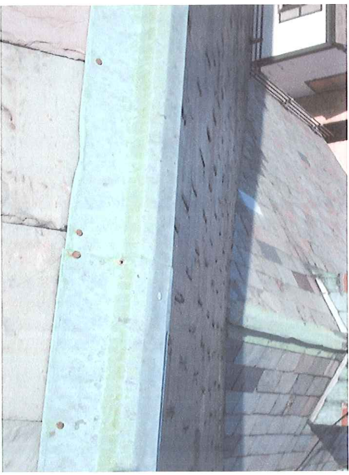
VIEW OF COPPER RIDGE VENT W/COMMON ROOFING NAILS
