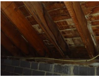
No attic insulation
