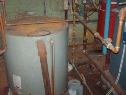
Condensate return tank and uninsulated steam piping
