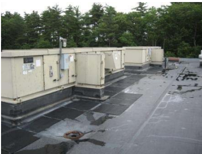
Gym rooftop air-handling units
