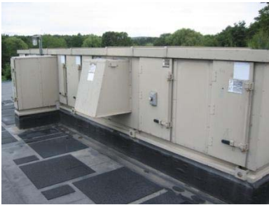
Cafeteria Rooftop Unit
