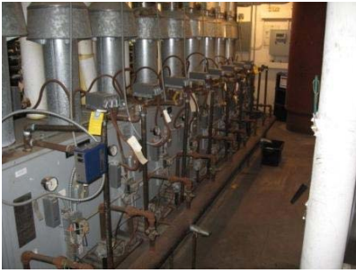
Existing Hydrotherm Boilers
