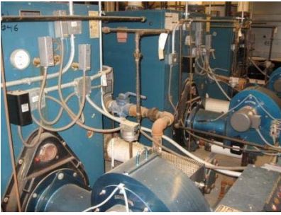
Existing Burnham Boilers
