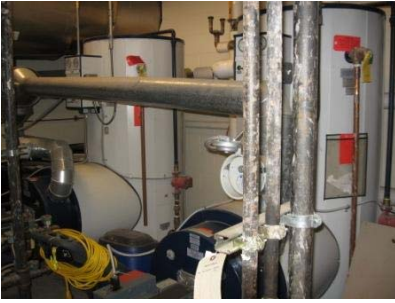
Domestic Water Heaters
