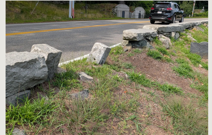
Road edge — displaced wall stone scattered down the bank
