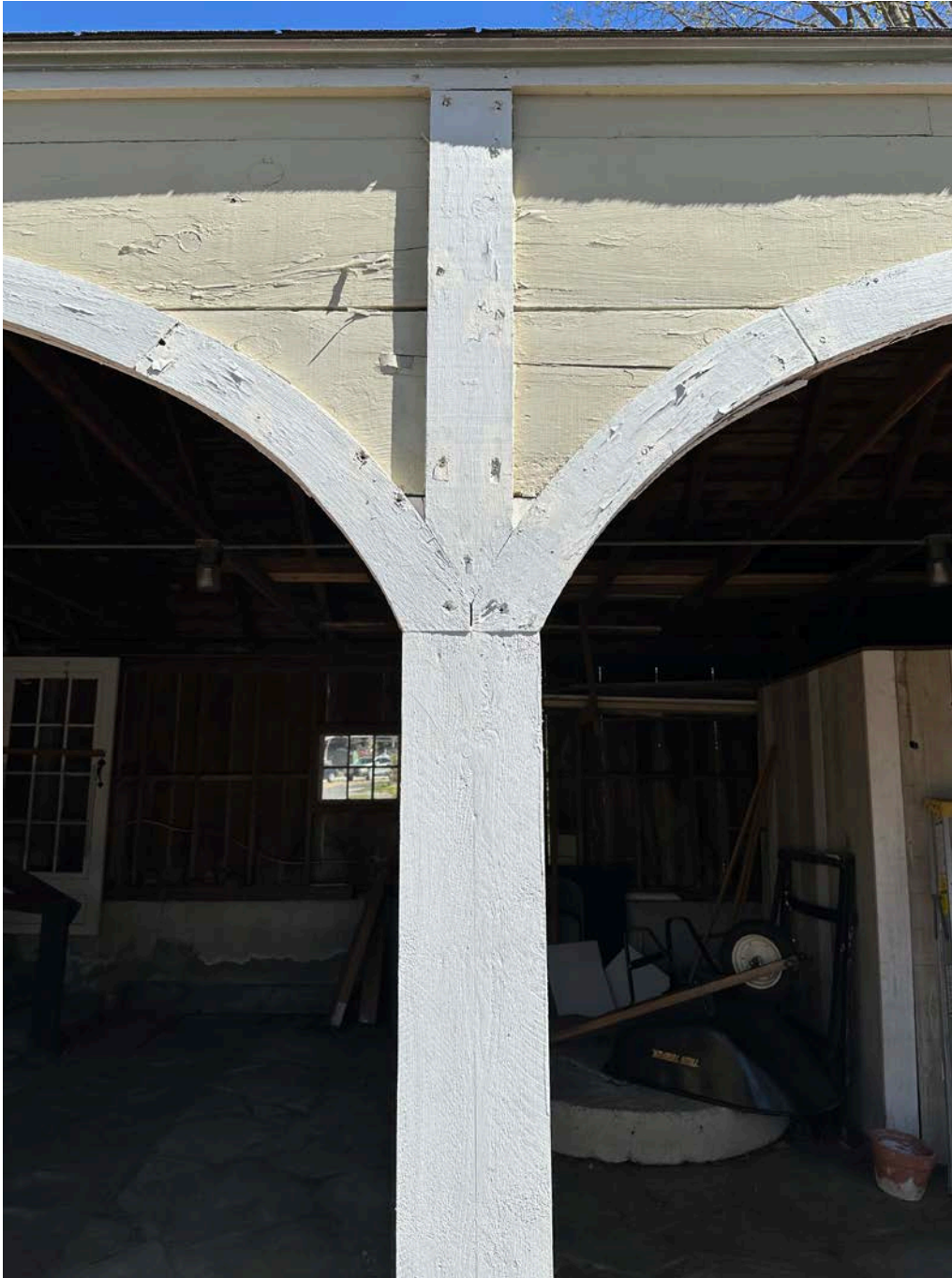
Figure 4.1-8 Peeling paint at carriage house columns and arches.
