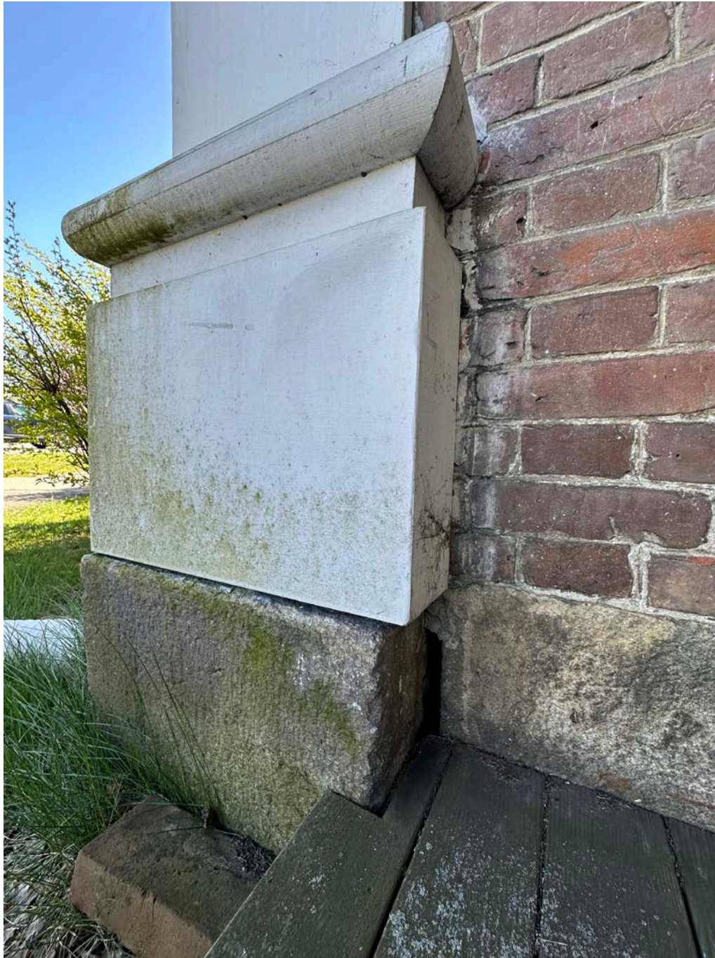
Figure 4.3-4 There is no evident base flashing between the wood pilaster and the granite foundation.
