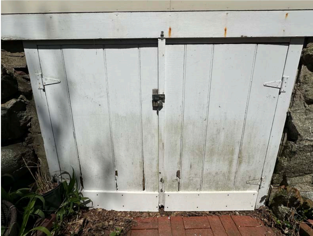
Figure 4.1-12 Fasteners used to secure the trim, corner boards and water tables have begun to corrode and stain the wood.
