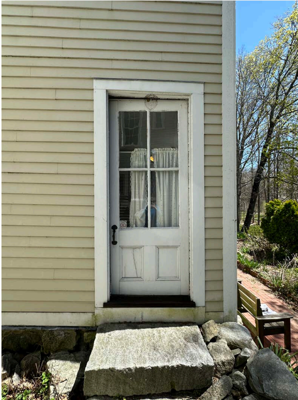
Figure 4.4-8 D-12 in poor-to-fair condition, showing signs of wood deterioration, cracks, and previous repairs.
