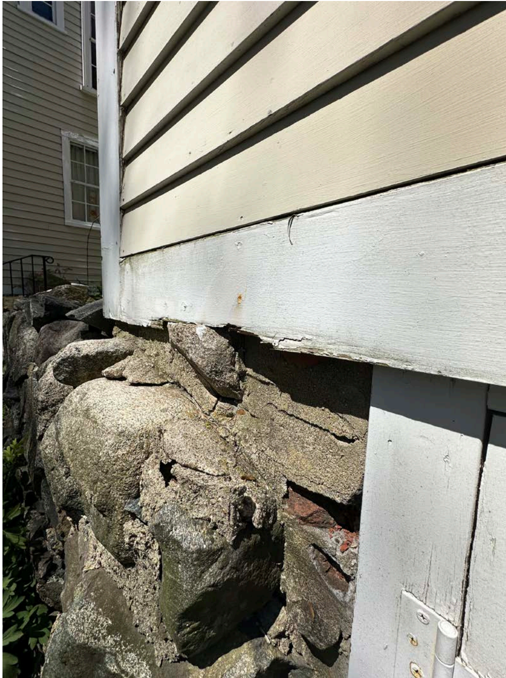
Figure 4.3-6 There is no evident base flashing between the cladding system and the ashlar stone foundation wall.
