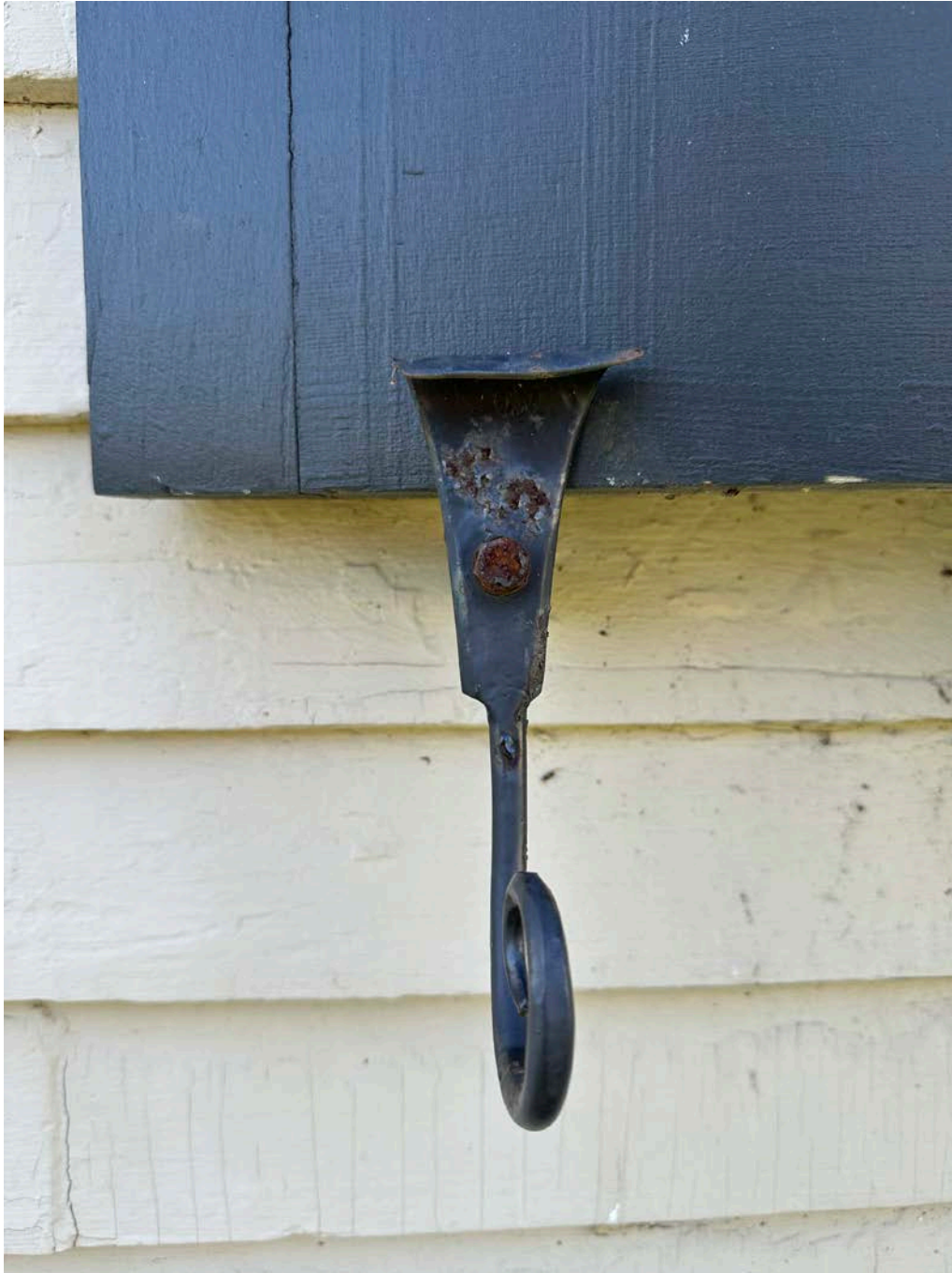
Figure 4.6-5 Less typical conditions found were that the shutters have been loosely anchored to the building, and many of the tiebacks are loosely installed and are rusting. Typical condition seen throughout.
