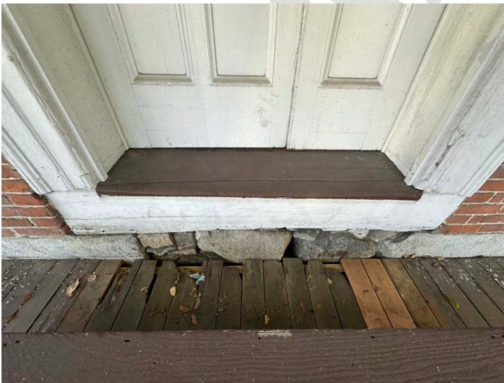
Figure 4.10-3 The decking planks directly below the door threshold are rotted, and are exhibit the most severe deteriorated of the deck.
