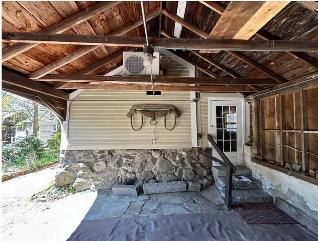
Figure 4.3-7 Ashlar foundation wall shared by the east wall of the southeast addition, and the carriage house.
