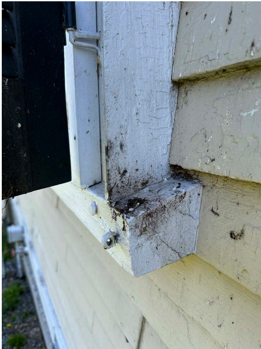
Figure 4.6-4 Evidence of soiling such as dust, dirt and debris piling up. Typical condition seen throughout.
