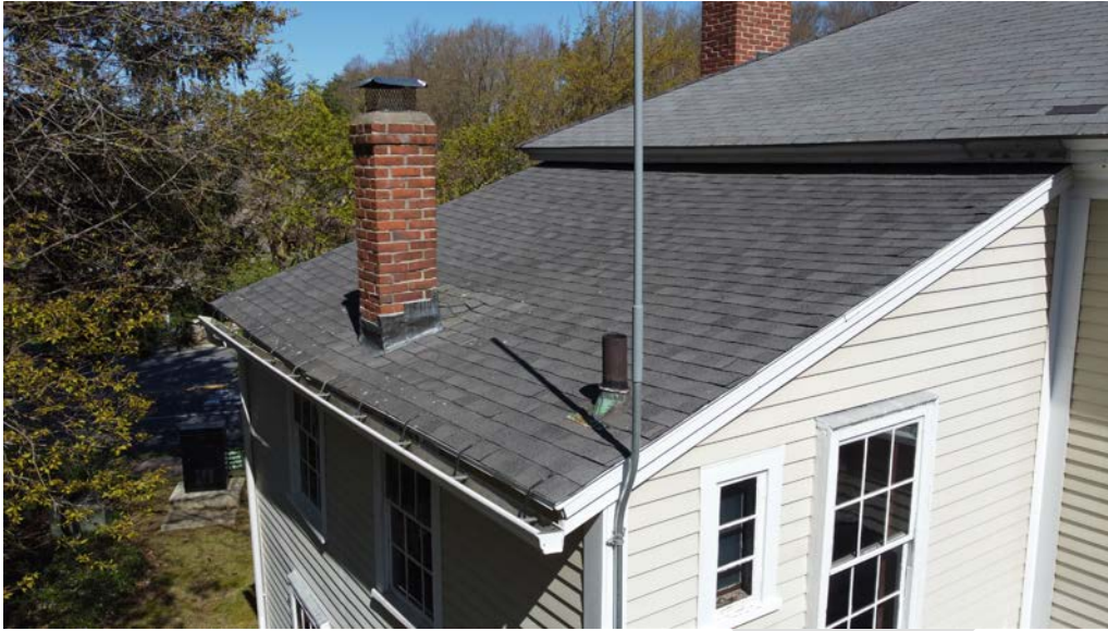
Figure 4.8-6 Along the southwest extension, Wood blocking was cut to match the profile of the fascia and was installed on this elevation, however, only one of the three blocks are actually fastened to the body of the gutter.
