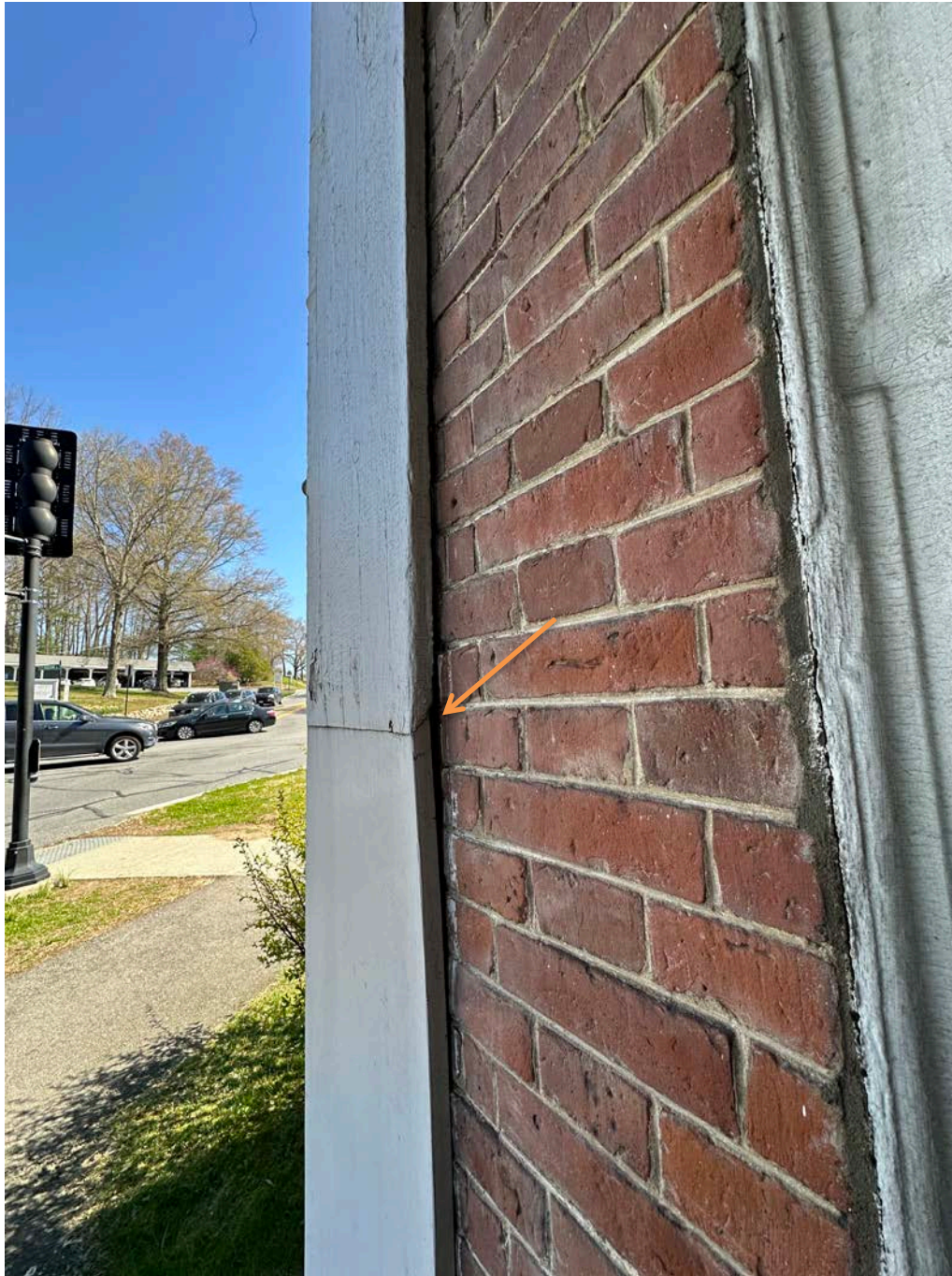
Figure 4.1-15 The pilasters are separating from the brick walls causing gaps between the materials.
