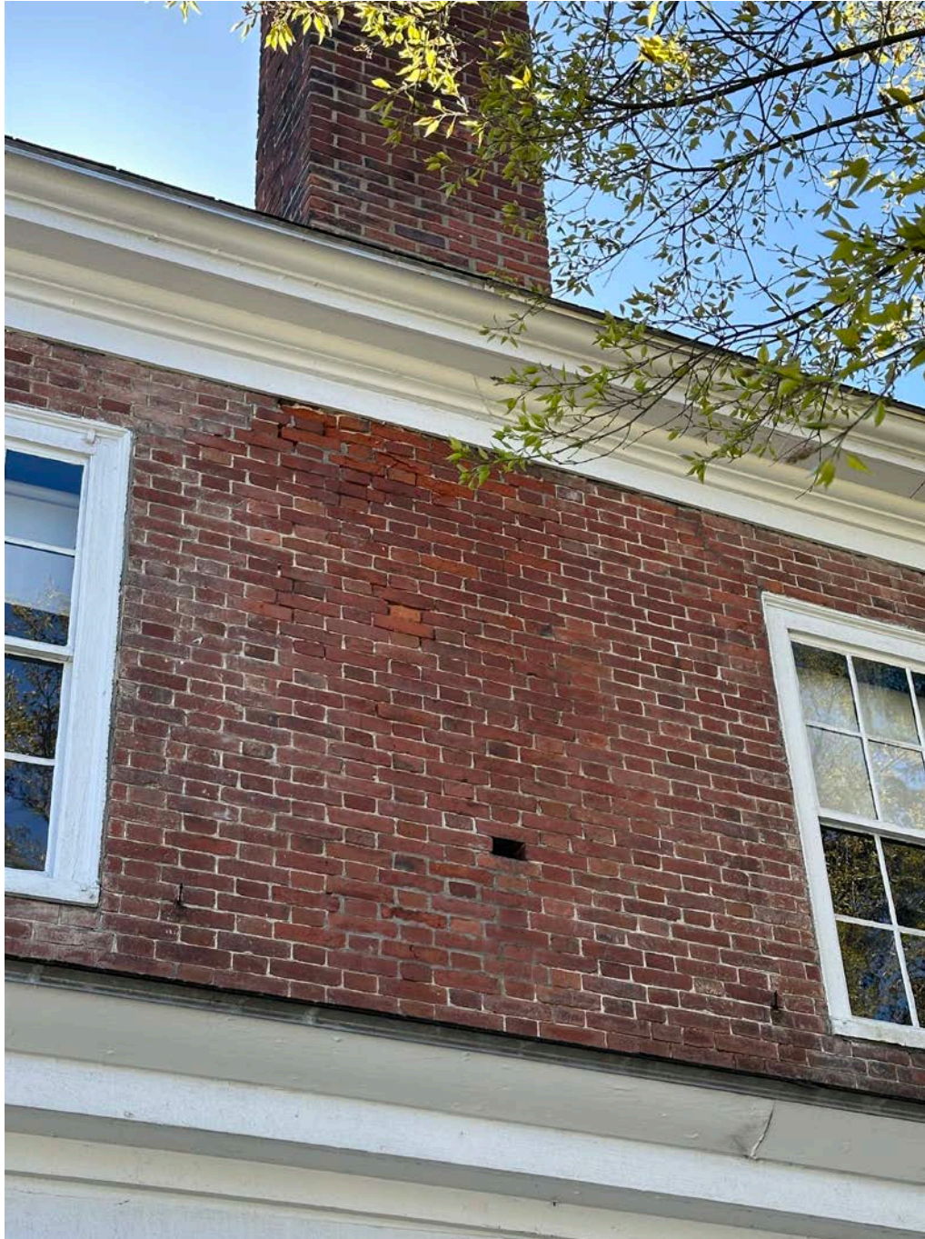
Figure 4.2-7 There are two areas on the west elevation of approximately 3' by 5' between windows W-46 and W-47, which show signs of deterioration. Bricks are missing their fire faces or cracked, and there is extensive mortar loss.
