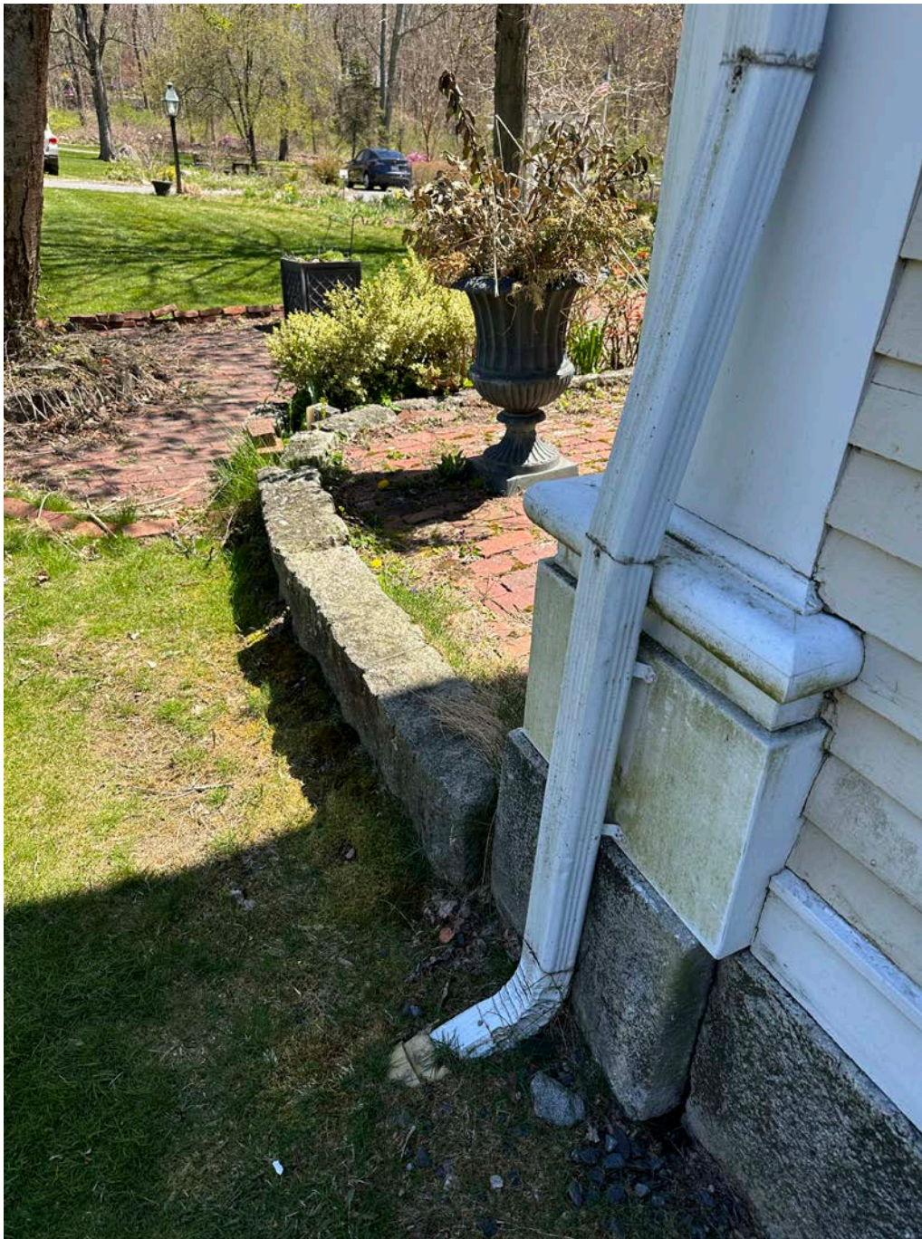
Figure 4.8-1 Located at the northeast corner of the house is a downspout that expels water below grade.
