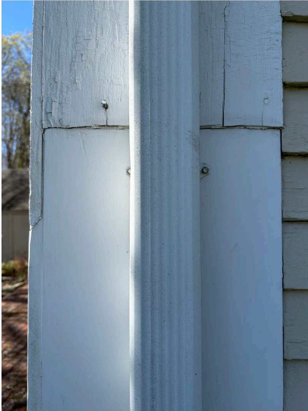
Figure 4.8-5 Downspouts fastened directly to the wooden pilasters with downspout straps installed without spacers at the northwest and northeast corners
