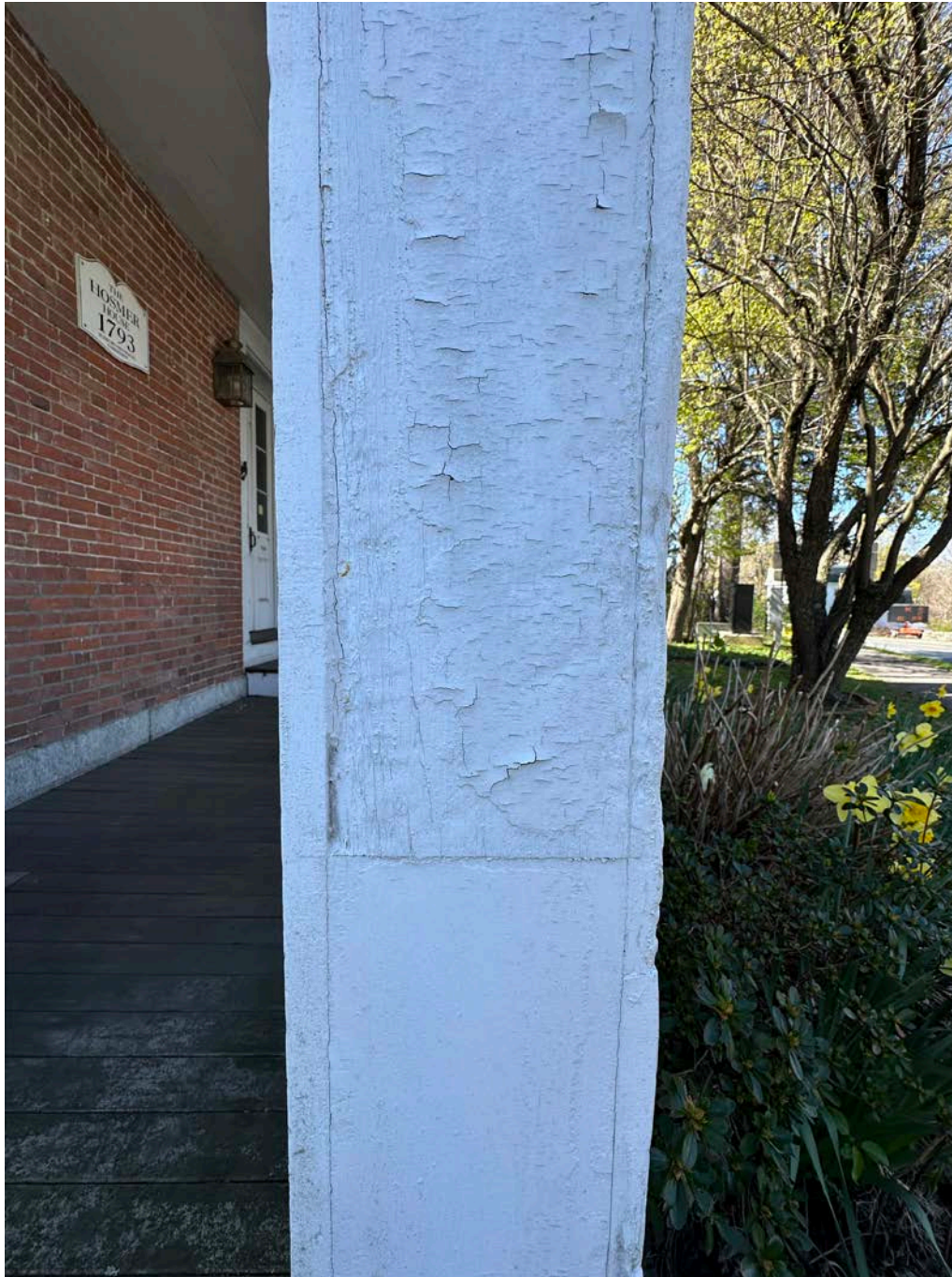
Figure 4.10-5 Between 12" to 14" of the shafts of the two columns at either end of the porch have been replaced along with all 4 column capitals and bases.
