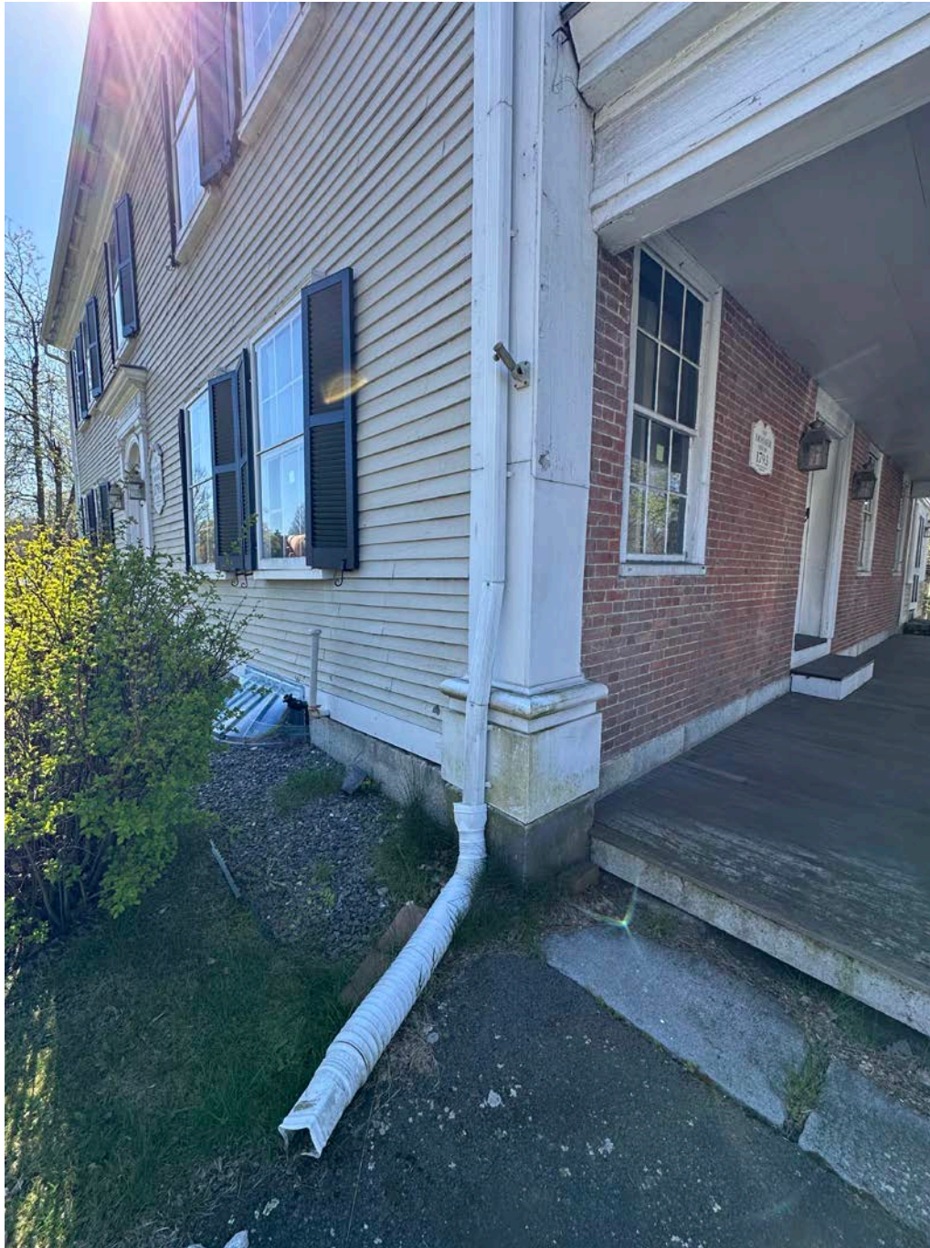
Figure 4.8-2 Located at the northwest corner of the house is a downspout that expels water through a downspout extension above grade, away from the house's foundation walls.
