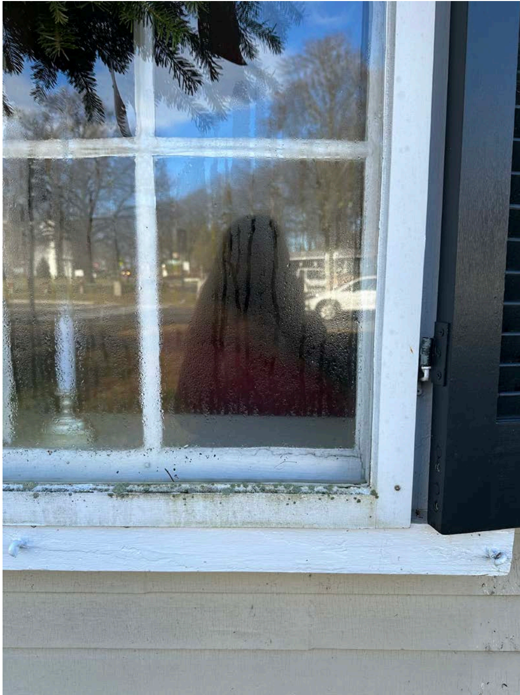
Figure 4.4-12 During the Request for Proposal process in December 2023, condensation was observed between the window and storm window.
