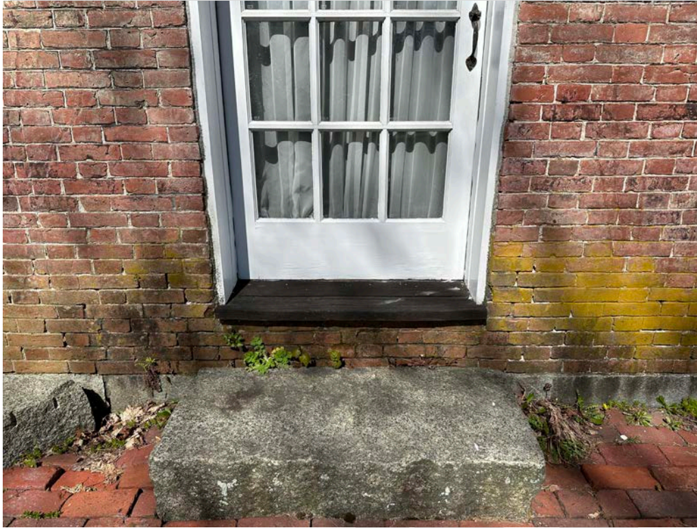
Figure 4.4-9 Door and sill on D-12 and D-06 were found to be damaged, cupped, and pitched backward.
