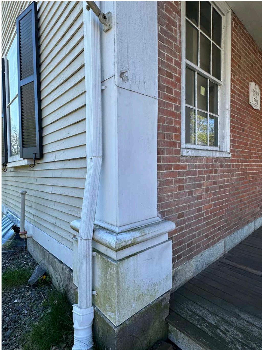
Figure 4.1-13 Bottom 3 feet of each pilaster shaft and both bases have been replaced.
