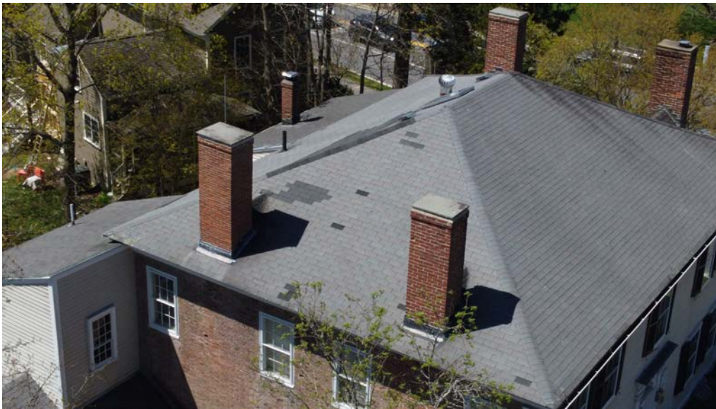
Figure 4.9-1 Four tall, brick-masonry chimneys are situated in pairs along the east and west elevations of the main house, slightly set back from the hipped roofline. The fifth chimney is located in the southwest addition.
