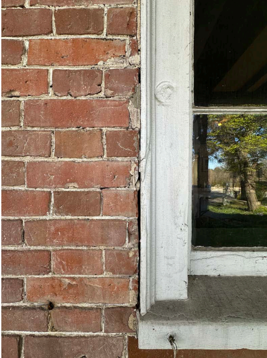
Figure 4.2-6 Several of the bricks at the outer edge of the masonry openings are damaged, missing pieces, and patched with mortar.
