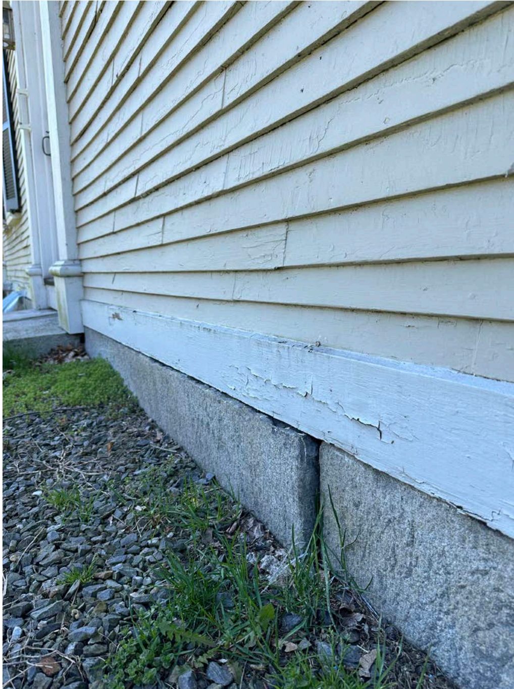
Figure 4.1-11 Splits in the wood ranging from 1 linear foot to 2 linear feet.
