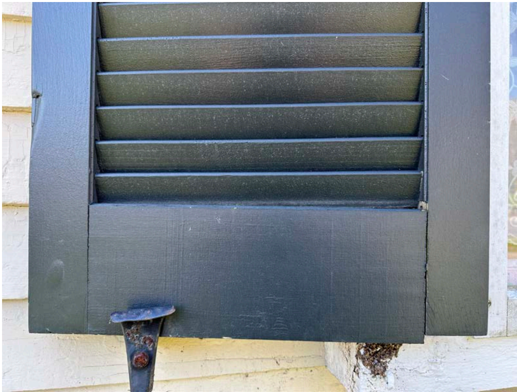
Figure 4.6-1 Loose bottom rail of a shutter. Typical conditions seen throughout.
