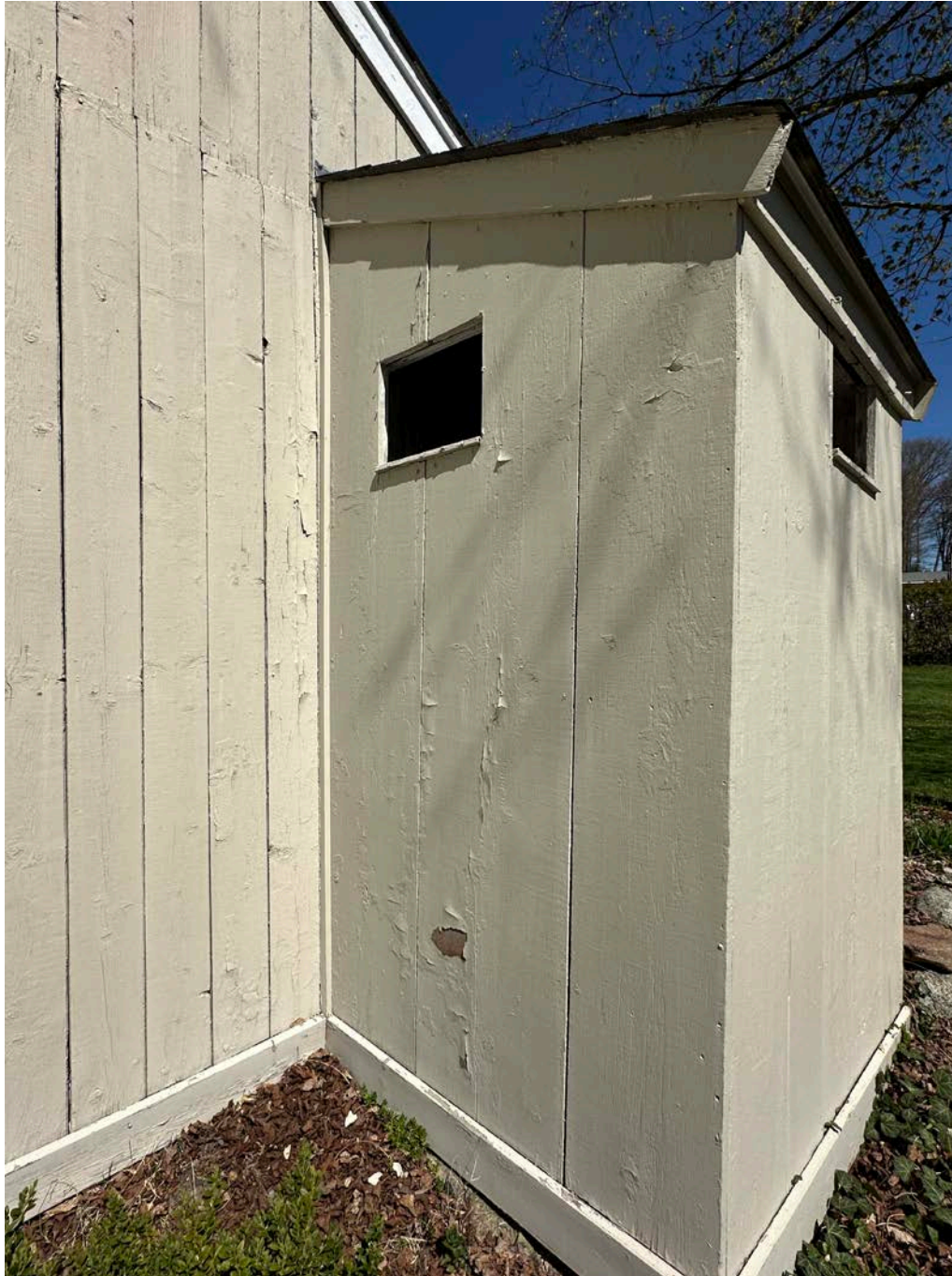
Figure 4.1-10 Vertical planks at outhouse with an average exposure of 15 inches. Visible gaps varying approximately 1 inch to 2 inches in width, and peeling paint.
