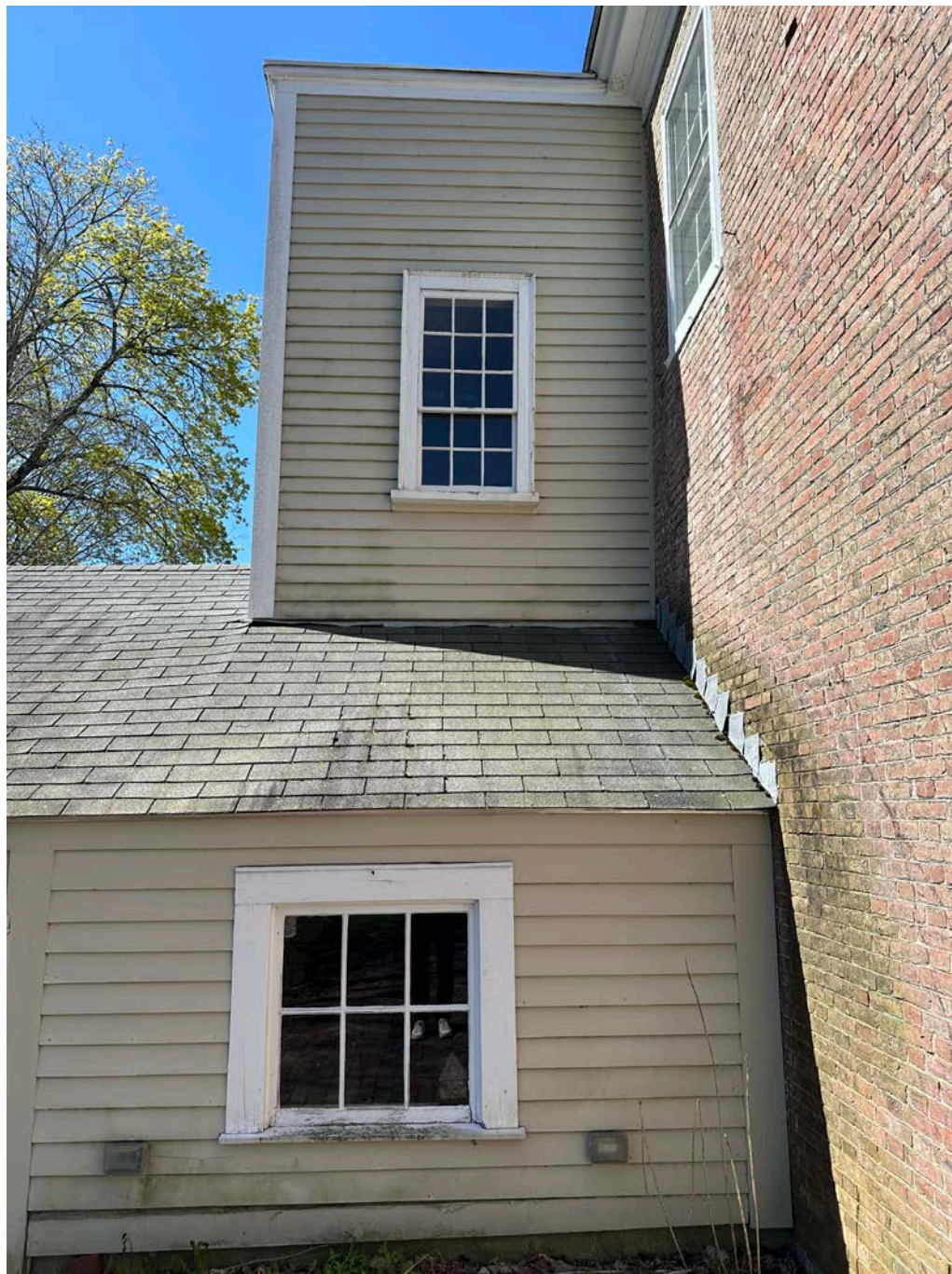
Figure 4.4-11 Window W-35 in the servant's room, north façade, was installed upside down, as its configuration should be six-over-nine instead of nine-over-six.
