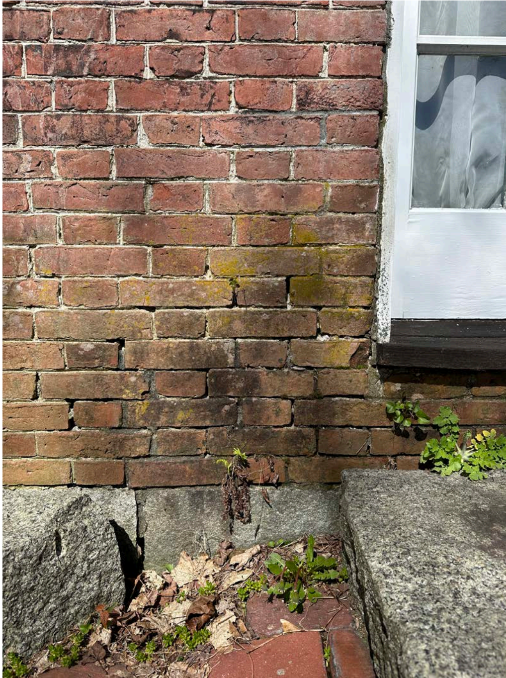
Figure 4.2-8 Several areas along the base of the building on the east elevation in which the mortar has deteriorated due to water infiltration, and in these gaps, small plants have taken root.
