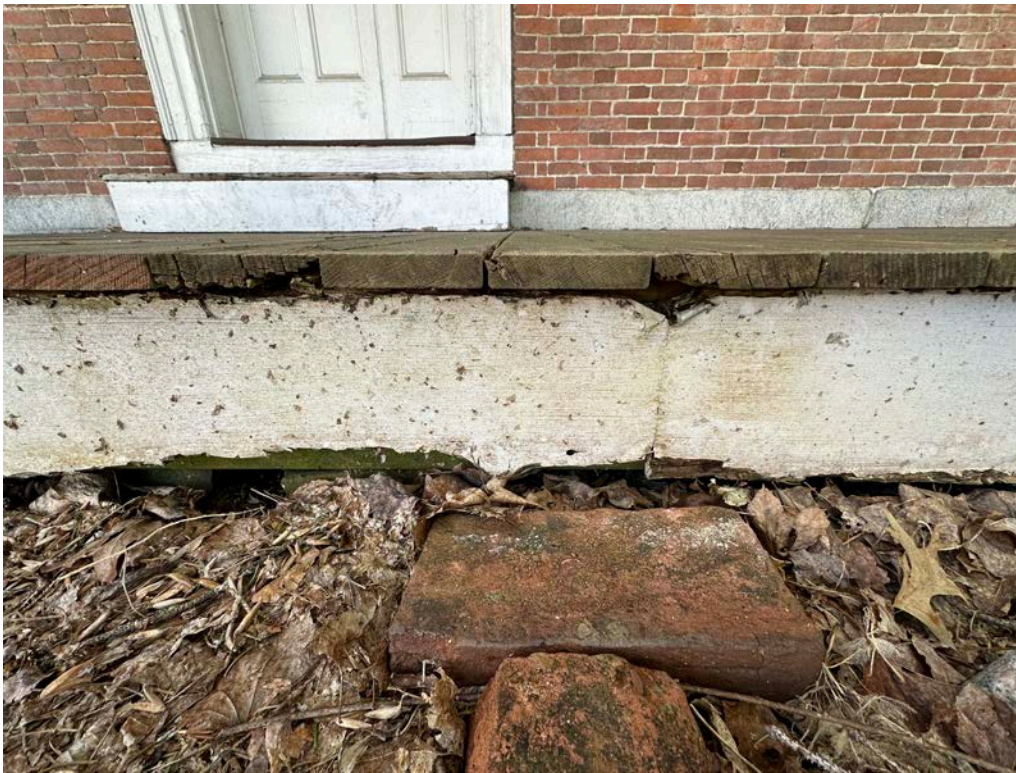
Figure 4.10-2 There is extensive mildew and mold on the deck fascia, most likely due to its proximity to the earth and surrounding vegetation and the section of fascia between the second and third columns is rotted through, the wood is cracked, and a portion of the fascia has fallen off.
