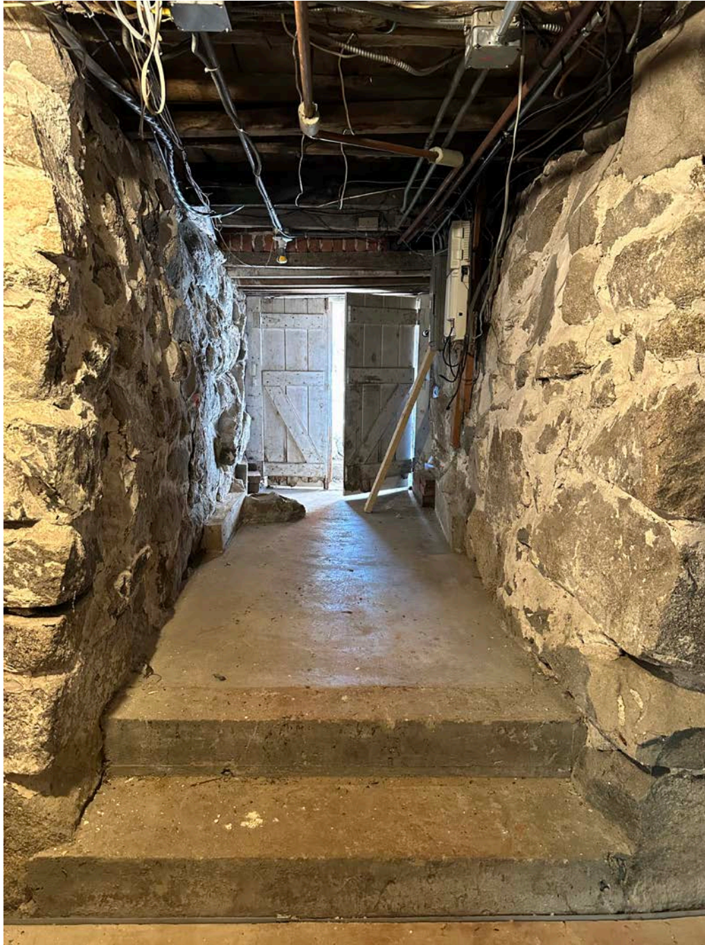
Figure 4.3-9 The basement is partially below-grade with an exterior access door along the south wall of the southwest addition. The foundation walls are constructed of ashlar masonry, which are also exposed in the basement.
