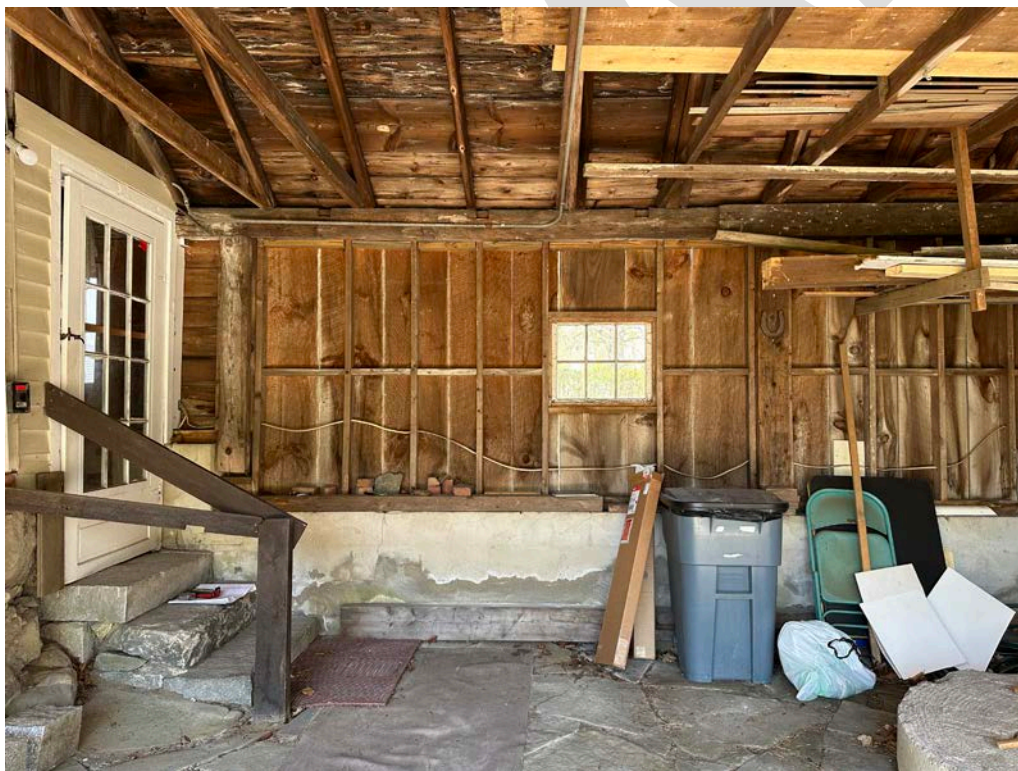
Figure 4.3-8 The foundation along the northern wall is constructed of concrete masonry units (CMU's) and timber. These foundations seem to have been restored in the recent past and are in good condition.
