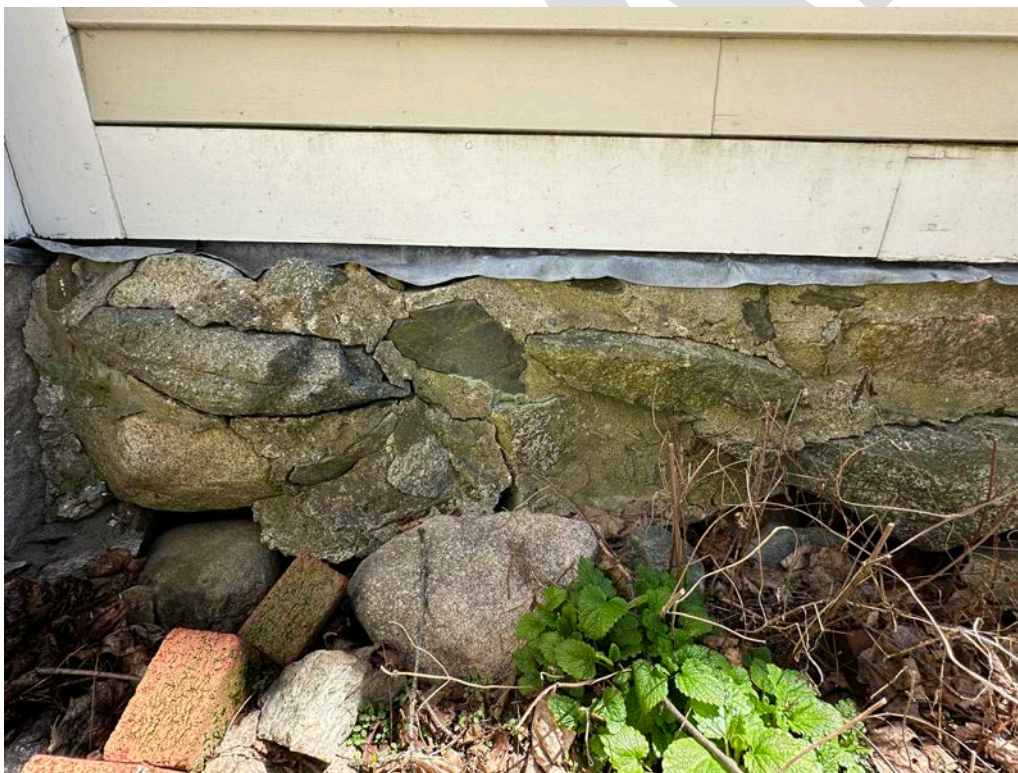
Figure 4.3-3 Base flashing was found in certain locations along the ashlar stone walls; however it is not entirely covering the foundation wall, and is bent out of shape in several locations.
