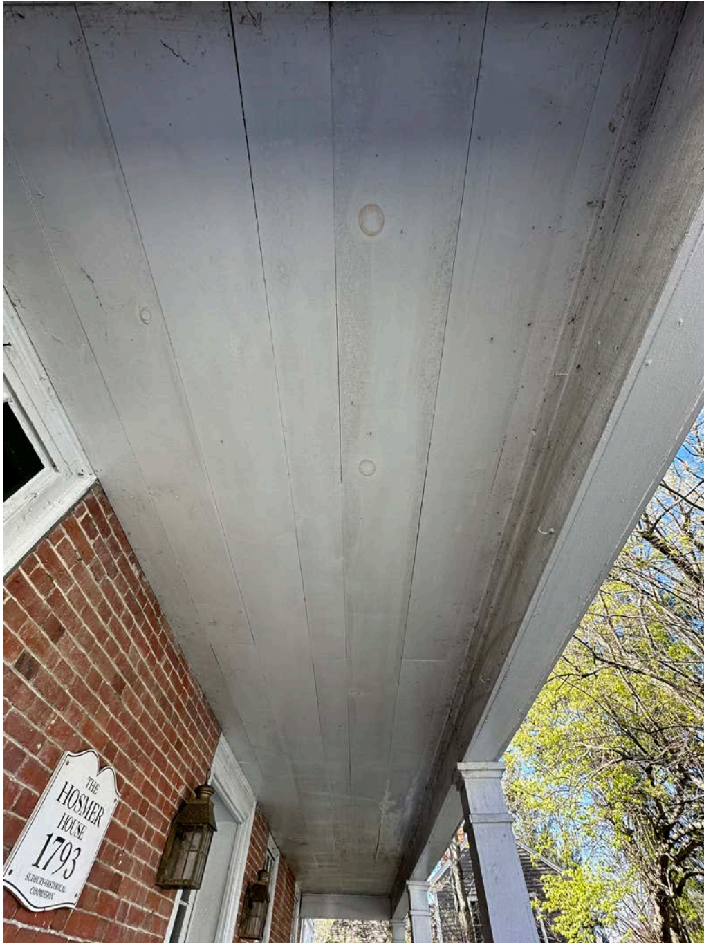
Figure 4.10-7 The porch ceiling is in good condition. The ceiling board at the underside of the roof is relatively new, however, oils are being drawn out from the knots in the wood, creating brown rings which telegraph through the white paint, typical throughout.
