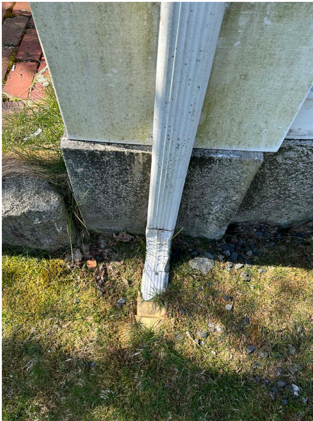
Figure 4.3-5 There is no evident base flashing between the wood pilaster and the granite foundation.
