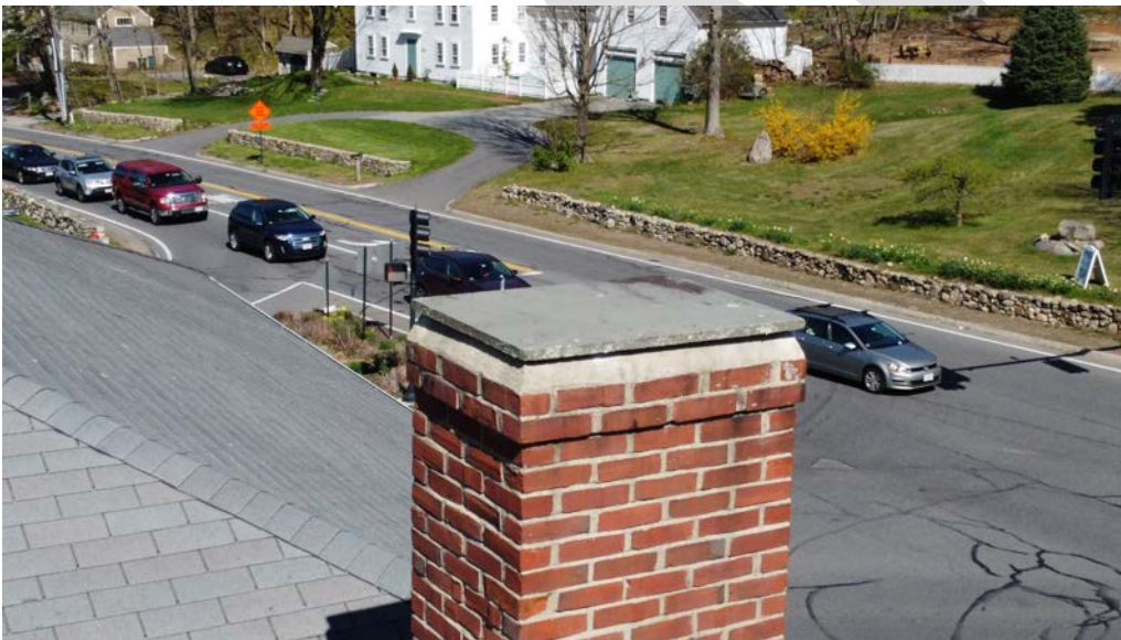
Figure 4.9-2 All chimneys are laid in stretcherbond pattern. Just below the coping stone the chimneys is crowned with two courses of protruding brick and cement, creating a drip edge.
