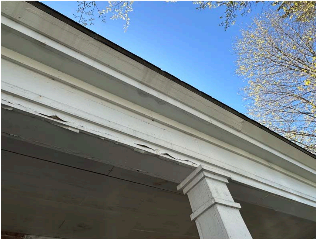
Figure 4.10-8 The frieze board and fascia of the porch roof have as well been replaced.
