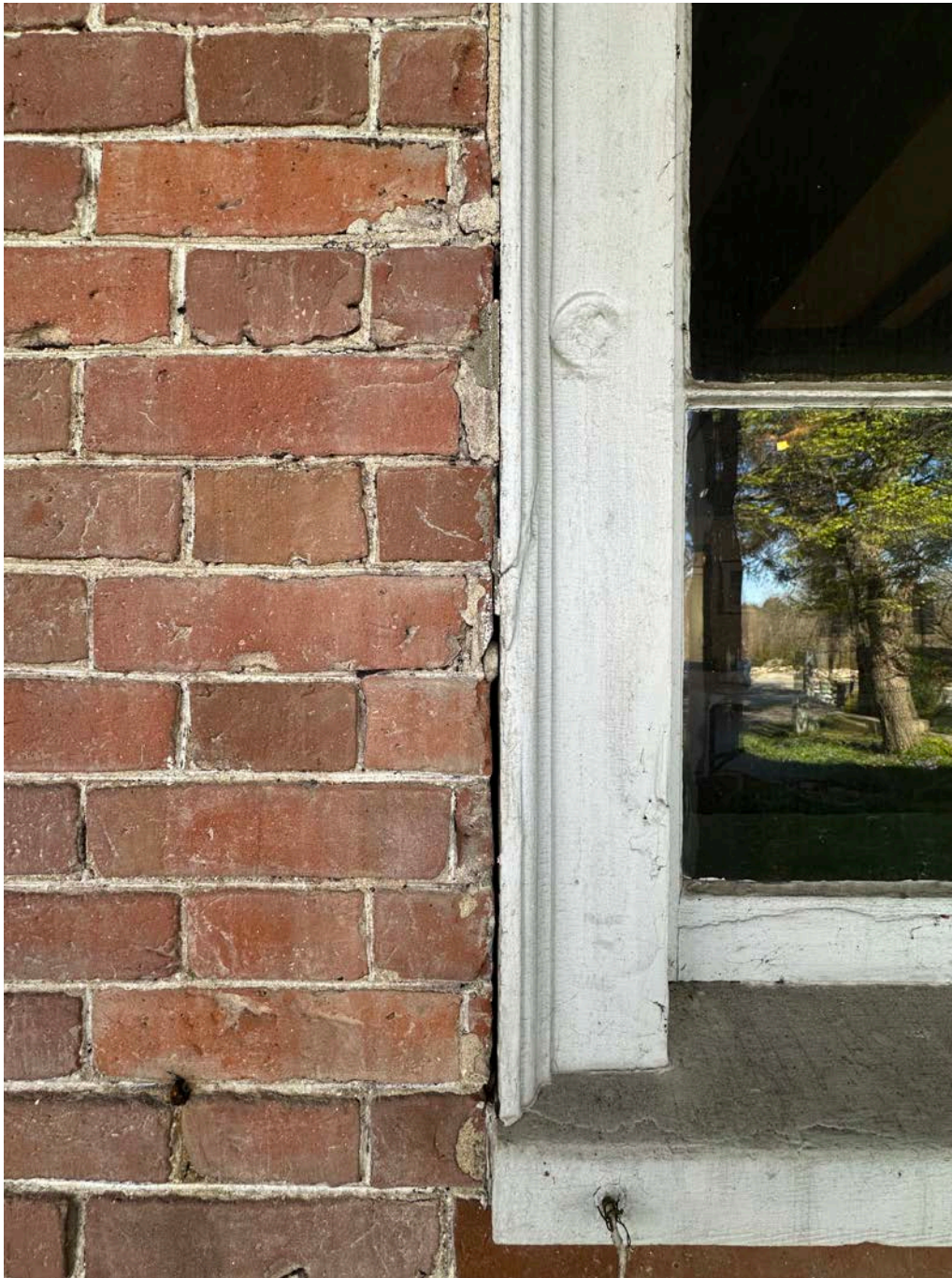
Figure 4.4-14 The perimeter sealant and glazing putty around the windows appear deteriorated, with cracks and gaps in some locations, leading to poor performance.
