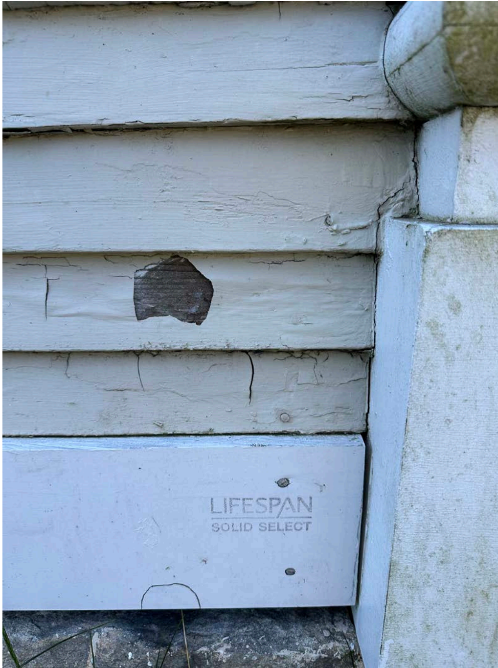
Figure 4.1-6 Blistering paint on butt-beveled clapboard.
