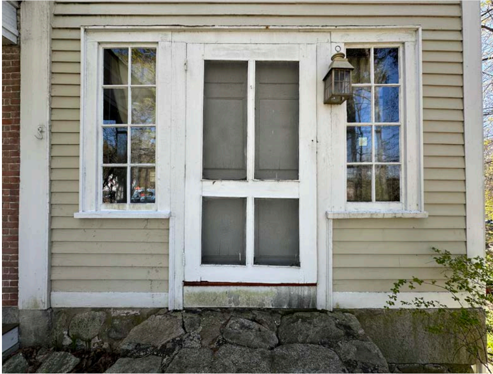
Figure 4.4-2 Two vertical fixed wood windows flanking the office entrance door (D-21). The screen door was found to be damaged and inappropriate in design.
