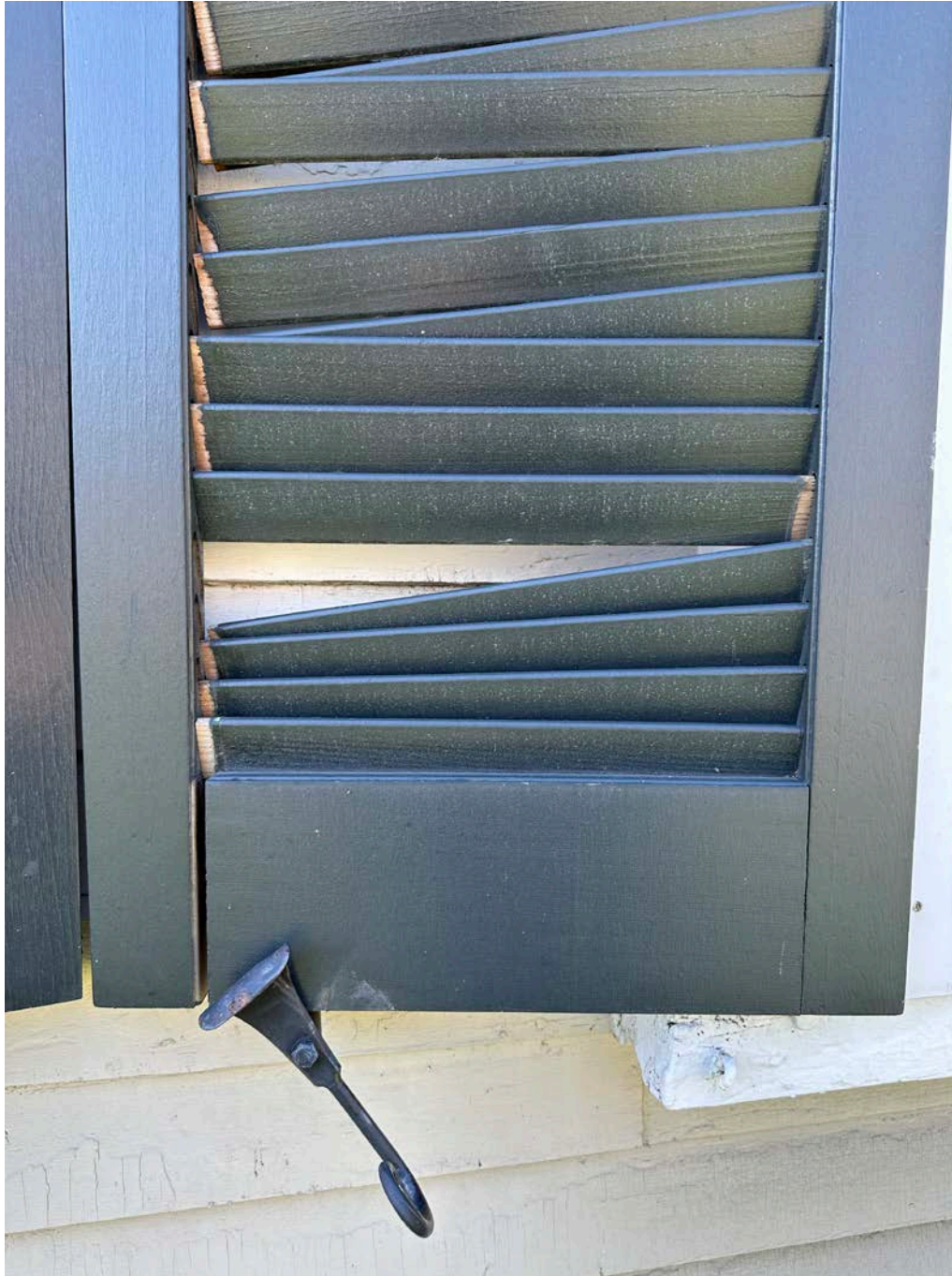
Figure 4.6-2 Louvers which have fallen out of place. Typical condition seen throughout.
