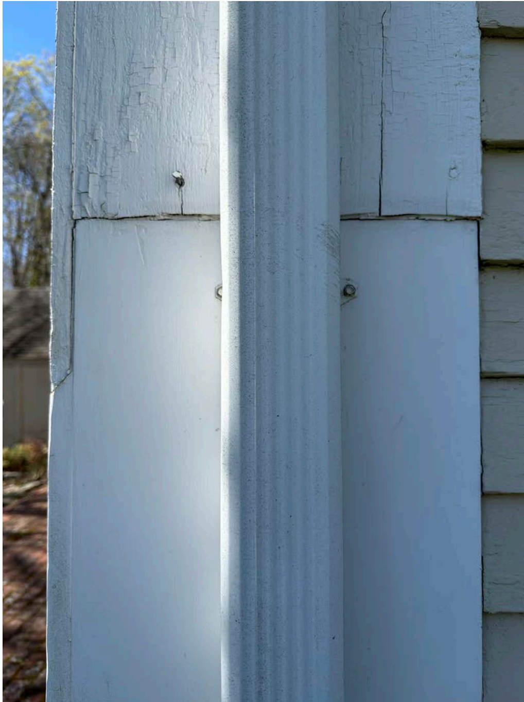
Figure 4.1-14 At the joint of the repaired pilasters, there are several splits in the wood ranging from 8 inches to 2 feet in length.
