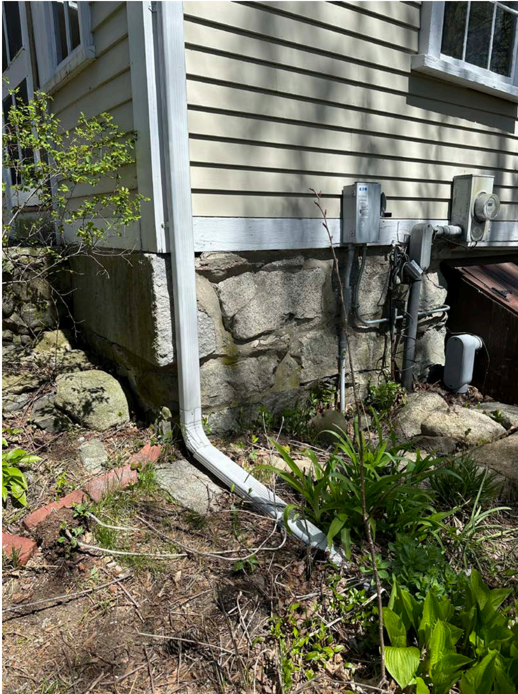
Figure 4.8-8 This downspout terminates an appropriate distance from the house's foundation, and expels water above grade.
