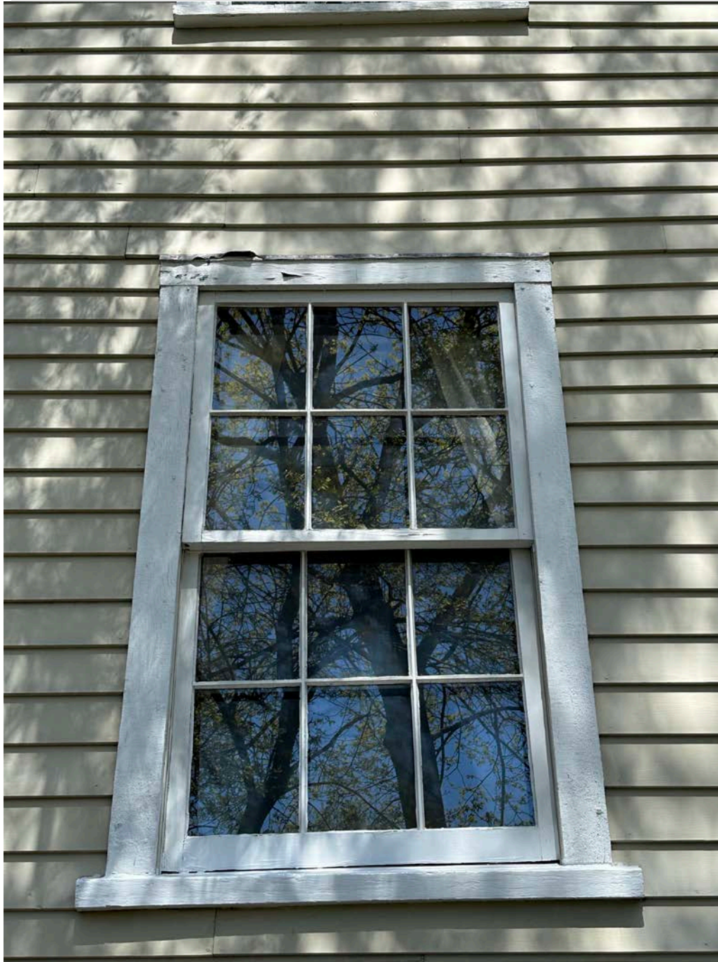
Figure 4.4-15 Metal window head flashing was noted at most windows but appears bent or poorly installed in some areas.
