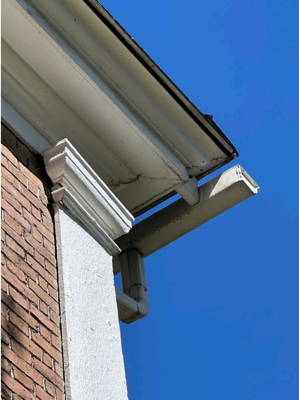
Figure 4.8-3 Along the north elevation, a gutter was installed along the roofline, supported by wood blocking.
