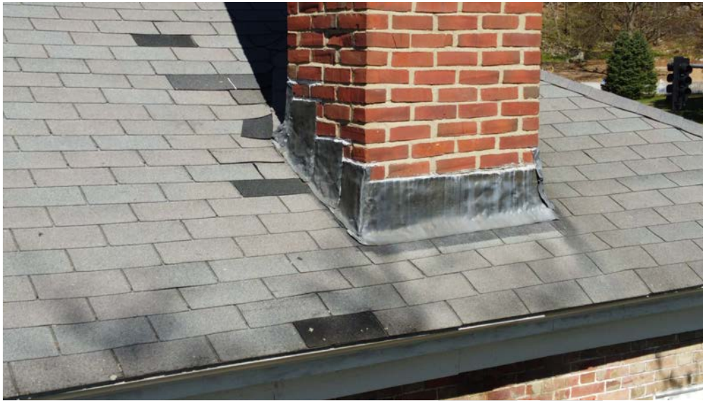
Figure 4.9-3 The step-flashing around the chimneystack s and crickets is in poor condition due to general end-of-life degradation as edges of the flashing are upturned and portions of the step-flashing are separating.
