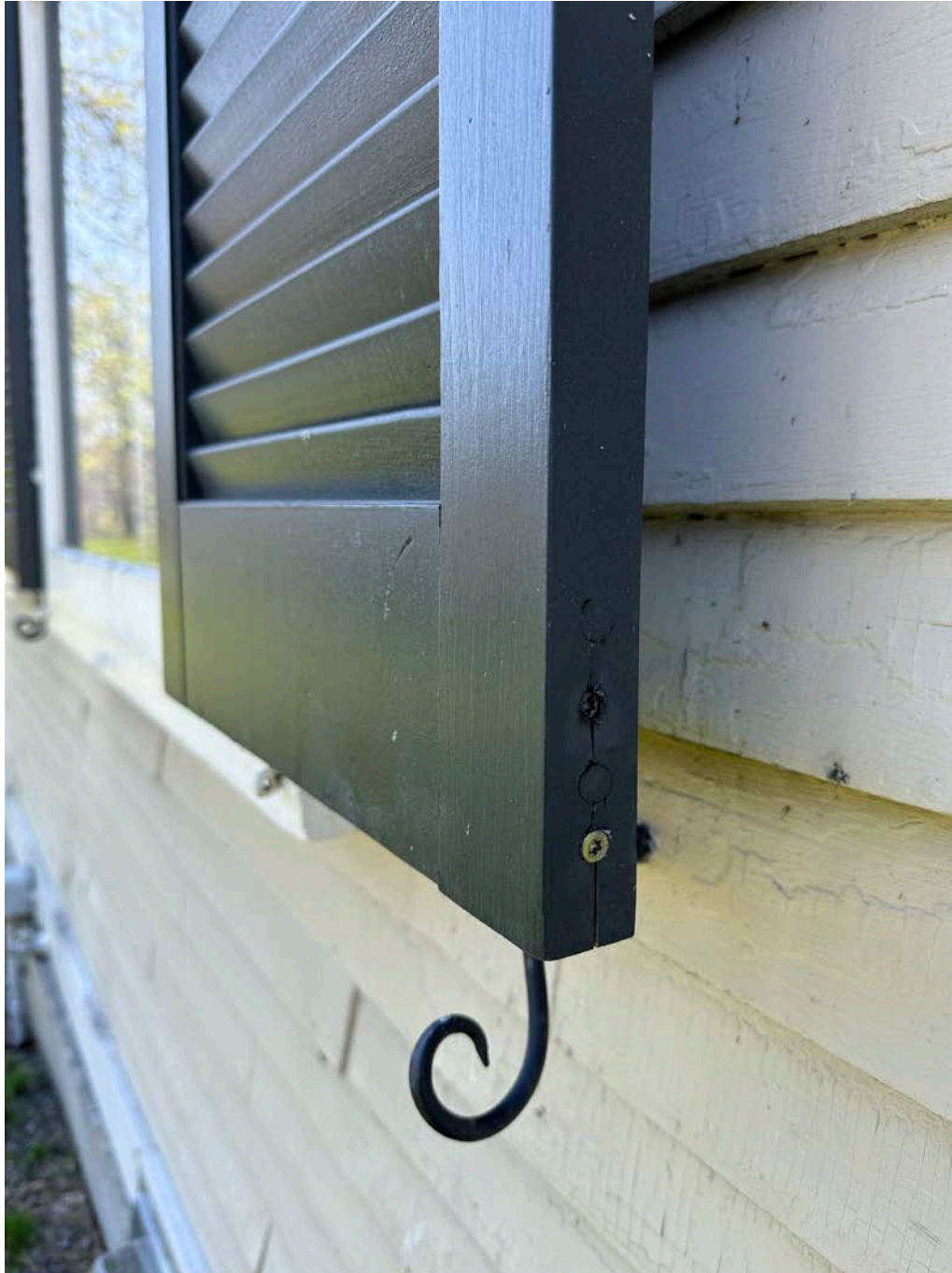
Figure 4.6-3 Instances where the bottom rail of the shutter has become loose. A repair had been made by inserting a screw into the side of the stiles, through to the bottom rail, however this seems to have failed as well, as the wood around the screw is now splitting.
