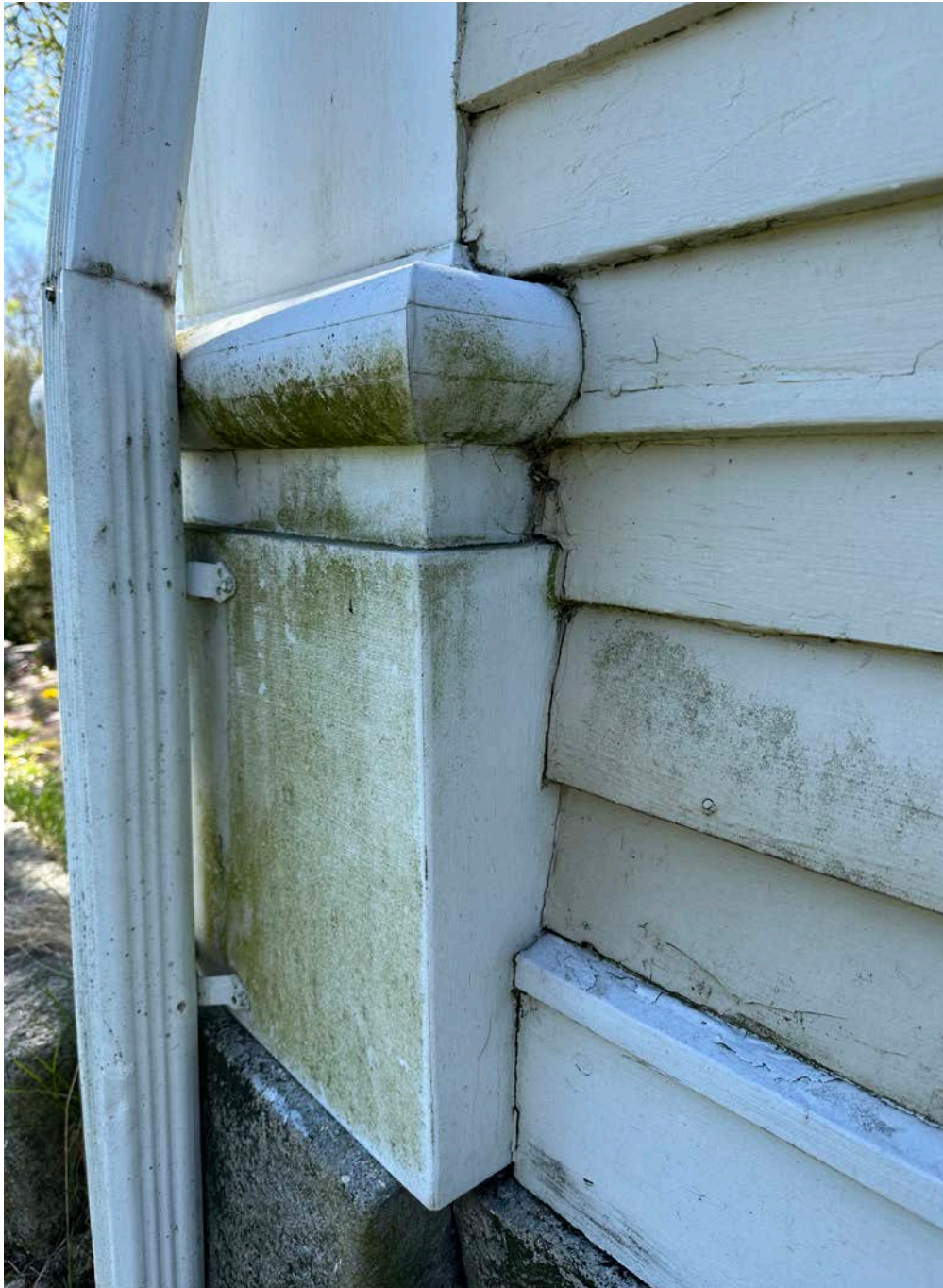
Figure 4.1-16 Both bases of the pilasters are covered in a slight layer of biological growth and mildew due to excessive moisture on the surface of the wood, and the proximity of vegetation to the lower elements of the building.
