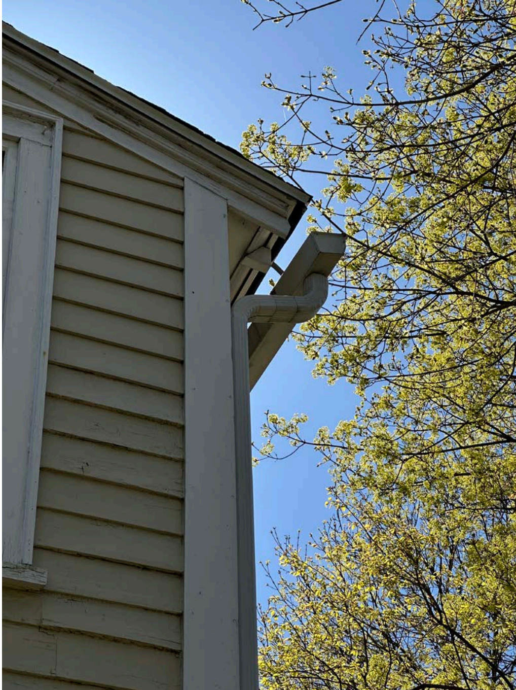
Figure 4.8-7 This gutter is fastened to the roof rafter at the southeast corner with a spike-and-ferrule, while the remaining length of gutter is fastened using strap hangers, which were installed atop the roof membrane, rather than below.
