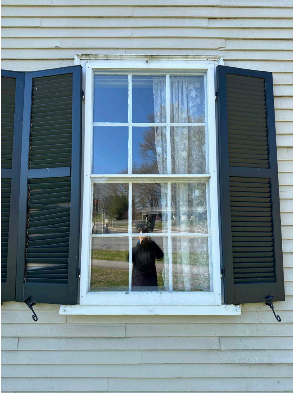
Figure 4.4-10 The storm windows are non-operable and are screwed to the wood casing. One storm window on the north façade (W-05) was installed upside down.
