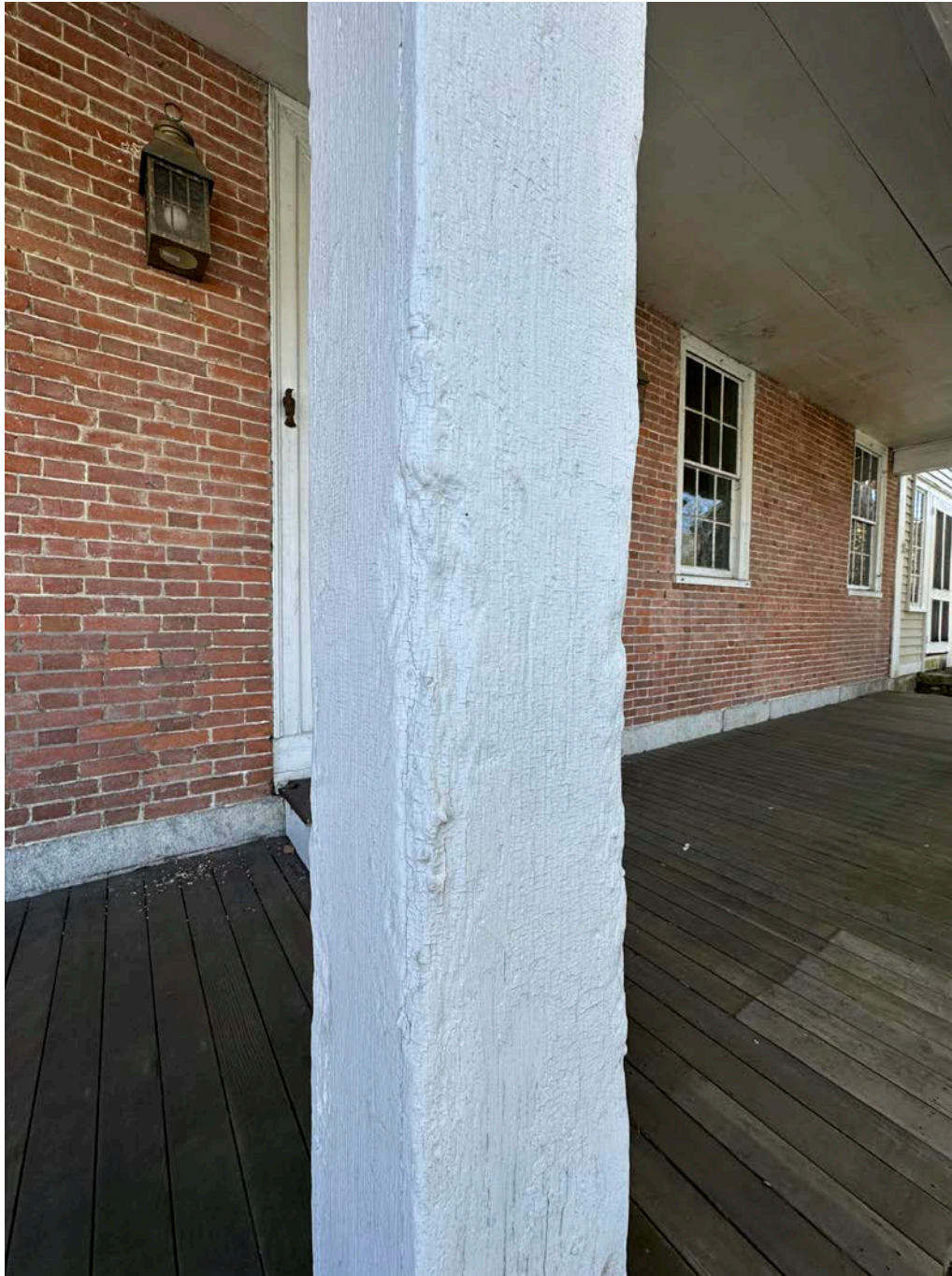
Figure 4.10-4 The 4 columns which support the porch roof are in poor-to-fair condition. The shaft of the columns have degraded over time, and have lost material mass at various locations.
