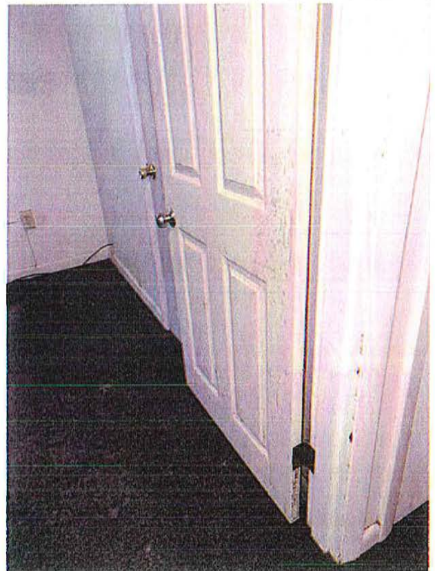
A bedroom door needs replacement.
