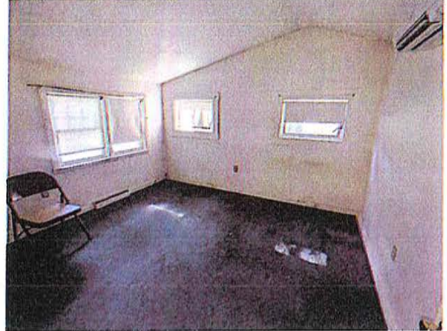
The carpet and interiors need replacement.
