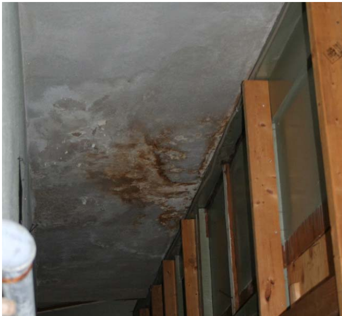
Figure 1. A fairly large area on the second floor ceiling shows water damage, the result of leaks that appear during heavy rains.
