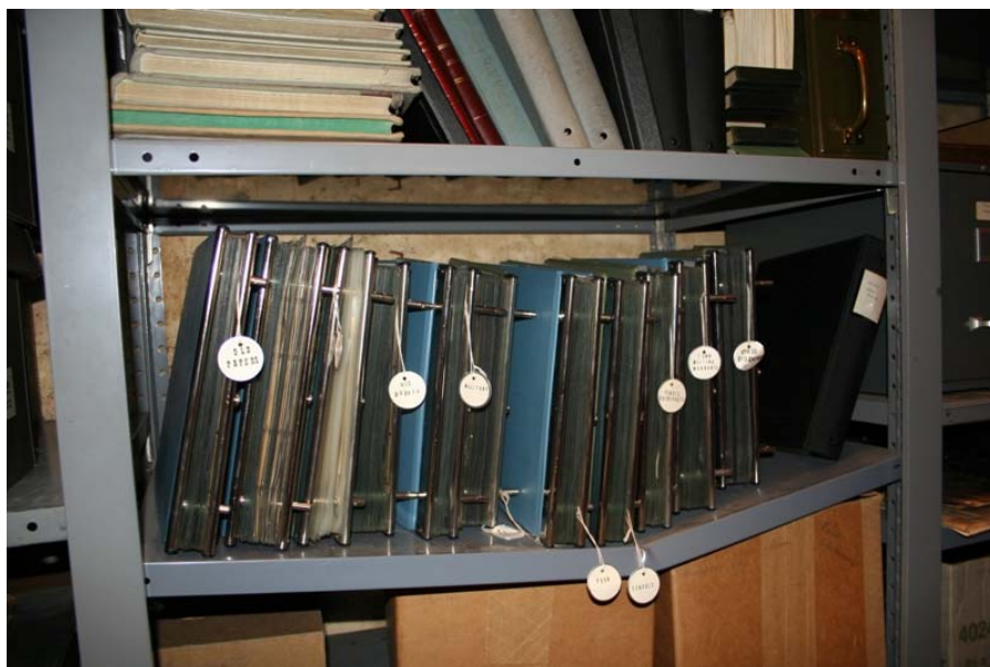
Figure 5. One shelf in the basement vault buckles under the weight of the volumes stored on it.
