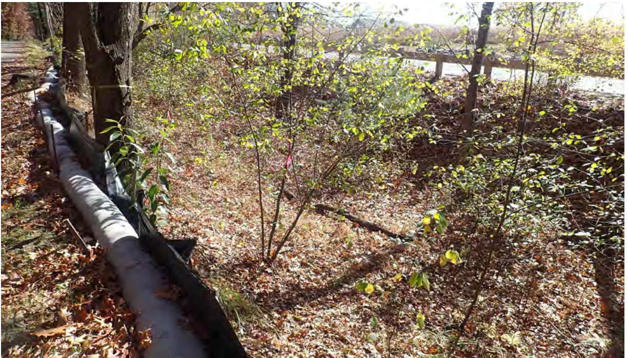
Photo #2: View of installed downed tree in Segment 11 near condominium complex. No sediment or construction debris observed within the resource area or beyond the silt fencing. Silt fencing are in good condition. Facing east.
