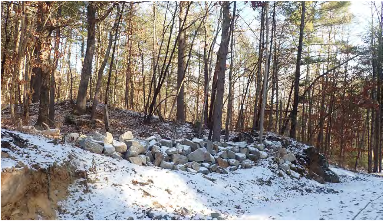
Photo #3: View of installed rock pile in Segment 10, east of Peakham Road. Facing northeast.
