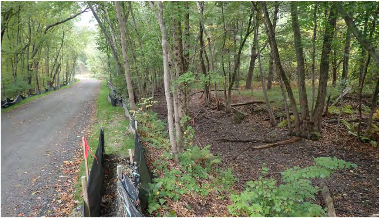
Photo #3: View of installed fallen logs in Segment 14. Silt fencing in this area is in good condition. No sediment or debris observed in the resource area or associated buffer zones. Facing west.
