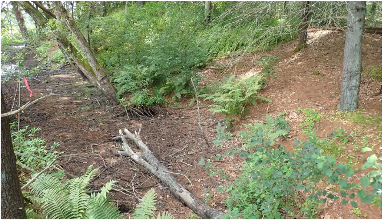
Photo #3: View of installed downed tree within wetland west of Bridge 127 in Segment 13. Silt fencing is in good condition. No sediment or debris observed in the resource area or associated buffer zones. Facing east.
