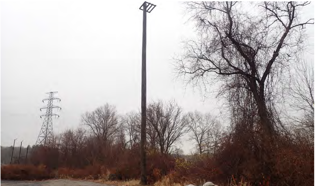
Photo #14: View of installed osprey nest by the Sudbury Substation. Facing south.
