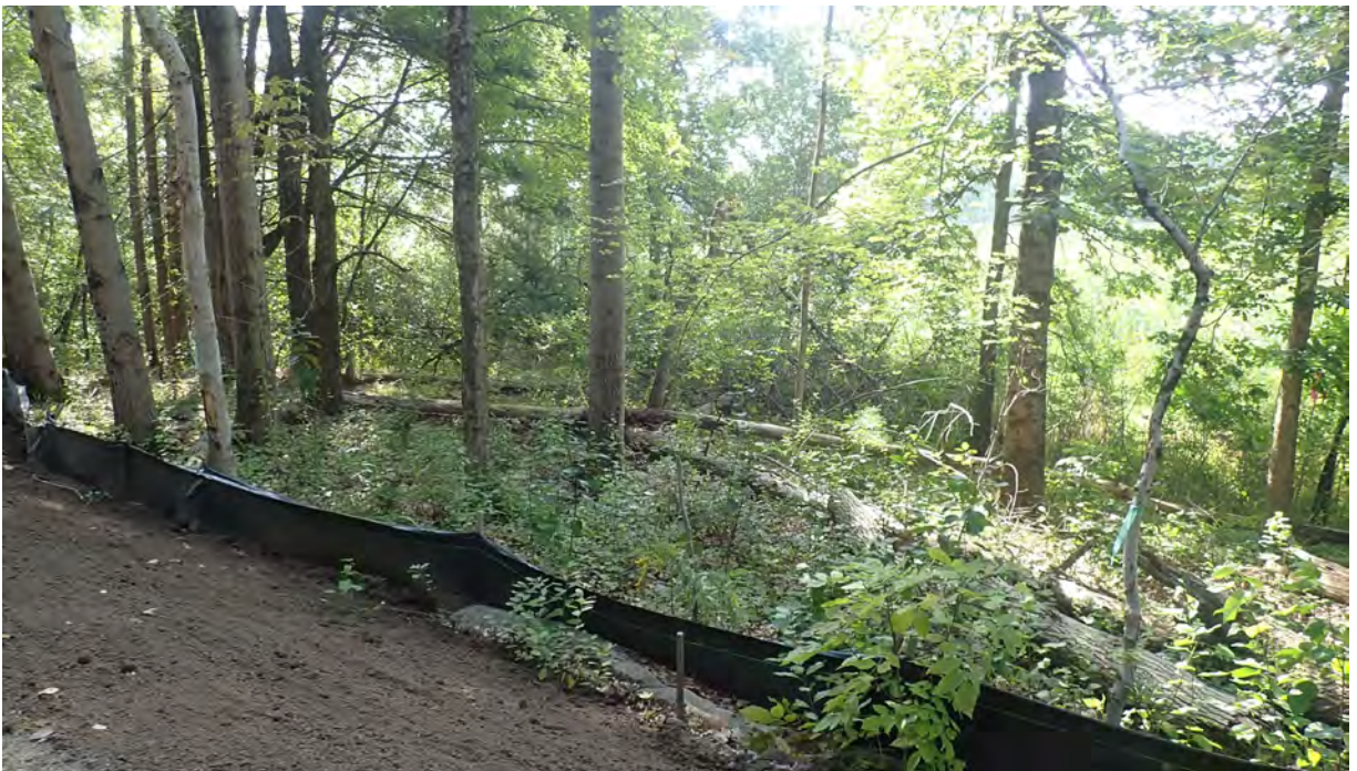
Photo #4: View of installed downed tree in Segment 14. Area adjacent to the silt fencing has been prepared for planting installation. No sediment or debris observed within the resource area. Facing south.
