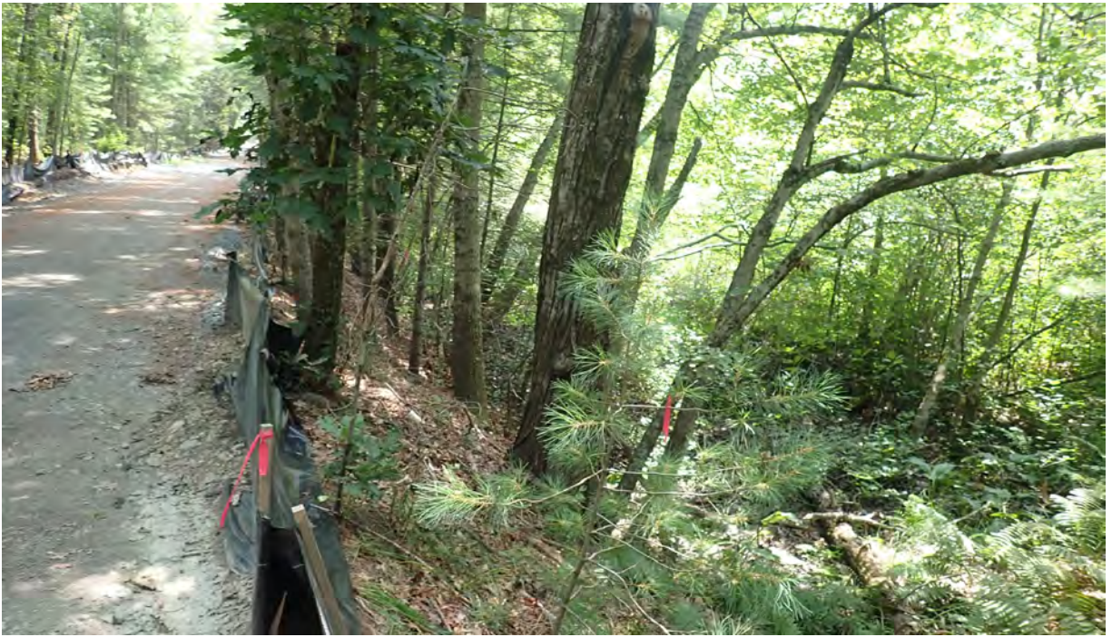
Photo #1: View of installed downed tree within vernal pool #5 in Segment 8. No sediment or debris observed within the resource area. Facing east.
