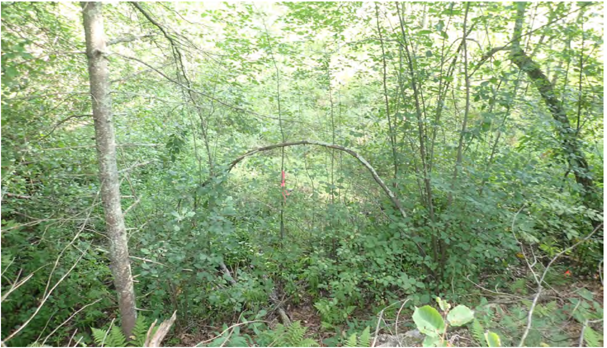
Photo #1: View of installed downed trees in Segment 7. Silt fence in the area is in good condition. No sediment or debris observed within the resource area. Facing north.
