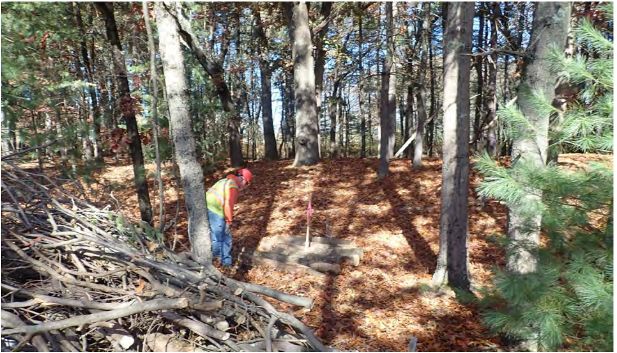
Photo #3: View of brush pile installation in Segment 11. Silt fencing in this area is in good condition. No sediment or debris observed in the resource area or associated buffer zones. Facing north.
