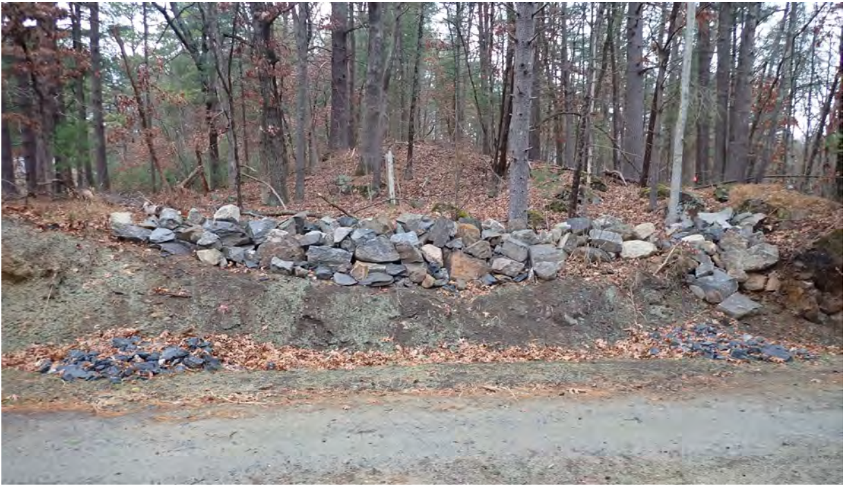
Photo #5: View of installed rock pile in Segment 10, east of Peakham Road. Facing north.
