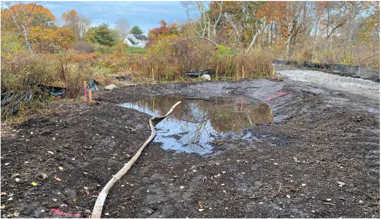
Photo #5: View of the wetland mitigation area after area was graded. Photo taken October 27, 2023. Facing west.
