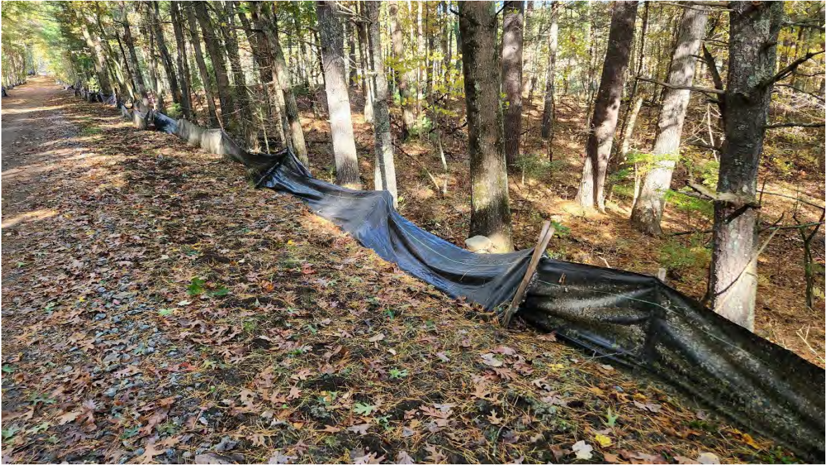
Photo 2: Broken stakes in the silt fence along segment 8. Photo taken on 10/15/24
