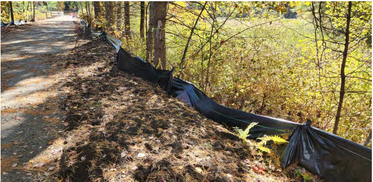
Photo 1: Broken stakes in the silt fence along segment 7. Photo taken on 10/15/24
