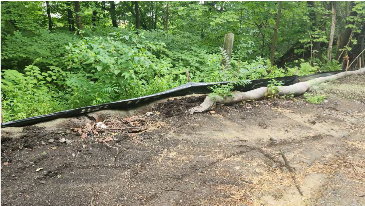
Photo 6: Filter tube is damaged and needs to be replaced along segment 13. Photo taken on 8/09/24.
