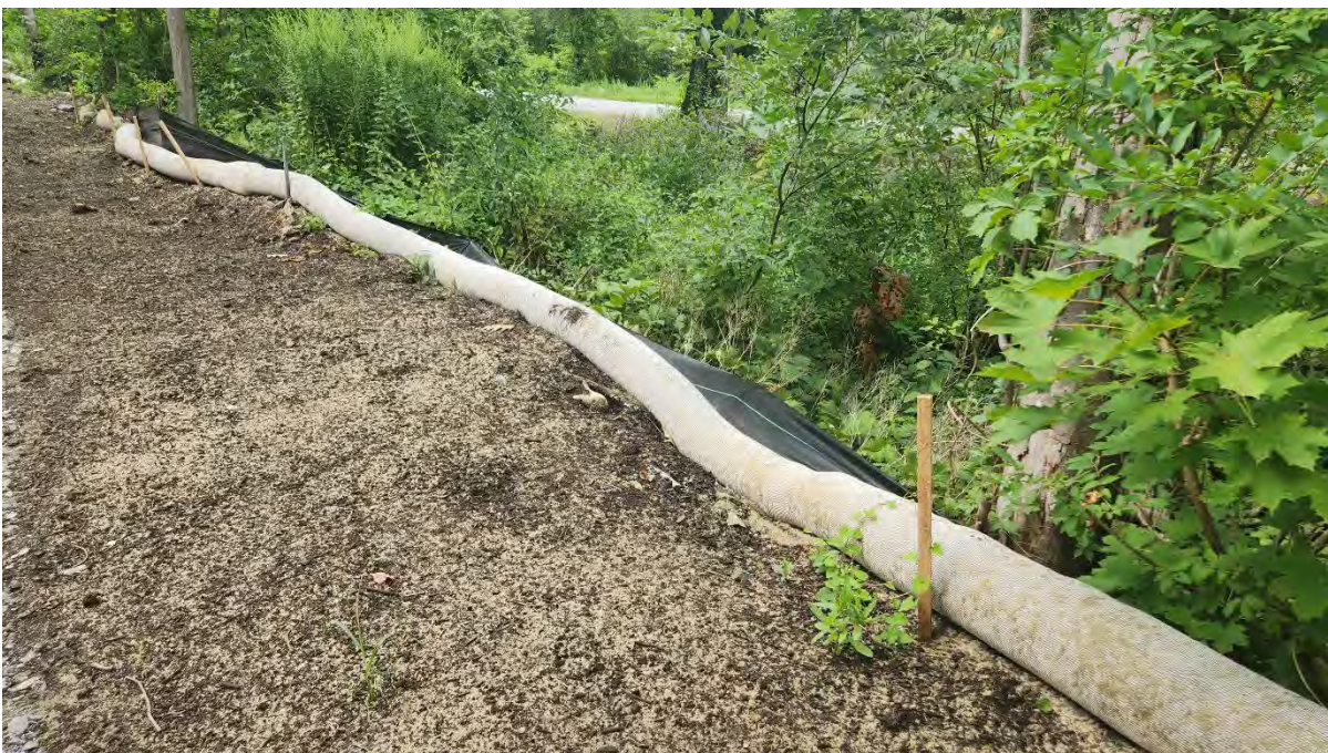
Photo 5: Broken stakes found in the silt fence along segment 12. Photo taken on 8/09/24.
