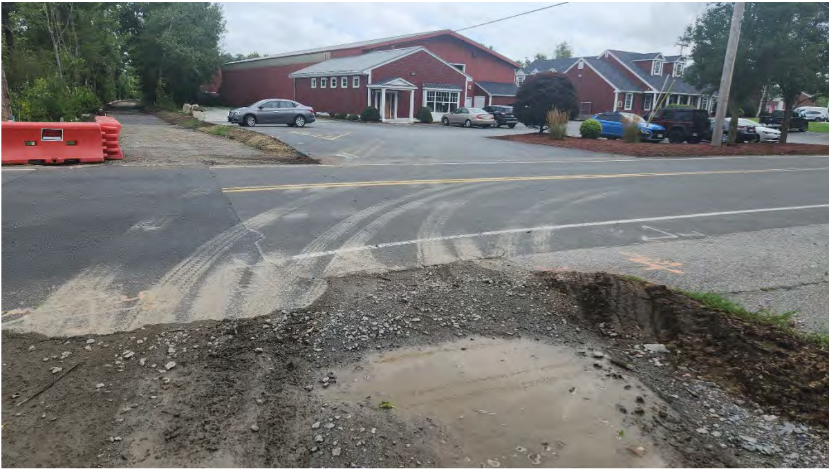
Photo 4: Sediment tracked into the road at construction entrance STA 407+50. Photo taken on 8/09/24
