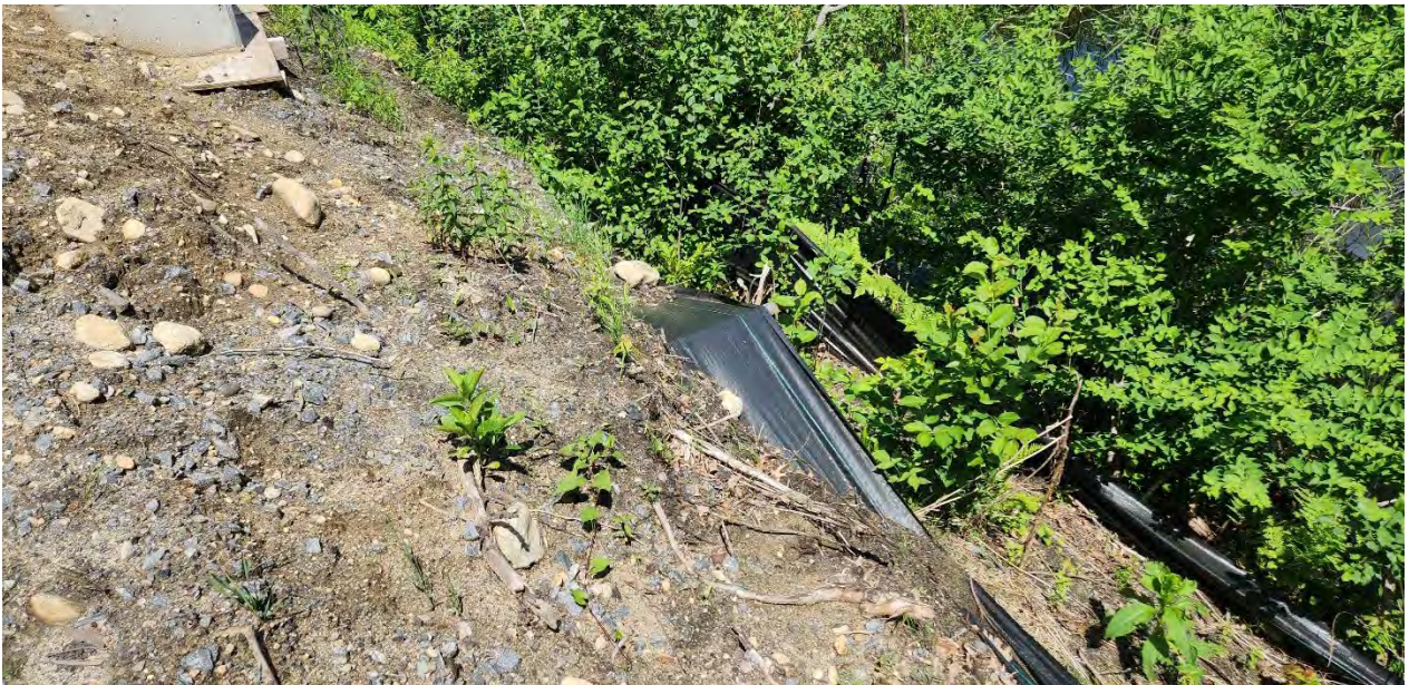
Photo 1: Broken stake in the silt fence along segment 8 near bridge 128. Photo taken on 5/31/24
