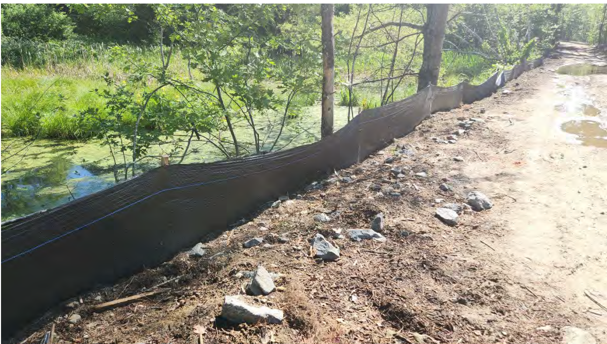
Photo 5: Newly installed silt fence along segment 14. Still awaiting new filter tube. Photo taken on 5/31/24.
