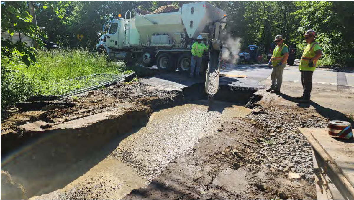
Photo 4: Concrete being poured over installed duct banks at Boston Post Road along segment 12. Photo taken on 5/31/24
