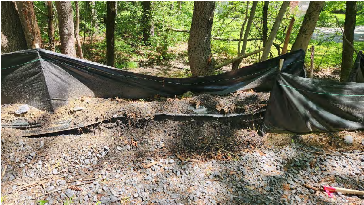
Photo 2: Silt fence untucked but above grade along segment 9. Photo taken on 5/31/24
