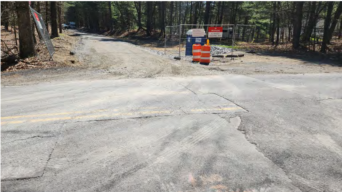
Photo 5: Sediment tracked into the road at gravel construction entrance STA 305+00. Photo taken on 4/22/24.
