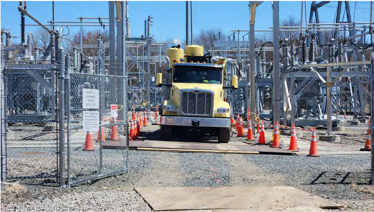
Photo 6: Vacuum truck removing sediment for conduit installation at Eversource substation. Photo taken on 4/22/24.
