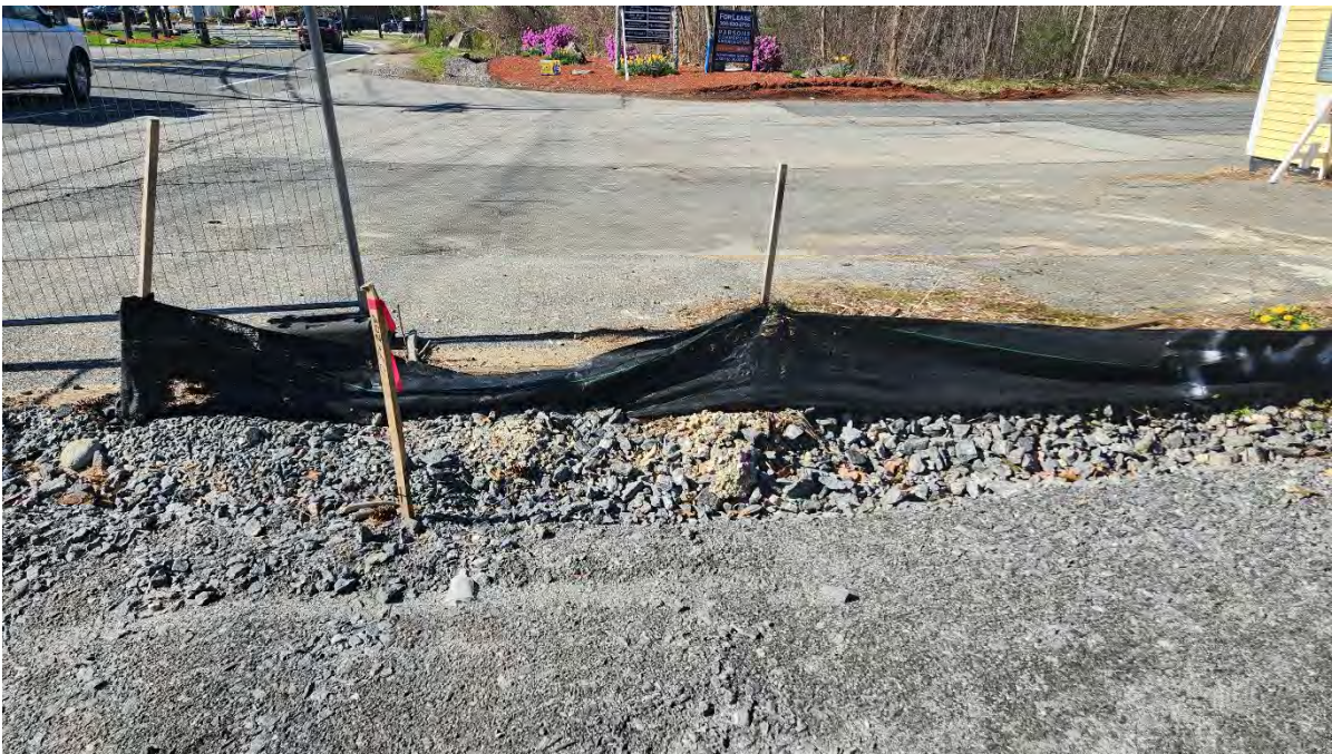
Photo 3: Ripped silt fence along segment 11. Photo taken on 4/22/24
