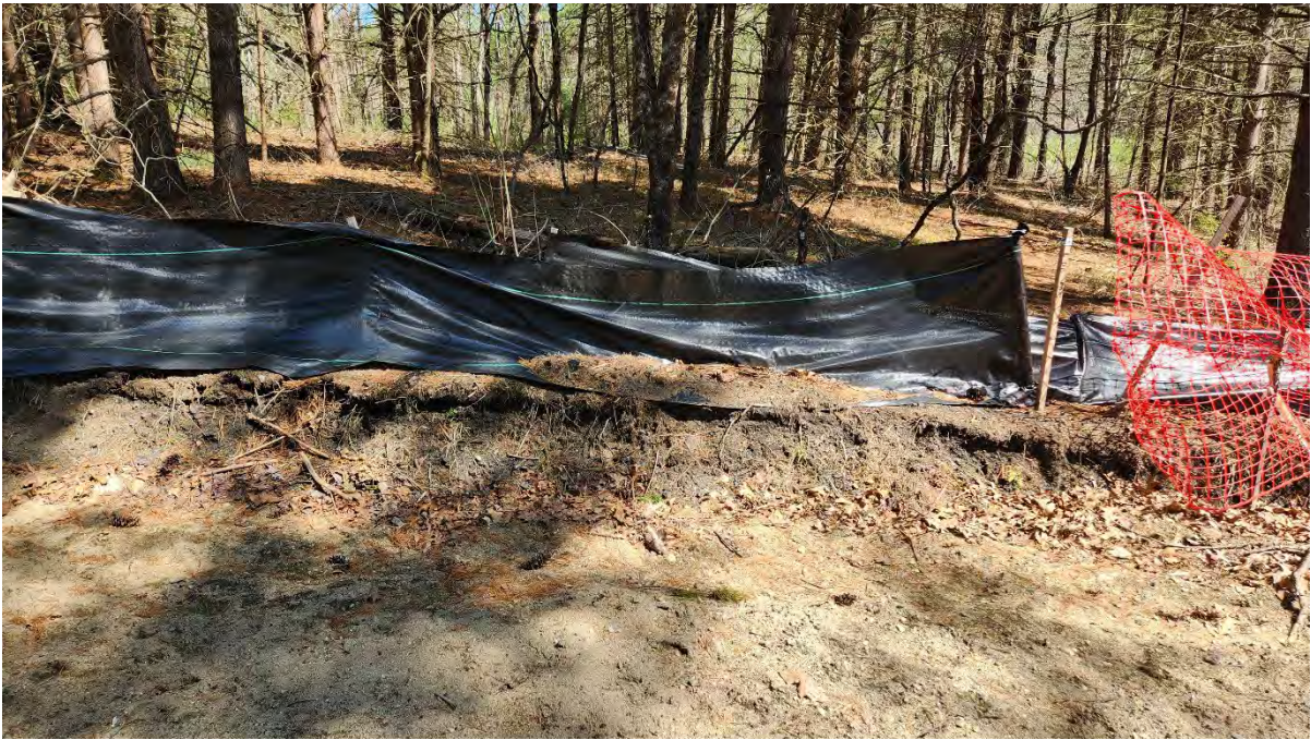
Photo 2: Exposed silt fence along segment 7. Photo taken on 4/22/24
