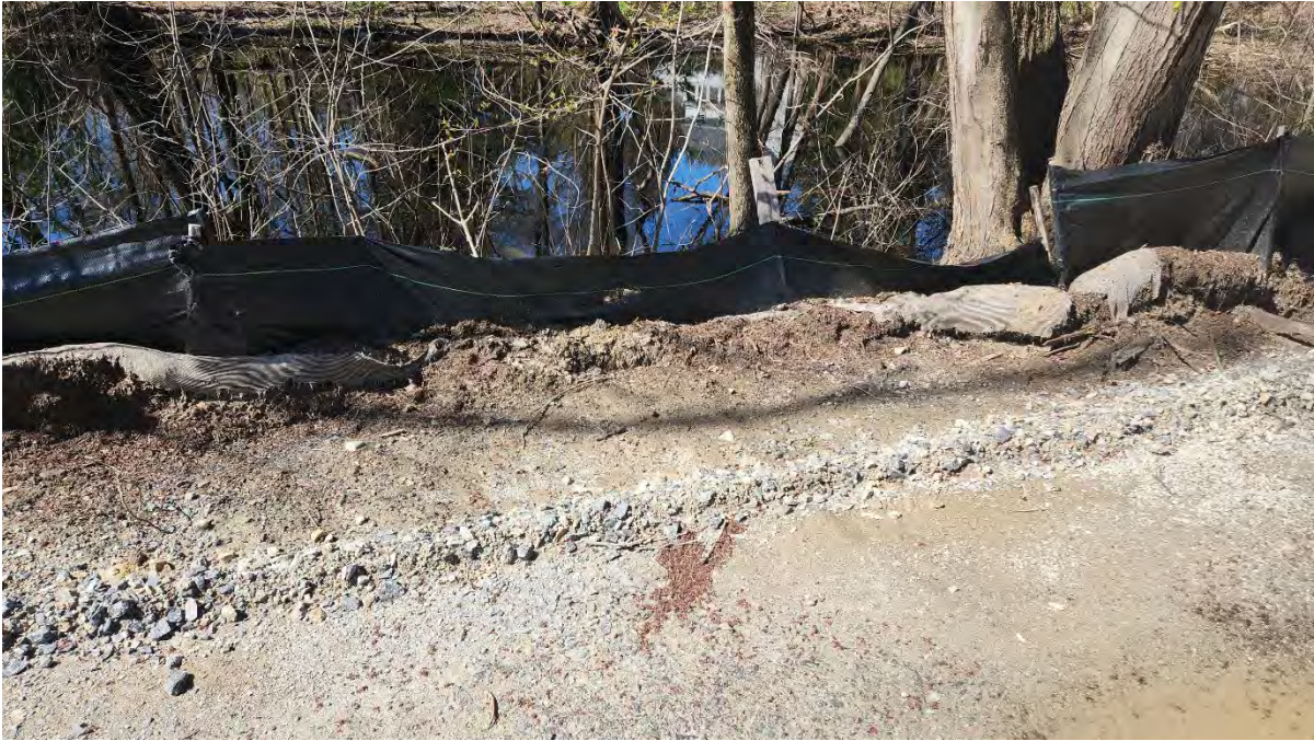
Photo 4: Broken stake and damaged filter tube along segment 14. Photo taken on 4/22/24
