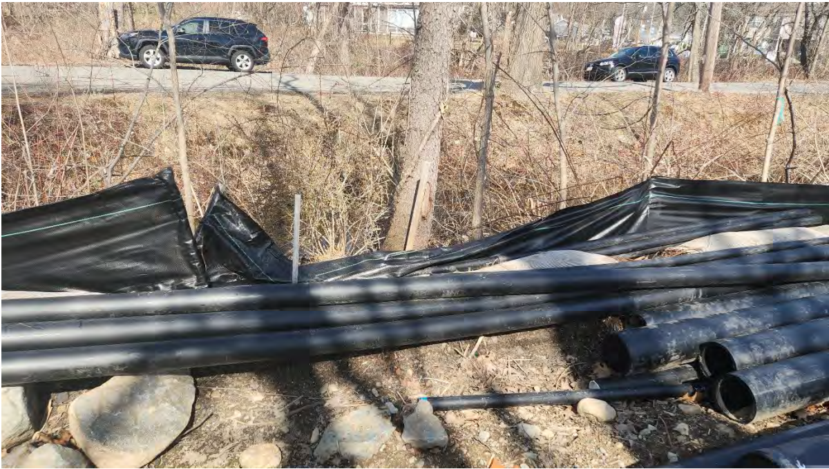
Photo 4: Ripping in the silt fence along segment 12. Photo taken on 3/27/24
