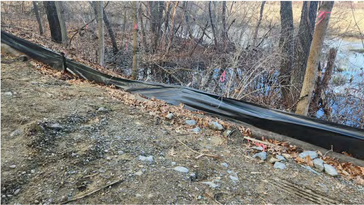
Photo 6: Broken stake in silt fence along segment 13. Photo taken on 3/27/24.
