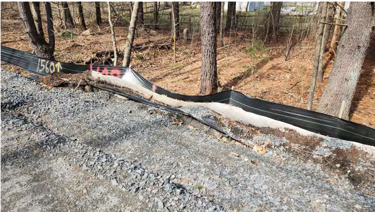
Photo 3: Broken stake and sagging in silt fence along segment 9. Photo taken on 3/27/24
