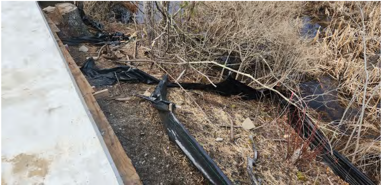
Photo 1: Broken stake in silt fence at Bridge 128 along segment 8. Photo taken on 3/27/24
