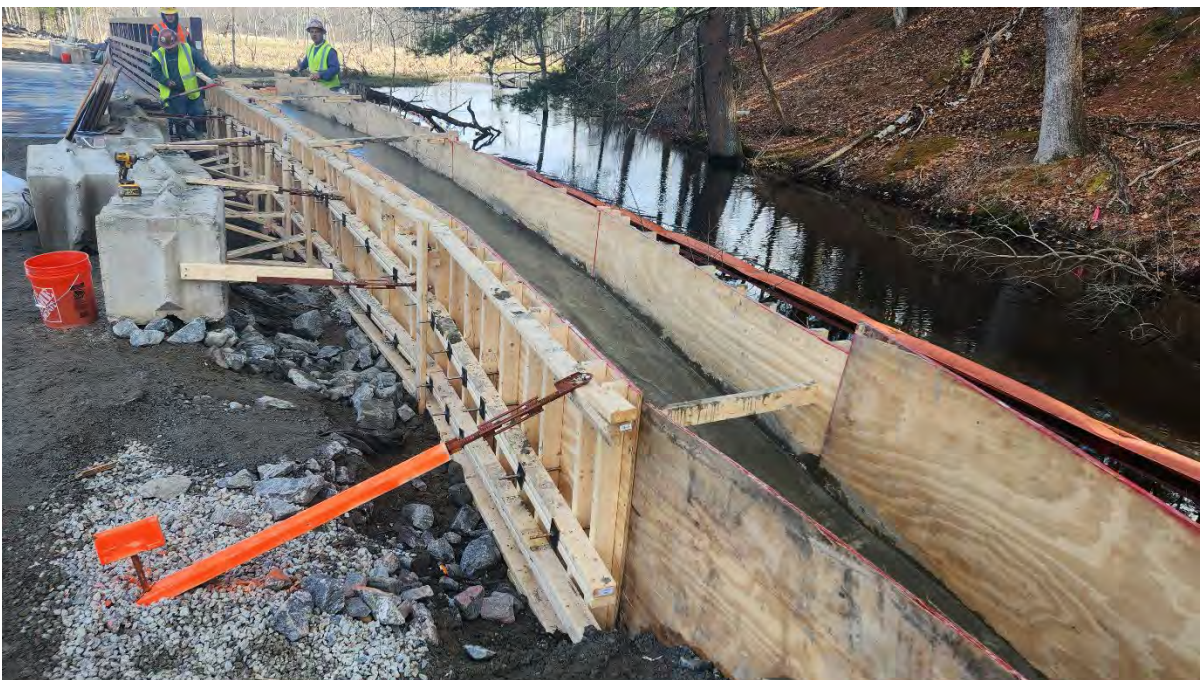
Photo 5: Wall cap installation under progress at Bridge 127 along segment 13 Photo taken on 3/27/24.
