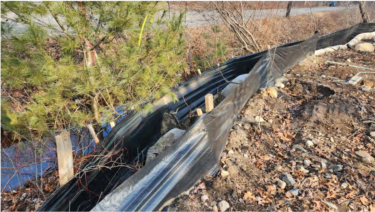
Photo 4: Extra support installed in the silt fence along segment 12. Photo taken on 2/27/24
