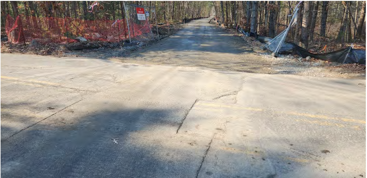
Photo 1: Sediment being tracked onto the road at construction entrance STA 305+00. Photo taken on 2/27/24
