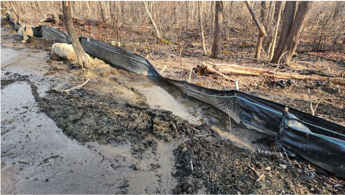
Photo 6: Broken stake in silt fence along segment. Photo taken on 2/27/24.
