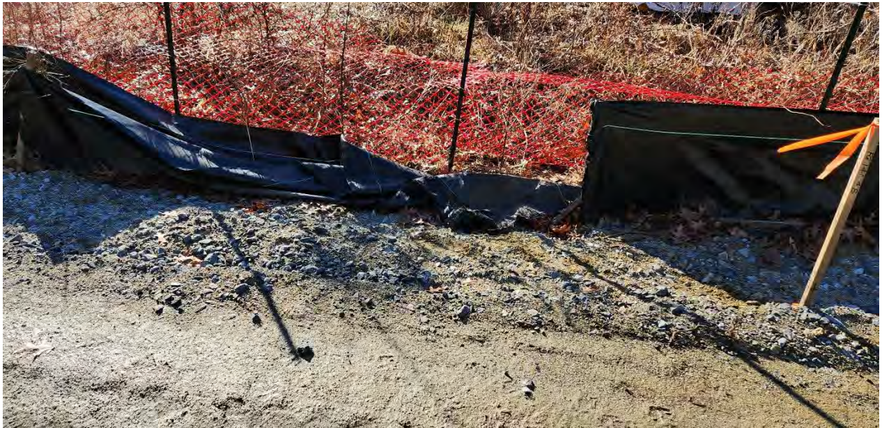
Photo 1: Rip in the silt fence along segment 11. Photo taken on 12/14/23
