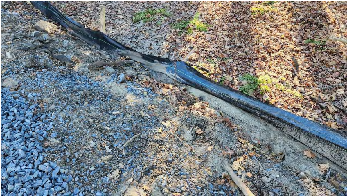
Photo 3: Broken stake in the silt fence along segment 13. Photo taken on 12/14/23
