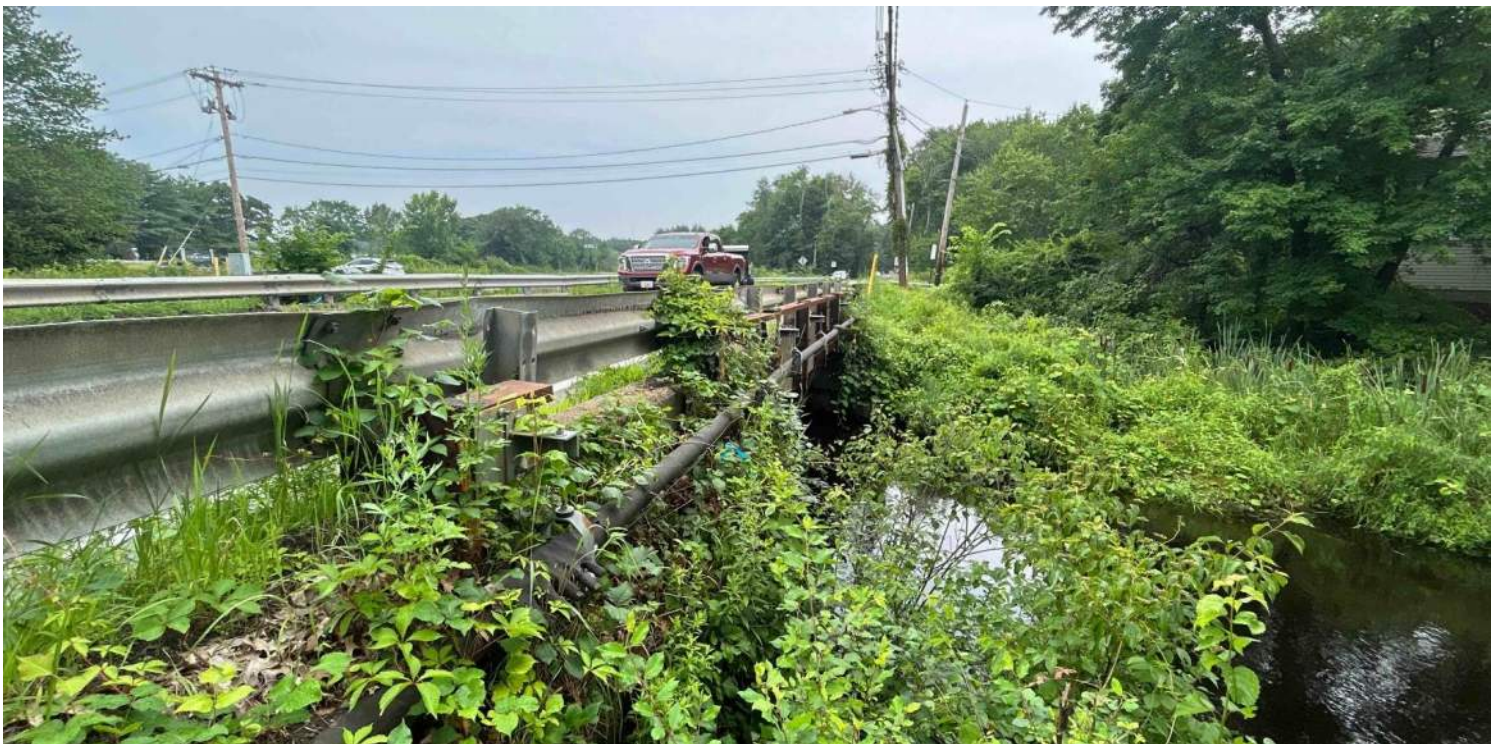
Photo #2: View of the exposed gas main on Union Ave bridge. Facing north.
