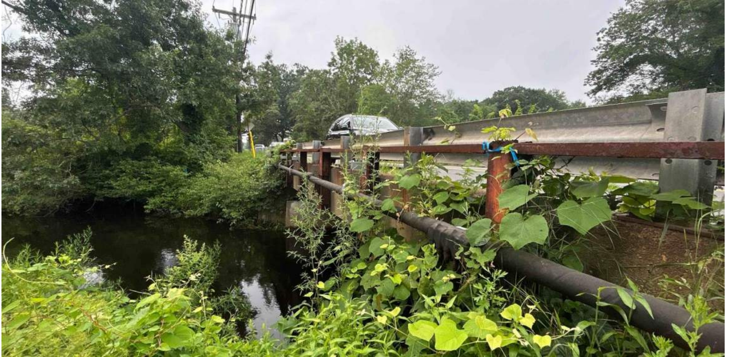
Photo #3: View of the exposed gas main on Union Ave. Facing southwest.
