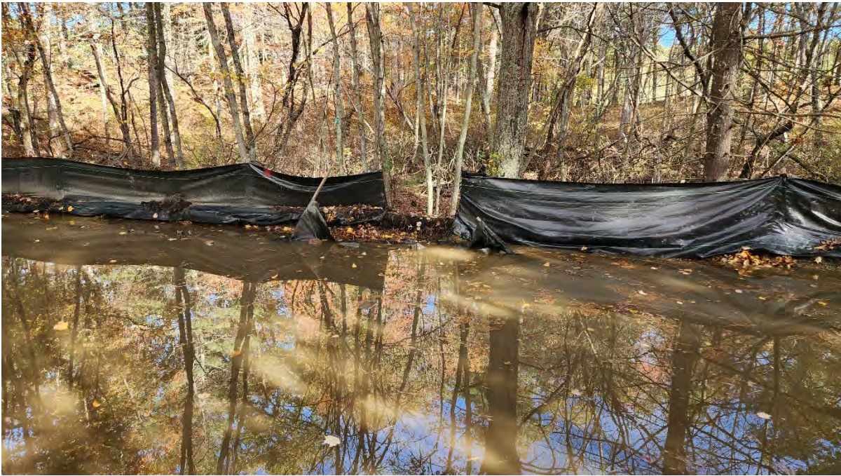
Photo 2: Rip in the silt fence in standing water along segment 8. Photo taken on 10/23/23
