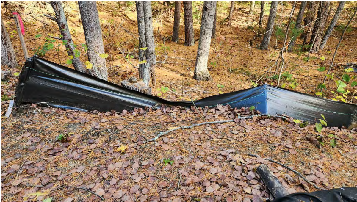
Photo 4: Broken stakes in the silt fence along segment 10. Photo taken on 10/23/23
