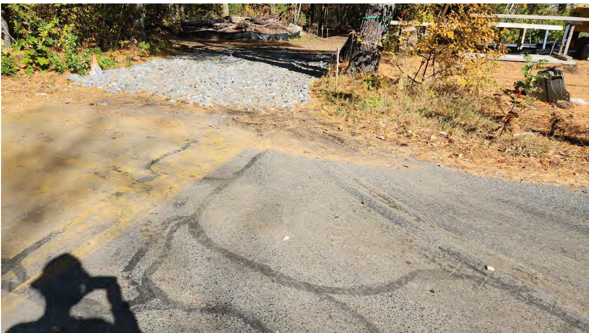
Photo 5: Sediment tracked into the road at construction entrance STA 407+50. Photo taken on 10/23/23
