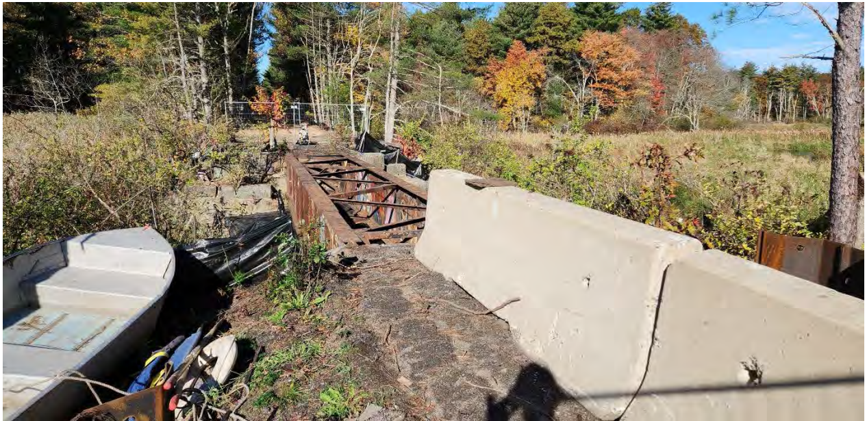
Photo 1: Bridge 128 closed. Photo taken on 10/23/23
