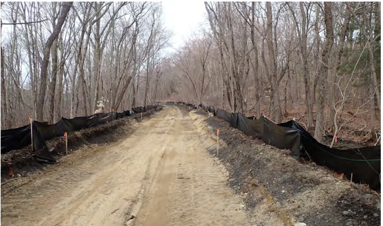
Photo #8: View of construction right-of-way with vernal pool #13 on the right and vernal pool #14 on the left in Segment 14. Silt fence in good condition. No sediment or debris observed in the resource area or associated buffer zones. Facing west.
