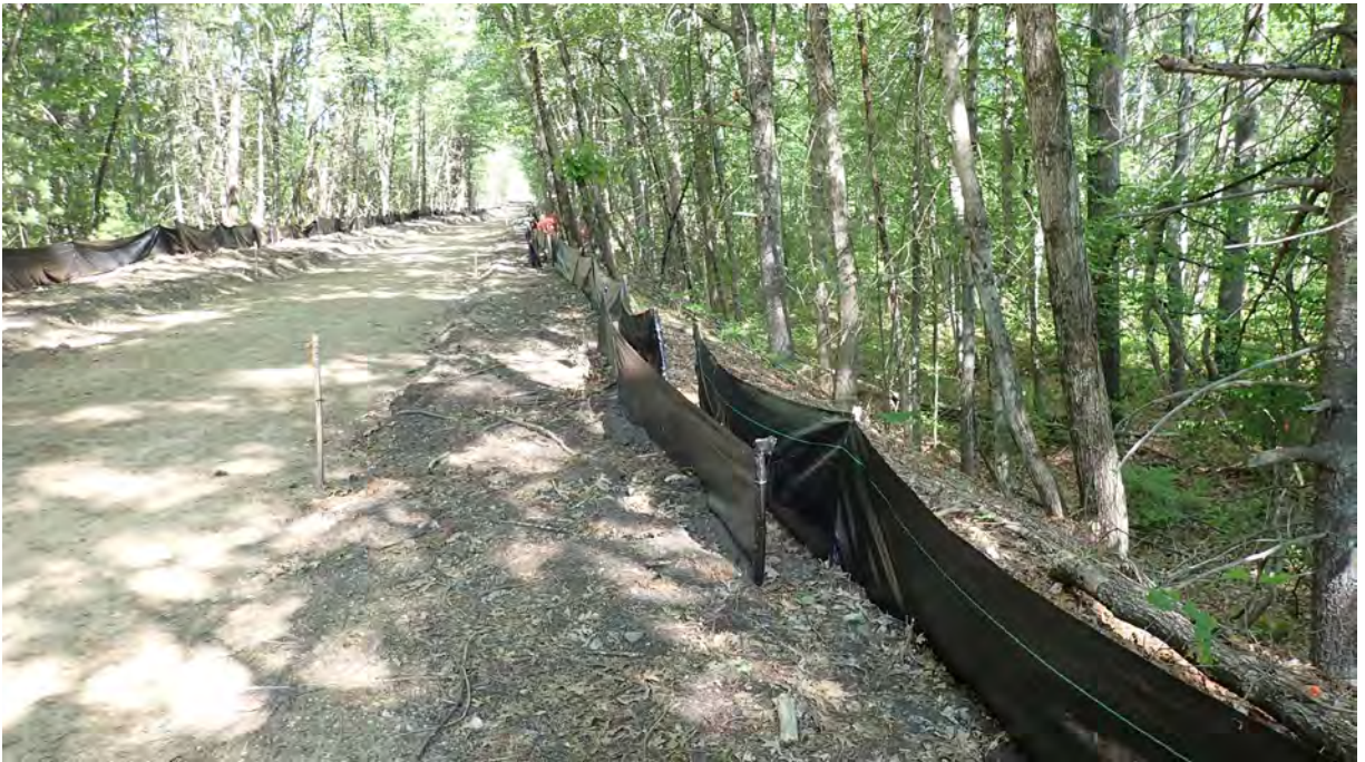
Photo #1: View of project area near vernal pools #7 in Segment 8. Silt fencing here, and throughout the project area, is in good condition. No sediment or debris observed within the resource area, buffer zone, or project area. Facing northwest.
