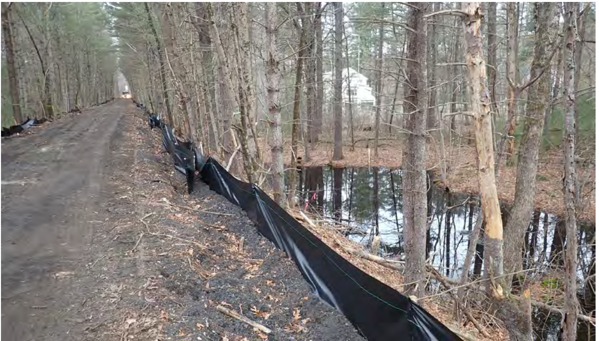
Photo #6: View of vernal pool #9 in Segment 9. Silt fence in good condition. No sediment or debris observed in the resource area or associated buffer zones. Facing northwest.
