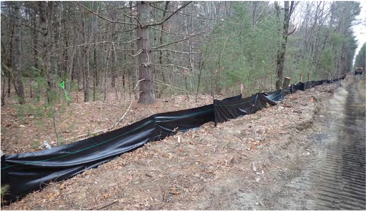
Photo #1: View of silt fence separating vernal pool #1 and the limit of work in Segment 7. Silt fence is in good condition. No sediment or debris observed within the resource area. Facing southeast.
