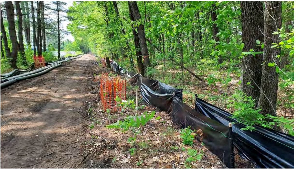
Photo #3: View of project area near vernal pool #11 in Segment 11. Silt fence in good condition. No sediment or debris observed in the resource area or associated buffer zone. Facing northwest.
