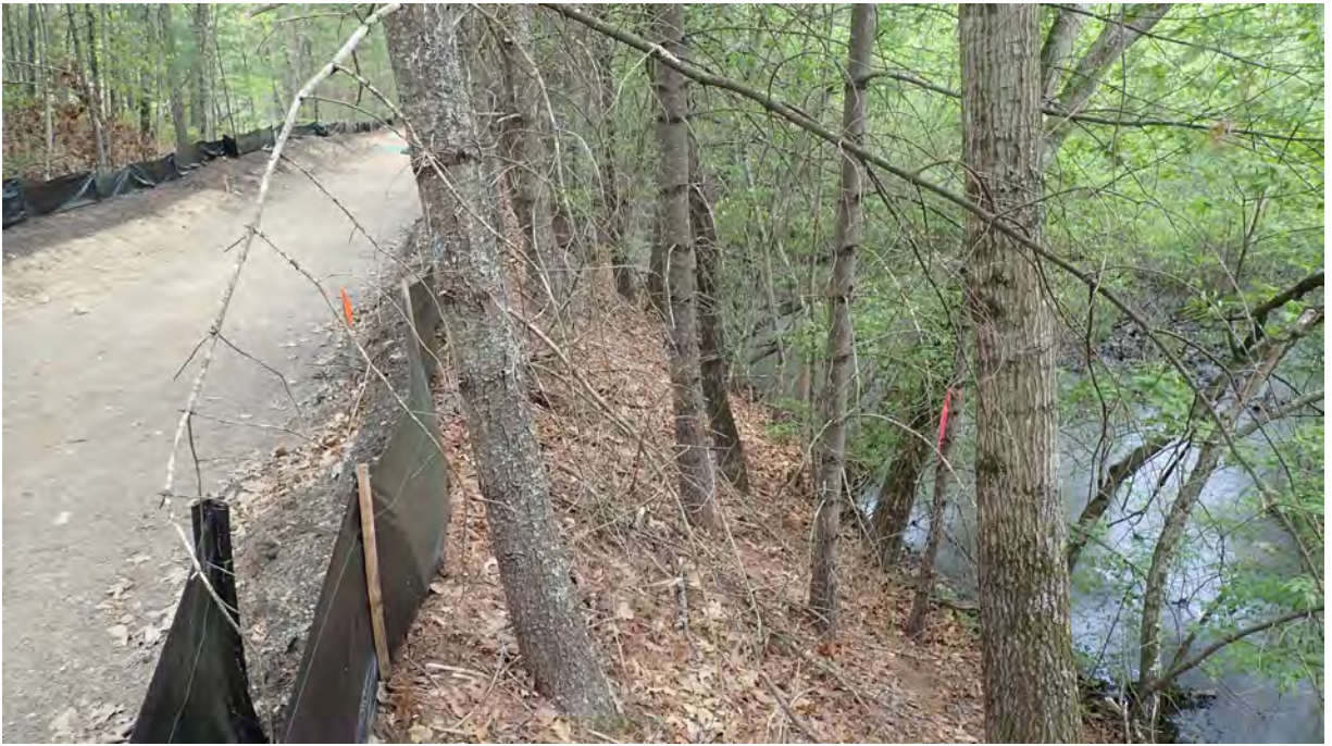
Photo #1: View of project area near vernal pools #5 in Segment 8. Silt fence is in good condition. No sediment or debris observed within the resource area, buffer zone, or project area. Facing southeast.
