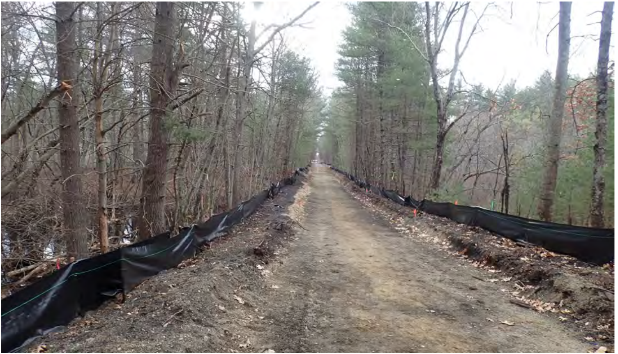
Photo #5: View of construction right-of-way with vernal pool #3 on the left and vernal pool #5 on the right in Segment 8. Silt fence in good condition. No sediment or debris observed in the resource area or associated buffer zones. Facing southeast.
