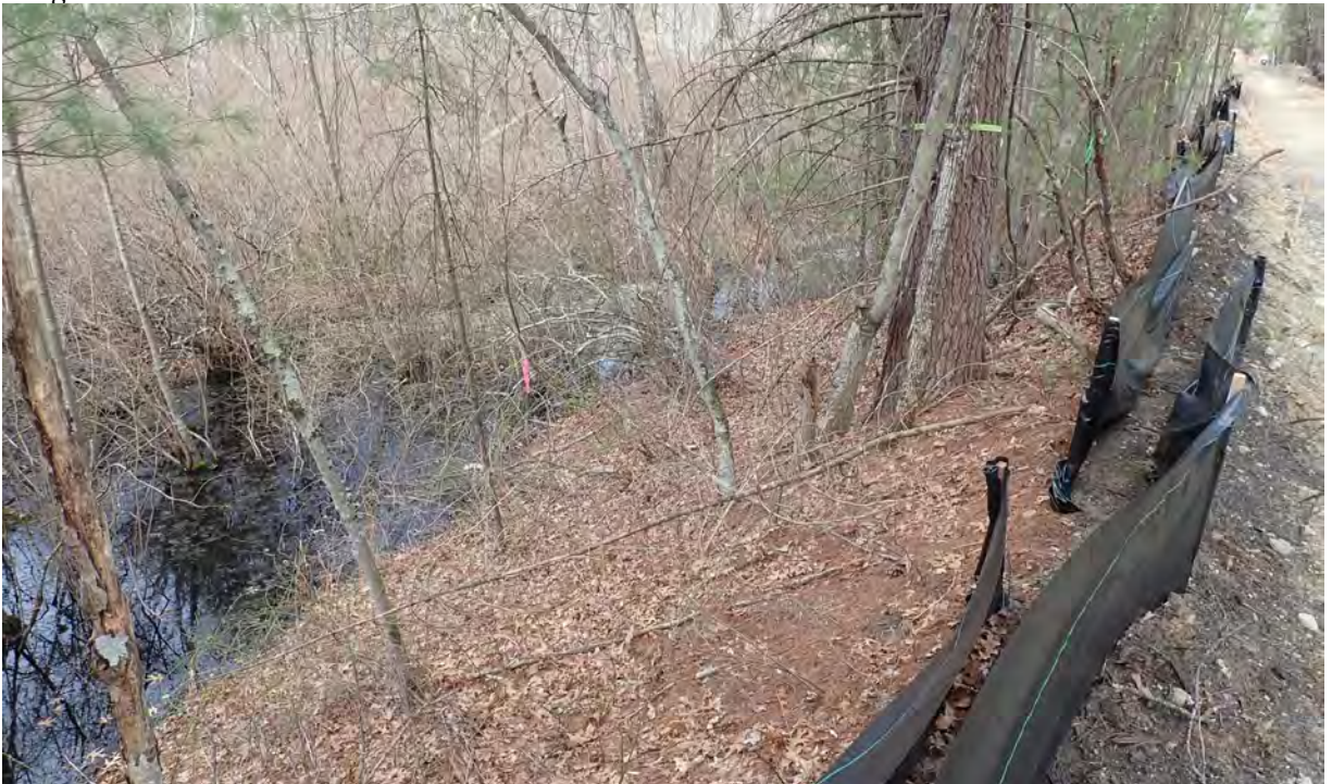
Photo #2: View of vernal pool #4 in Segment 8. No sediment or debris observed within the resource area or associated buffer zone. Silt fencing here and throughout the project area is in good condition. Facing southeast.
