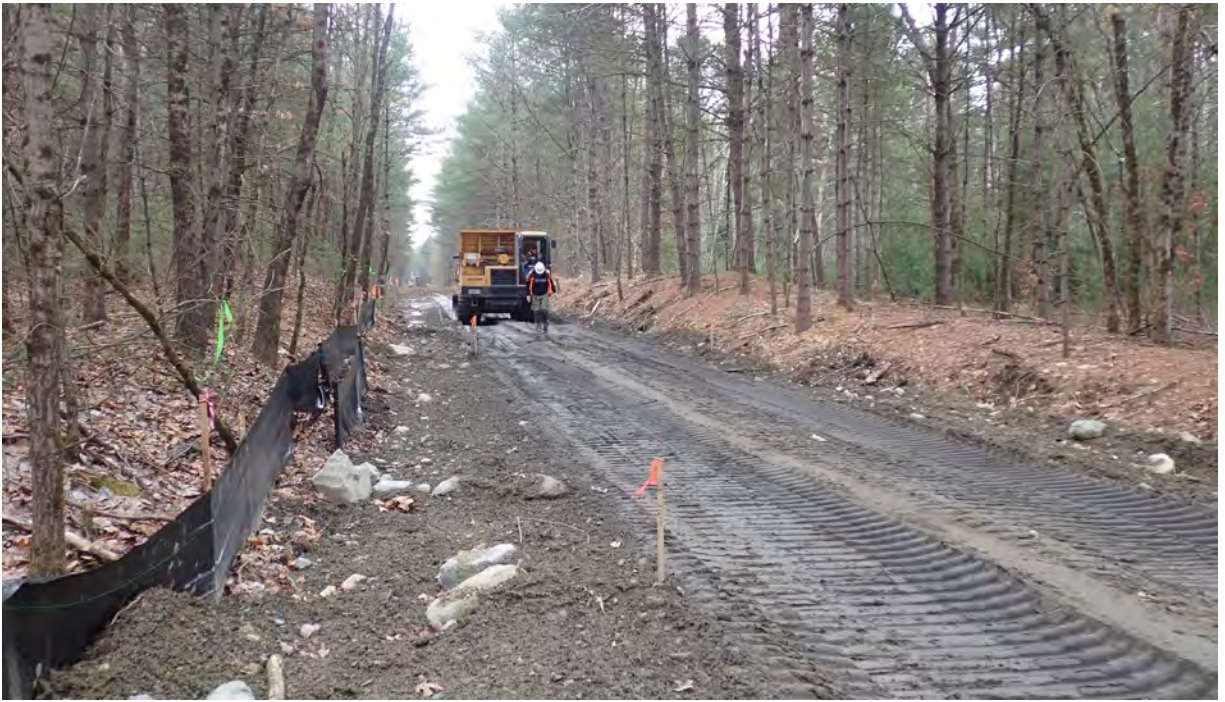
Photo #3: View of construction right-of-way near vernal pool #2 in Segment 7. Silt fence in good condition. No sediment or debris observed in the resource area or associated buffer zones. A monitor escorts construction vehicles through a portion of the right-of-way within vernal pool buffer zone. Facing southeast.
