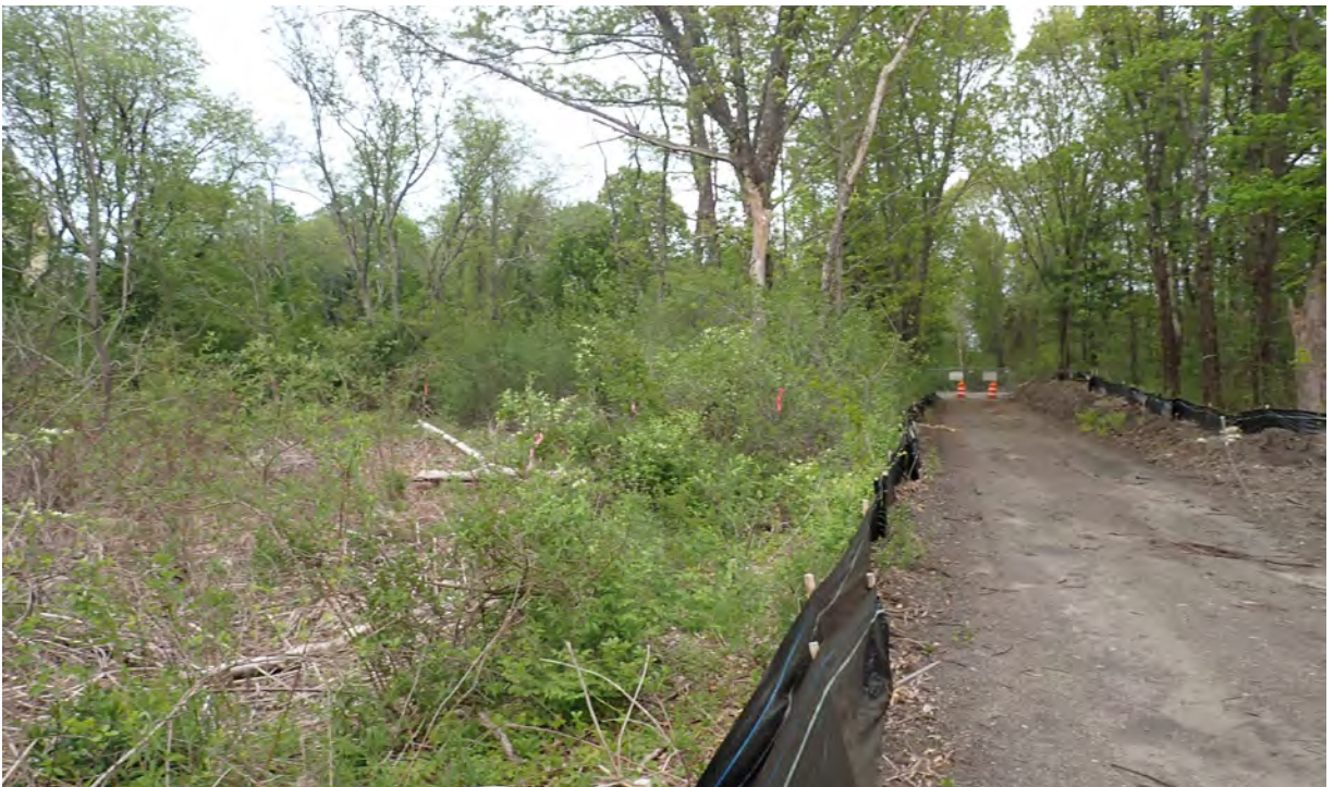
Photo #4: View of vernal pool #15 in Segment 14. Silt fence in good condition. No sediment or debris observed in the resource area or associated buffer zone. Facing east.
