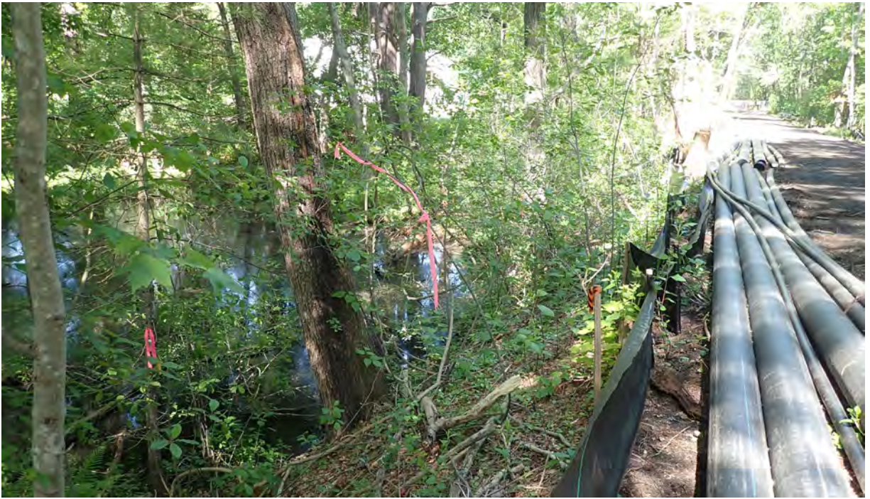
Photo #3: View of project area near vernal pool #10 in Segment 11. Silt fence in good condition. No sediment or debris observed in the resource area or associated buffer zone. Facing southeast.
