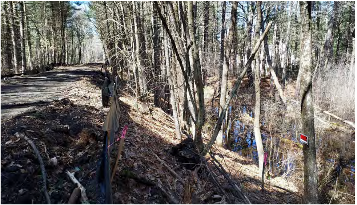
Photo #3: View of vernal pool #8 in Segment 10. Silt fence in good condition. No sediment or debris observed in the resource area or associated buffer zones. Facing northwest.
