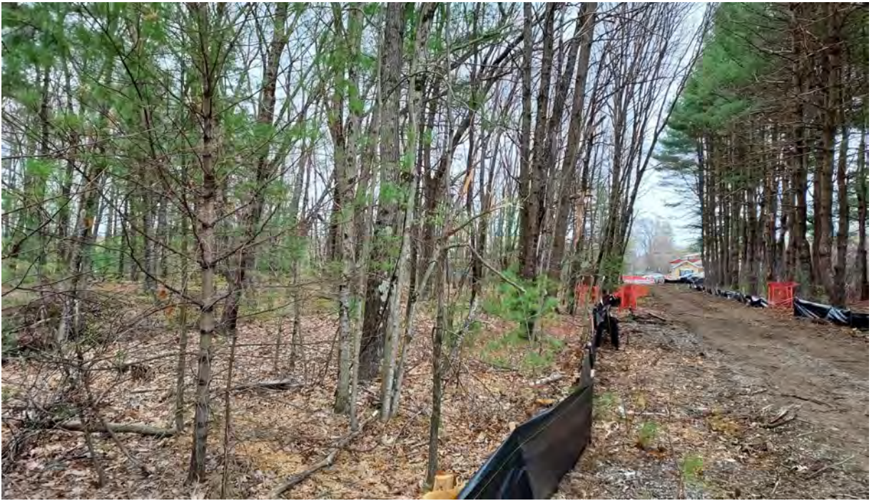
Photo #3: View of vernal pool #11 in Segment 11. Silt fence in good condition. No sediment or debris observed in the resource area or associated buffer zone. Facing southeast.
