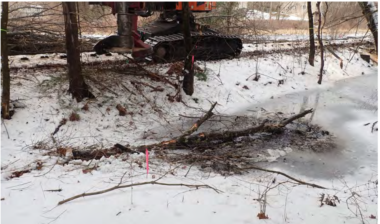
Photo #28: View of installed fallen log in Impact Area 16 near bridge crossing. Facing northeast.
