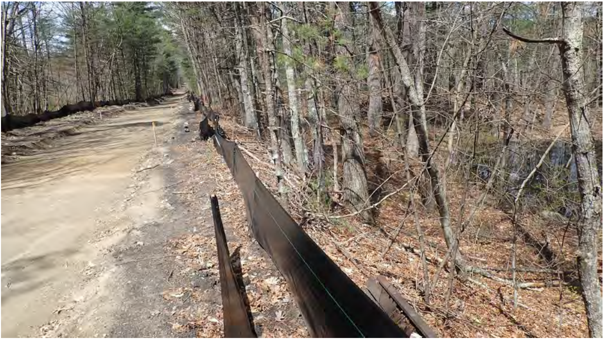
Photo #1: View of project area near vernal pool #6 and in Segment 8. Silt fence is in good condition. No sediment or debris observed within the resource area, buffer zone, or project area. Facing northwest.
