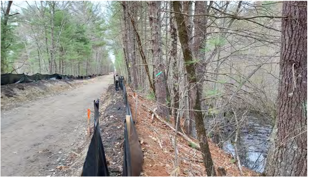
Photo #1: View of project area near vernal pool #5 and in Segment 8. Silt fence is in good condition. No sediment or debris observed within the resource area, buffer zone, or project area. Facing southeast.
