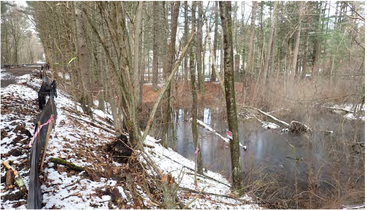
Photo #3: View of vernal pool #8 in Segment 9. Silt fence in good condition. No sediment or debris observed in the resource area or associated buffer zones. Facing northwest.
