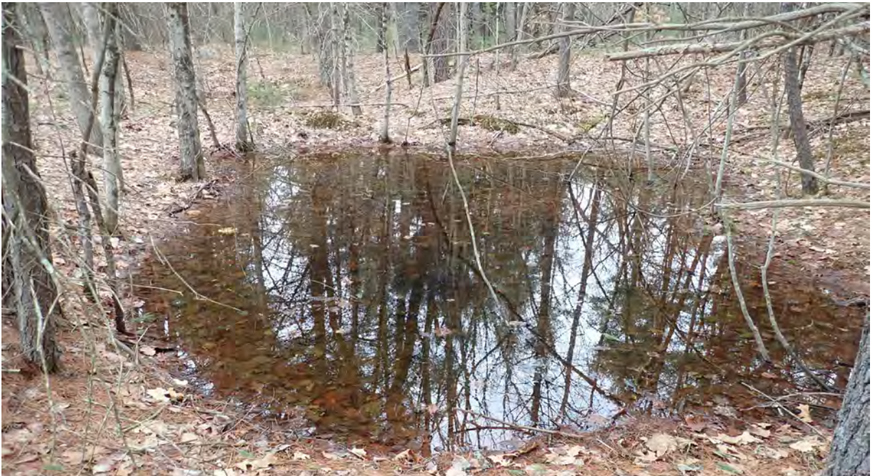
Photo #4: View of vernal pool #2 in Segment 7. Silt fence in good condition. No sediment or debris observed in the resource area or associated buffer zones. Facing north.
