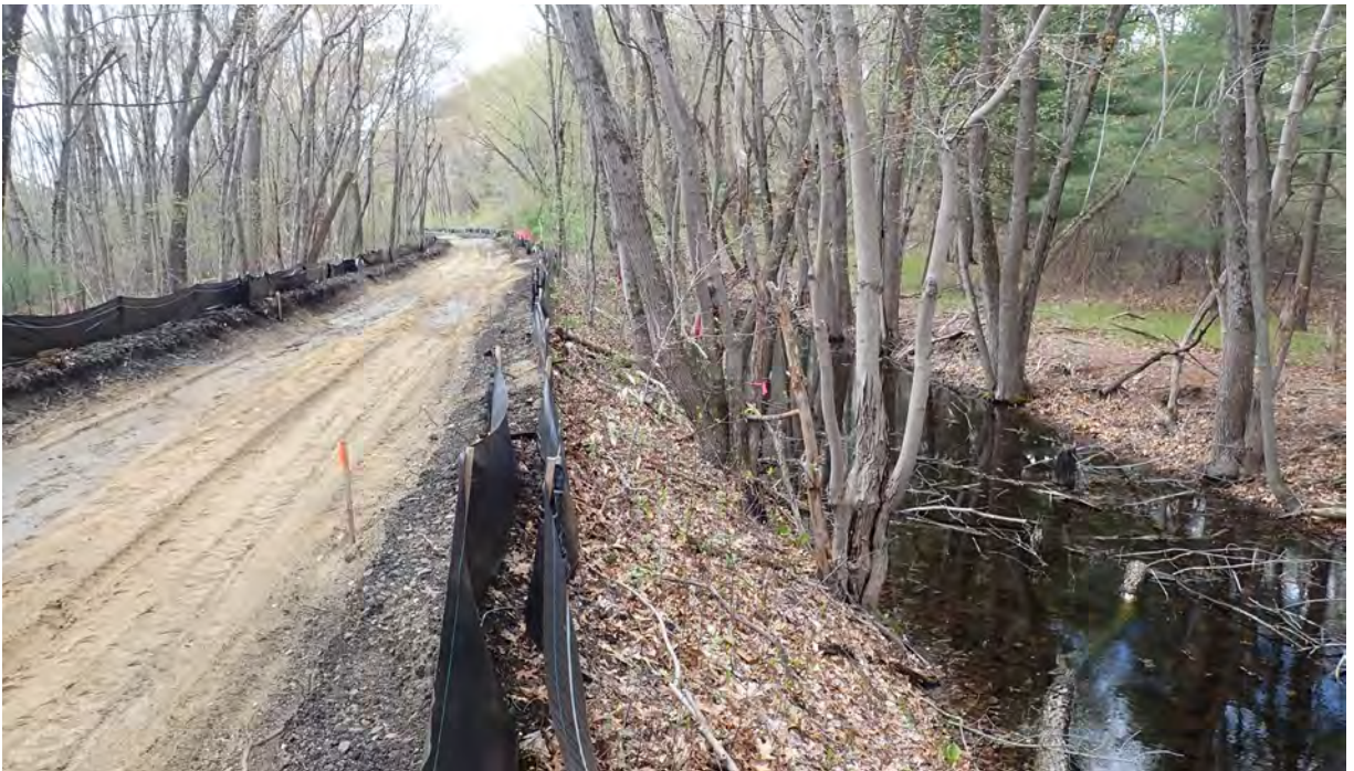
Photo #4: View of vernal pool #13 in Segment 14. Silt fence in good condition. No sediment or debris observed in the resource area or associated buffer zone. Facing west.
