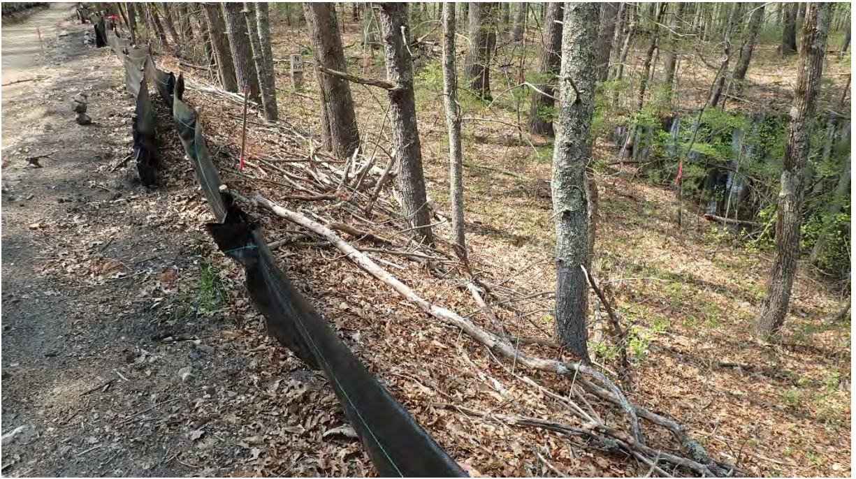
Photo #1: View of project area near vernal pools #6 in Segment 8. Silt fence is in good condition. No sediment or debris observed within the resource area, buffer zone, or project area. Facing north.
