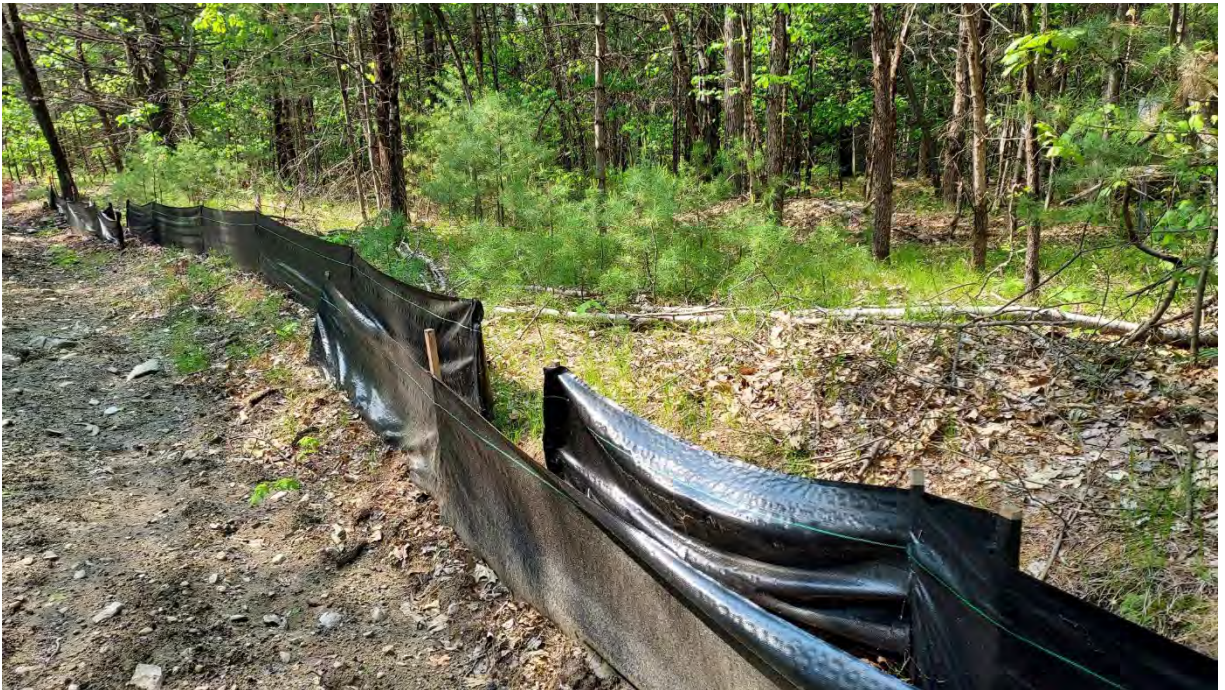
Photo #2: View of silt fence near vernal pool #2 in Segment 7. No sediment or debris observed within the resource area or associated buffer zone. Silt fencing here and throughout the project area is in good condition. Facing north.
