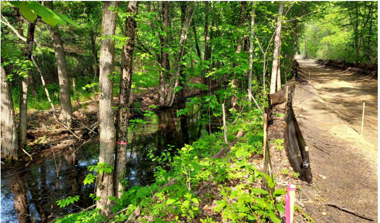
Photo #4: View of vernal pool #13 in Segment 14. Silt fence in good condition. No sediment or debris observed in the resource area or associated buffer zone. Facing east.
