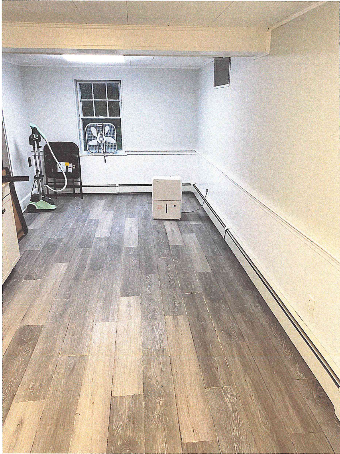
Semi-finished basement room primarily at ground level, which floods from the corners / sides of the room and up through the floorboards after significant rains. Drainage to be installed.
