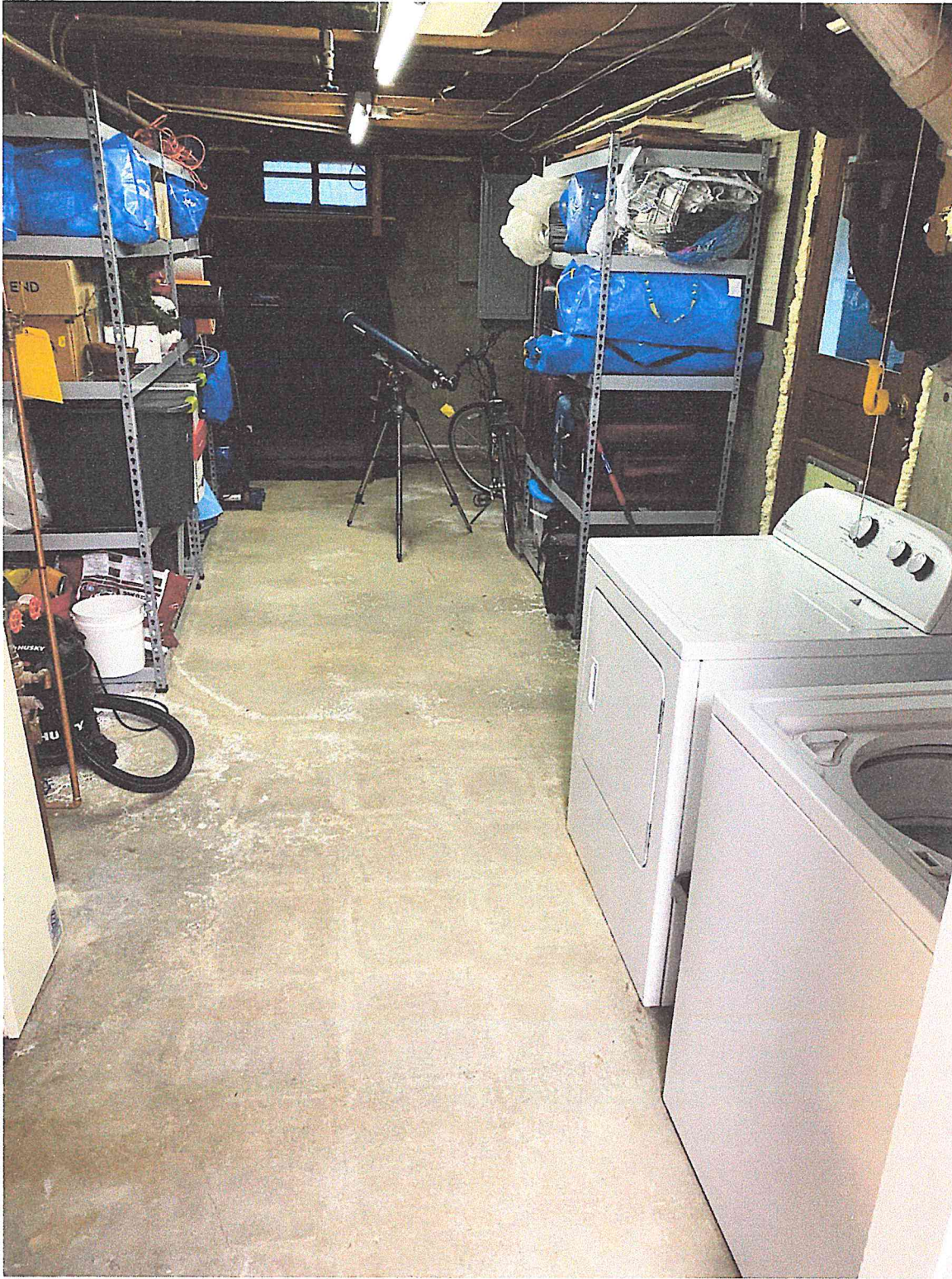
Unfinished utility room at ground level, which floods from the corners / sides of the room and up through the floor after significant rains. Sump pump would be installed near side door (right side of photo).
