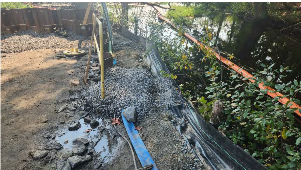
Photo 5: Broken stake in the silt fence near Bridge 127 along segment 13. Photo taken on 9/06/23
