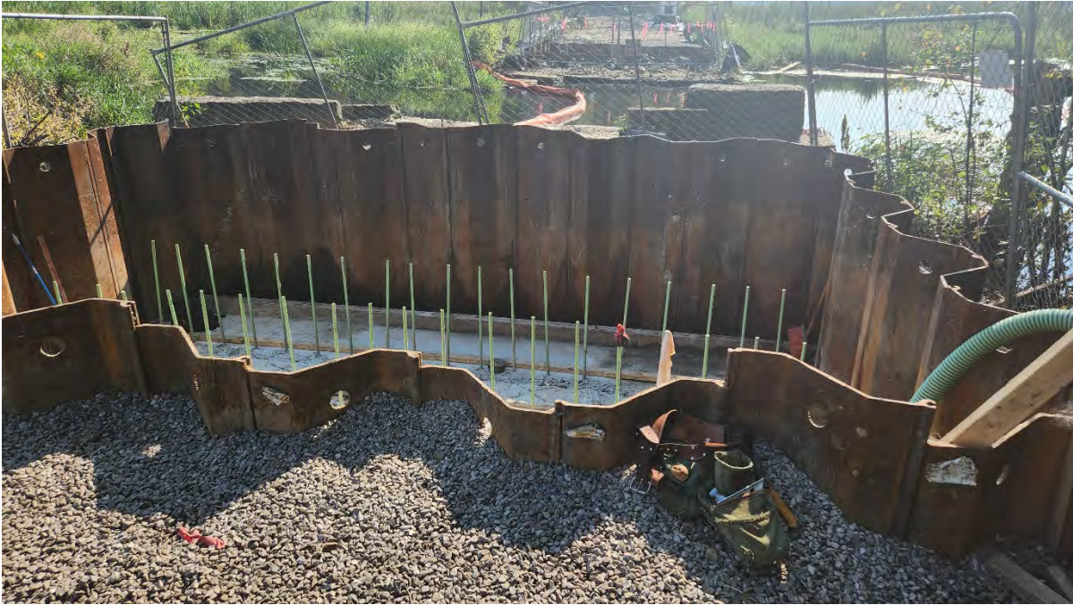
Photo 6: Form, rebar, and pour abutment wall being installed at Bridge 127. Photo taken on 9/06/23
