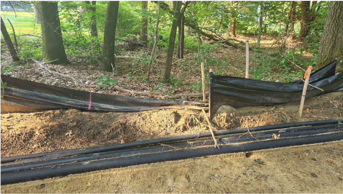
Photo 2: Broken stake in the silt fence along segment 10. Photo taken on 9/06/23
