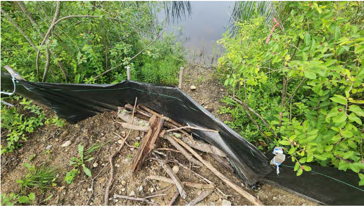
Photo 4: Debris piled up on the silt fence along segment 8 near Hop Brook Bridge. Sediment is washing under the silt fence and into Hop Brook. Photo taken on 7/19/23
