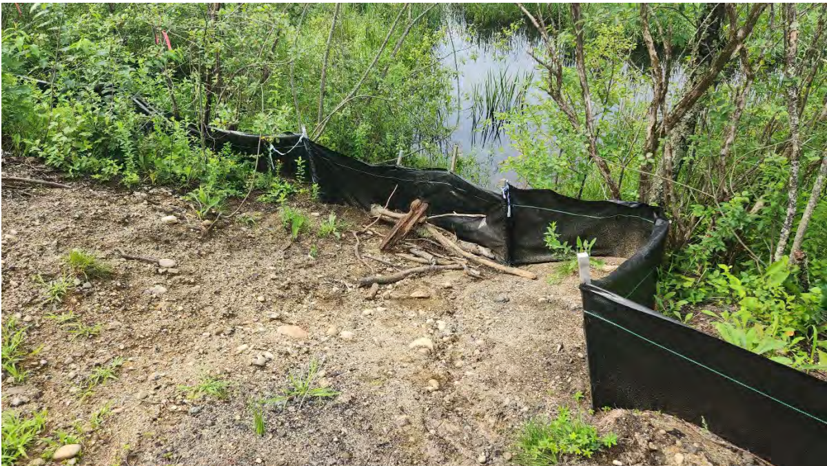
Photo 5: Debris piled up on the silt fence along segment 8 near Hop Brook Bridge. Sediment is washing under the silt fence and into Hop Brook. Photo taken on 7/19/23
