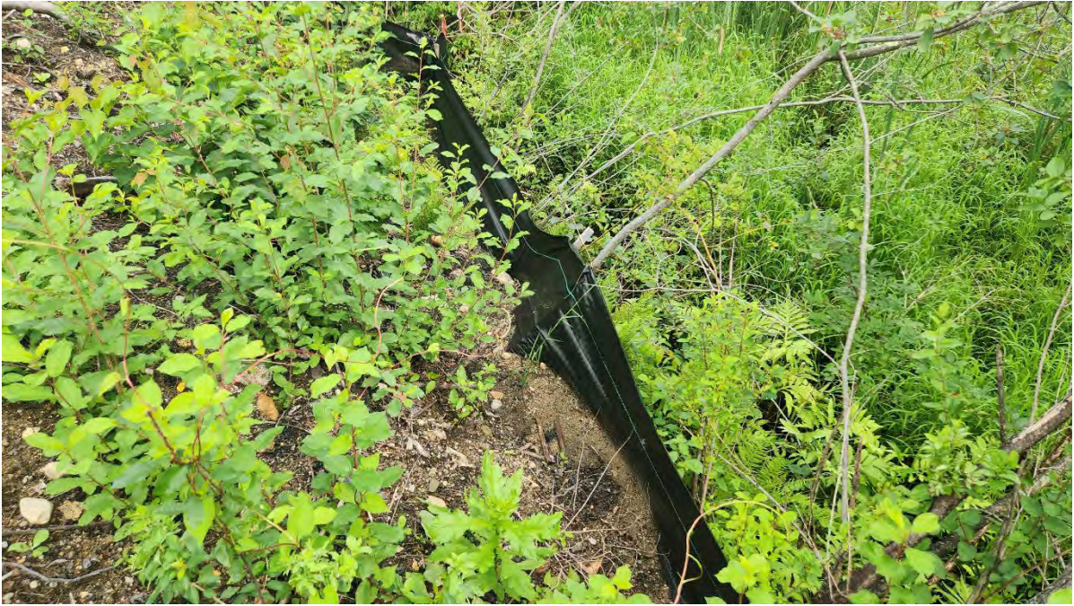
Photo 2: Broken stake in the silt fence along segment 8 near Hop Brook Bridge. Photo taken on 7/19/23
