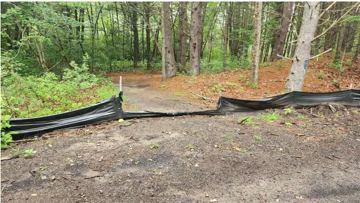
Photo 3: Rip in the silt fence along segment 8. Photo taken on 7/19/23
