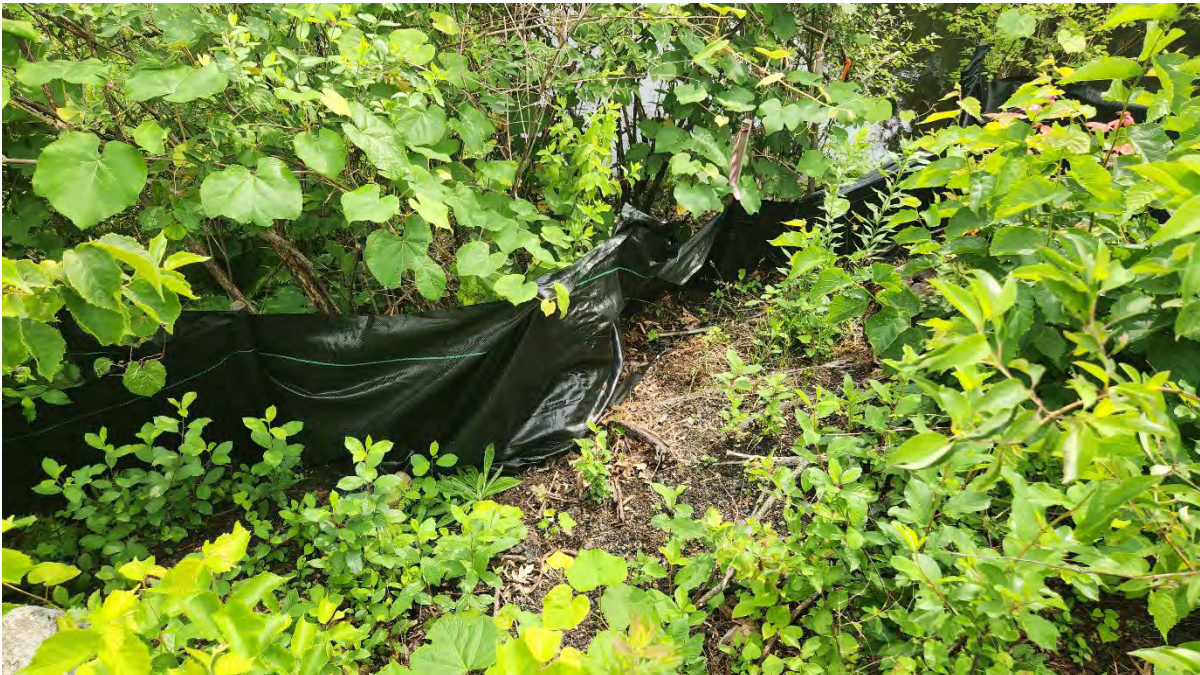
Photo 1: Broken stake and bagging in the silt fence along segment 7 near Hop Brook Bridge. Photo taken on 7/19/23
