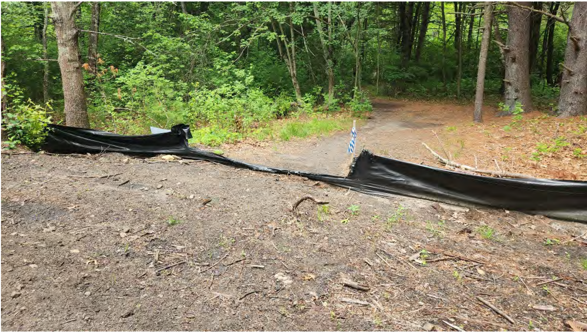
Photo 4: Rip in the silt fence along segment 8. Photo taken on 6/26/23
