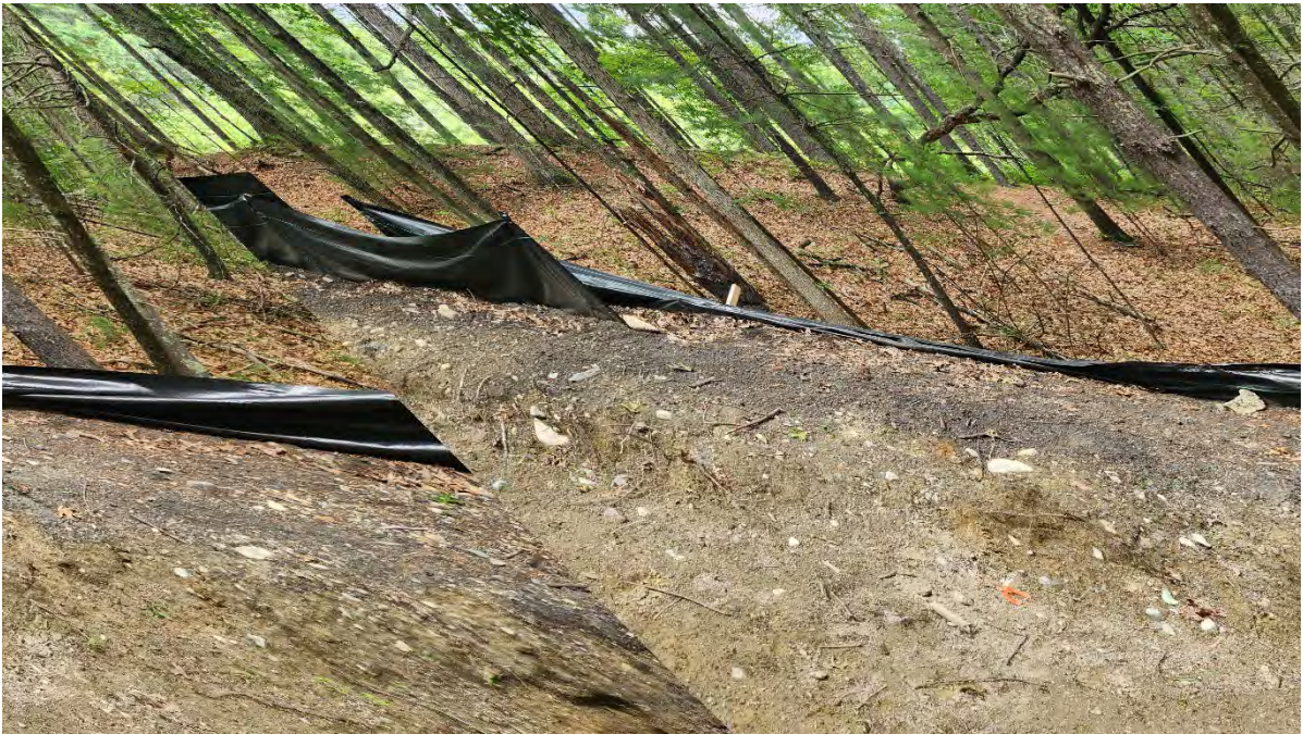
Photo 2: Broken stake in the silt fence along segment 8. Photo taken on 6/26/23
