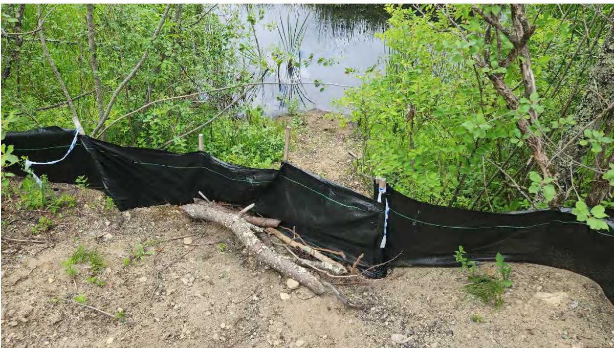
Photo 5: Debris piled up on the silt fence along segment 8 near Hop Brook Bridge. Sediment is washing under the silt fence and into Hop Brook. Photo taken on 6/26/23
