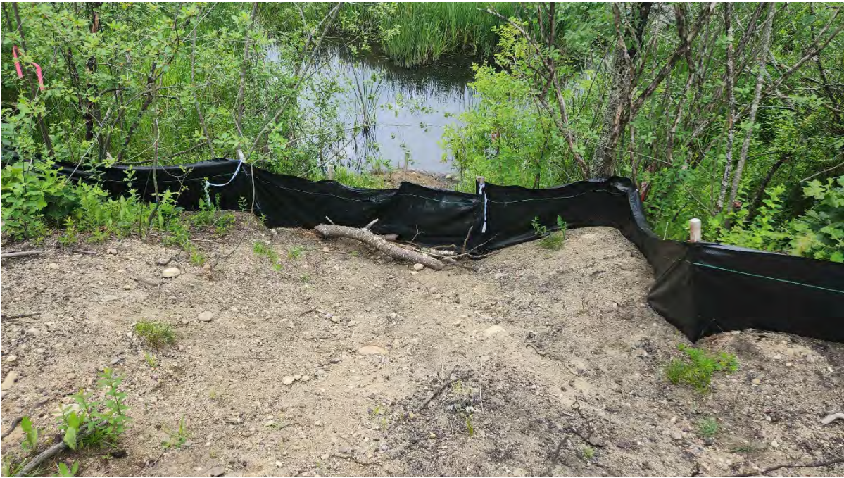
Photo 6: Debris piled up on the silt fence along segment 8 near Hop Brook Bridge. Photo taken on 6/26/23
