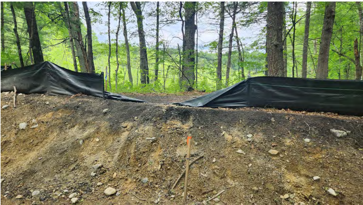
Photo 3: Rip in the silt fence along segment 8. Photo taken on 6/26/23
