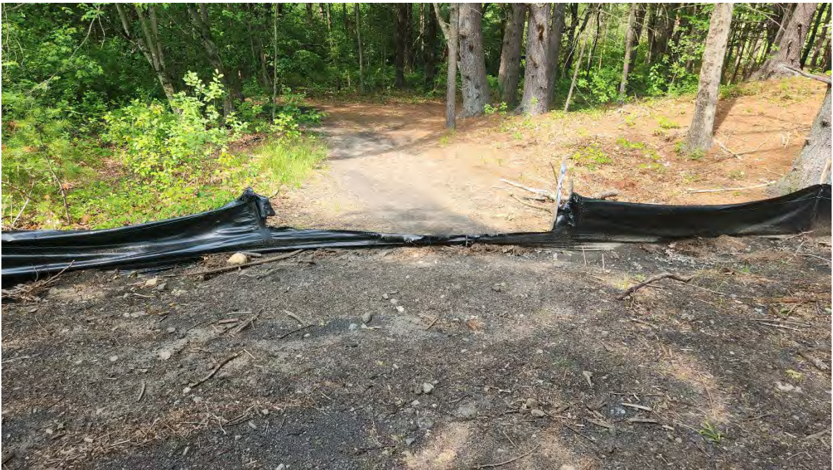
Photo 9: Rip in the silt fence along segment 8. Photo taken on 6/15/23
