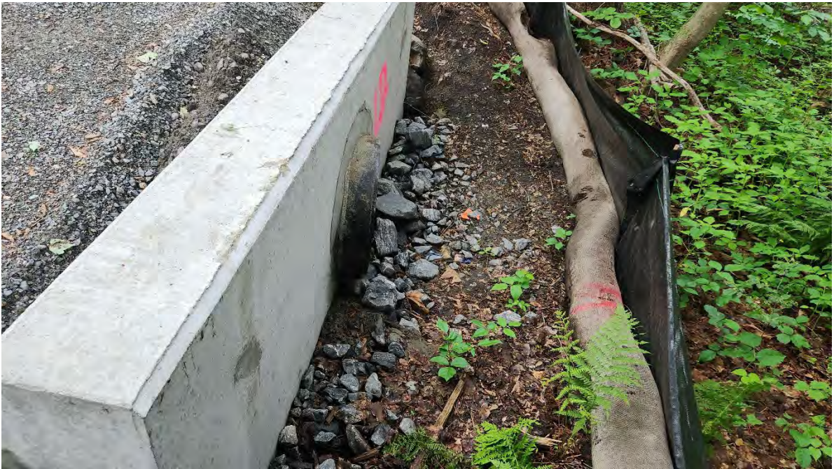
Photo 4: Silt fence and filter tube functioning properly next to installed culvert along segment 13. Photo taken on 6/15/23
