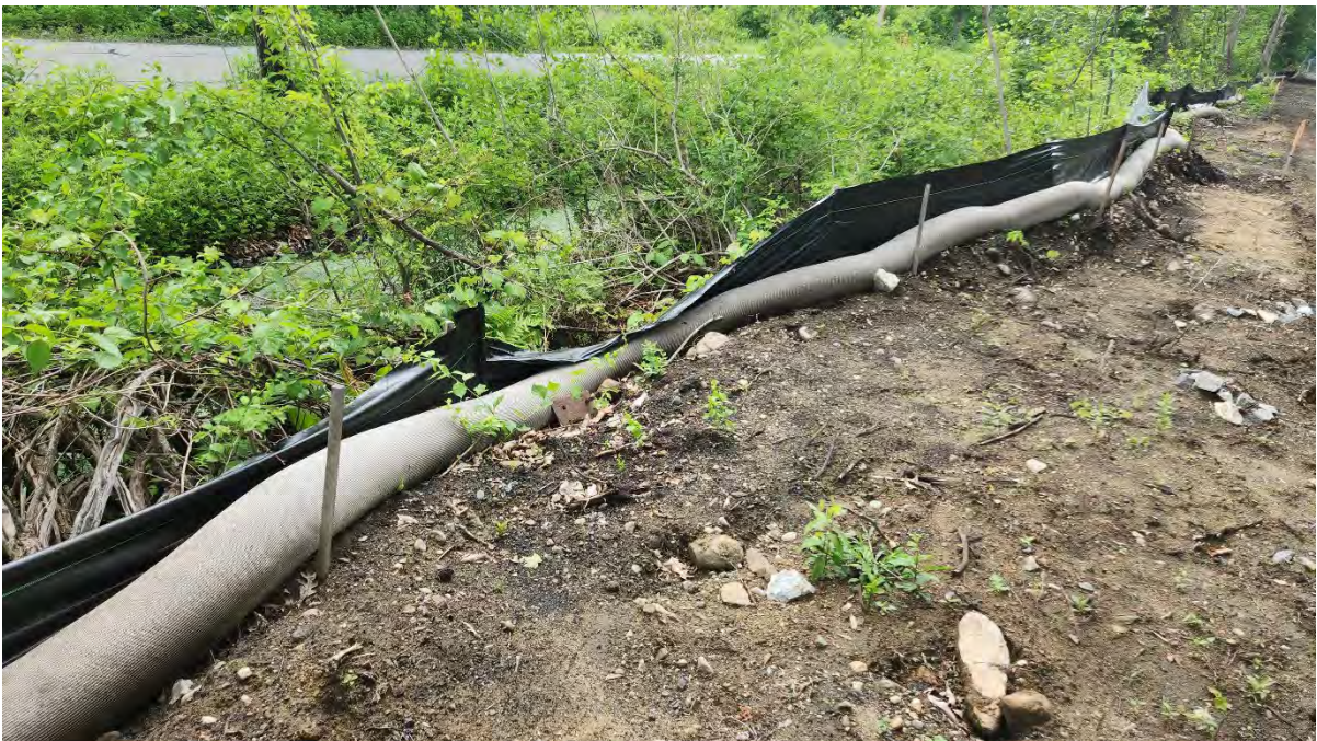
Photo 5: Silt fence and filter tube sagging along segment 12. Photo taken on 6/15/23
