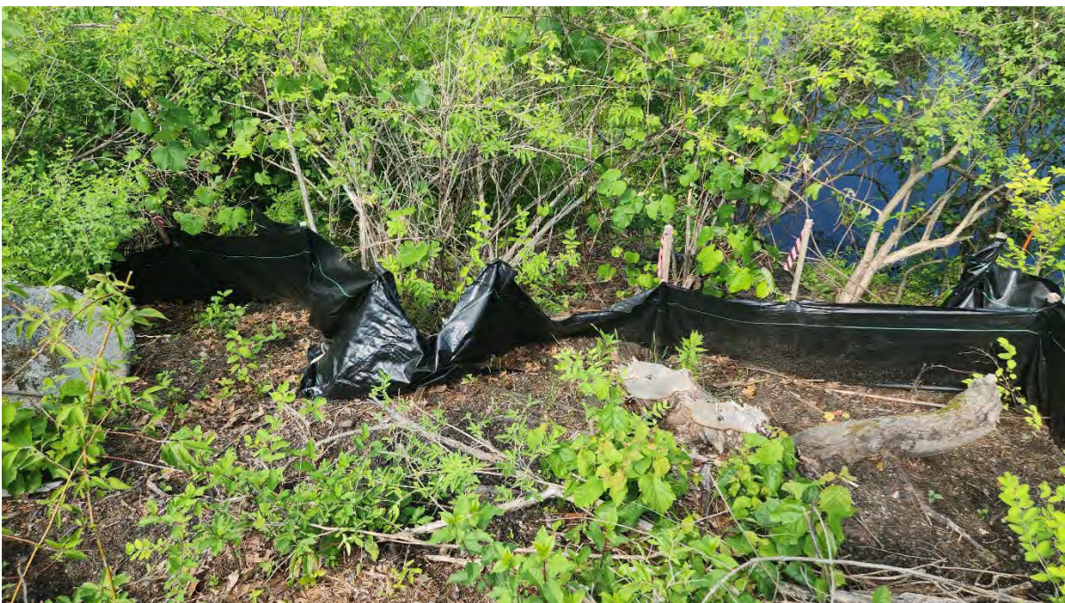
Photo 11: Broken stake in the silt fence along segment 7 near Hop Brook Bridge. Photo taken on 6/15/23
