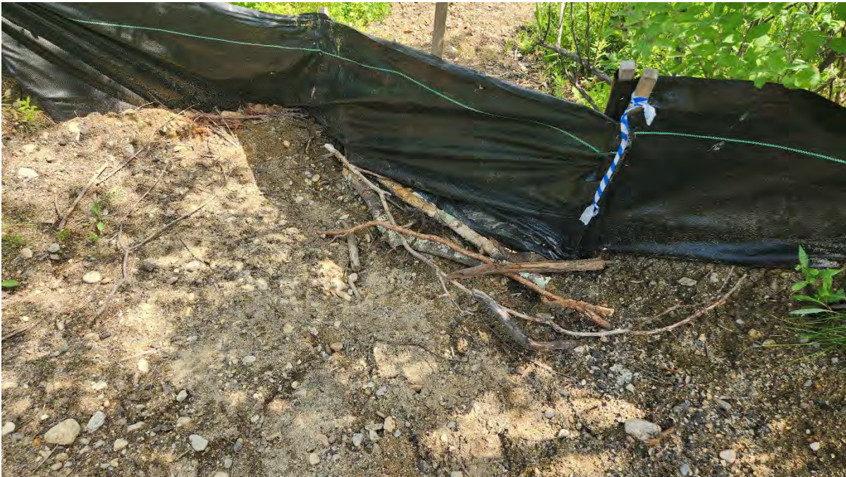
Photo 10: Debris pile up in the silt fence along segment 8 near Hop Brook Bridge. Photo taken on 6/15/23
