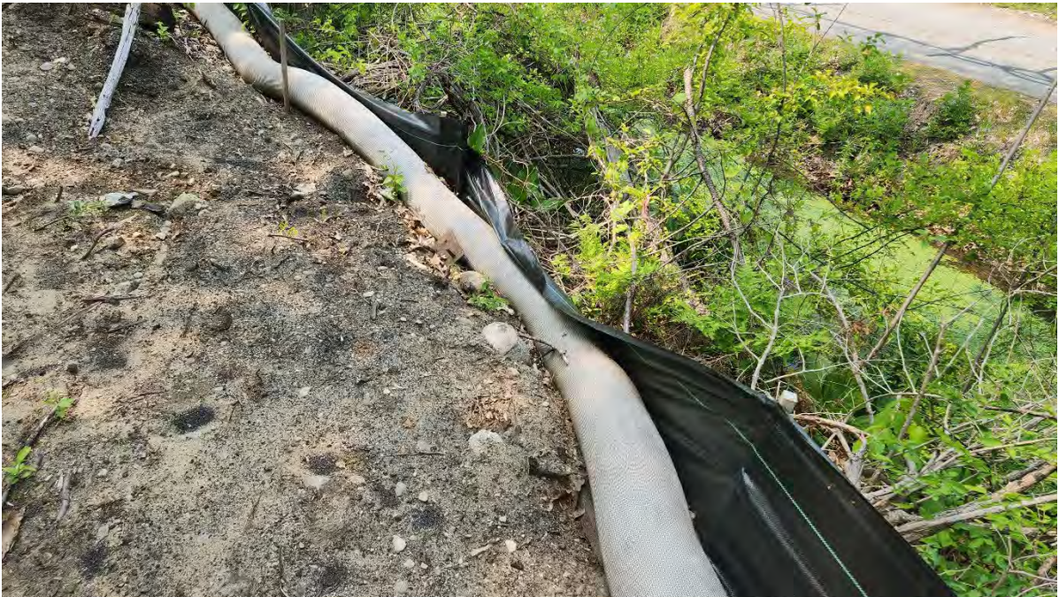
Photo 8: Broken stake in the silt fence along segment 9. Photo taken on 5/24/23
