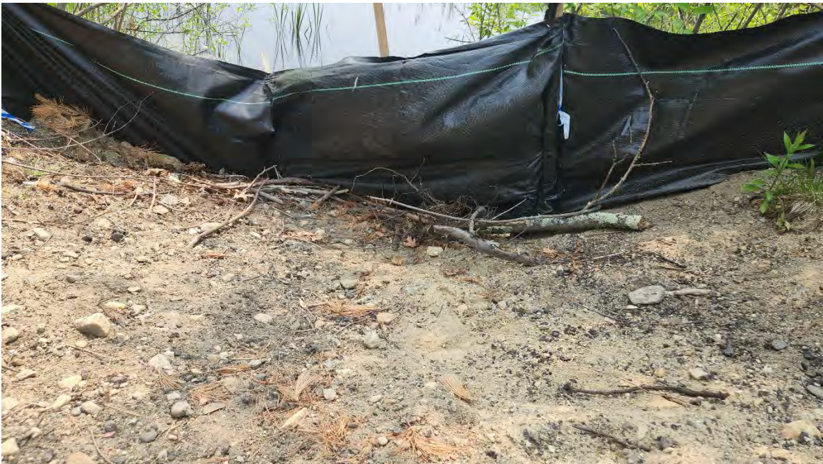
Photo 3: Debris accumulating and lifting of silt fence along segment 13 near Hop Brook Bridge. Photo taken on 5/24/23
