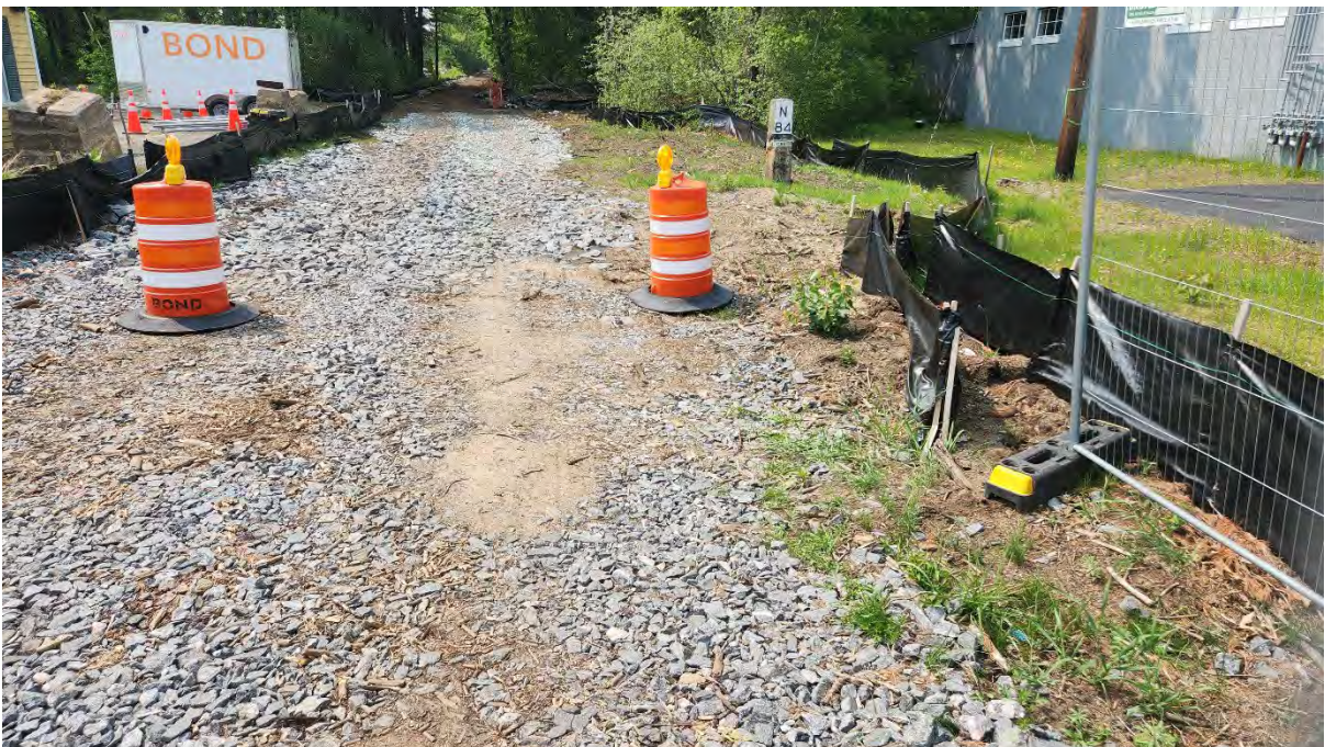
Photo 7: Construction entrance at STA 407+50 has visible sediment tracking onto the road. Photo taken on 5/24/23
