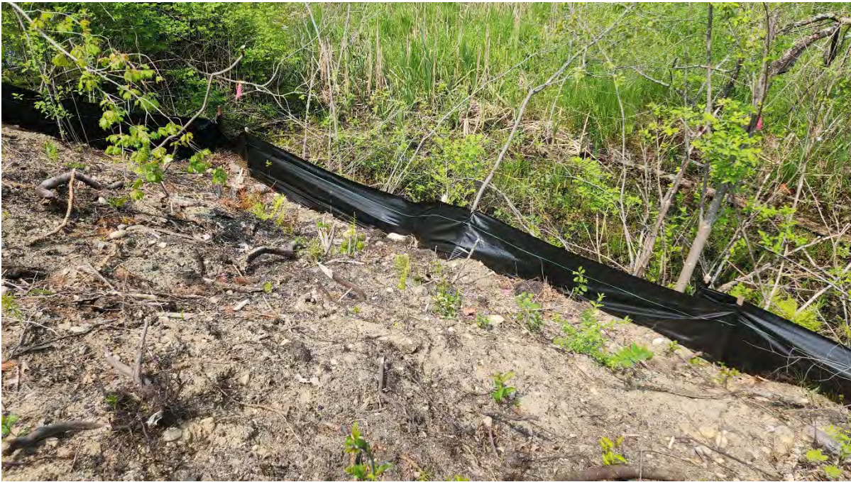
Photo 2: Broken stake in the silt fence along segment 13 near Hop Brook Bridge. Photo taken on 5/24/23
