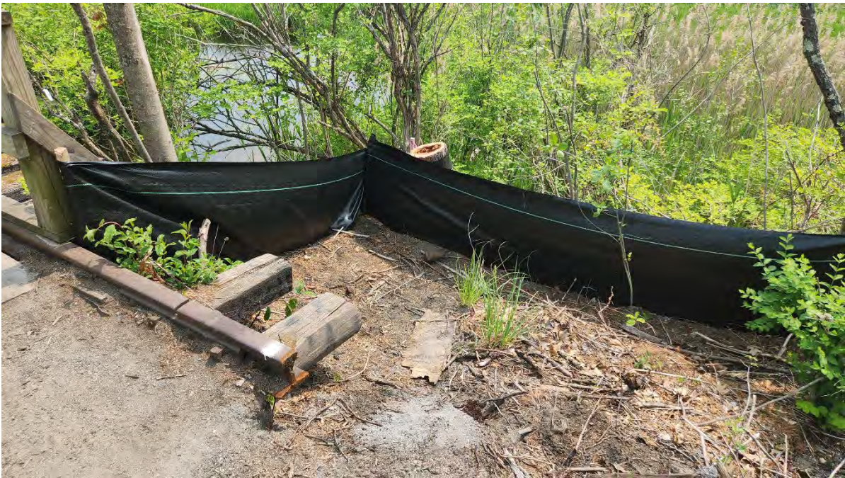
Photo 1: Silt fence and filter tube functioning properly along segment 14. Photo taken on 5/24/23
