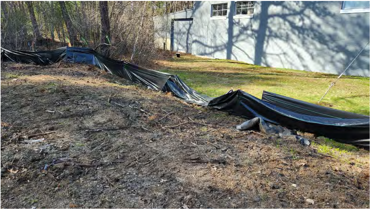
Photo 4: Broken stake in the silt fence along segment 11 near construction entrance STA407+50. Photo taken on 4/20/23
