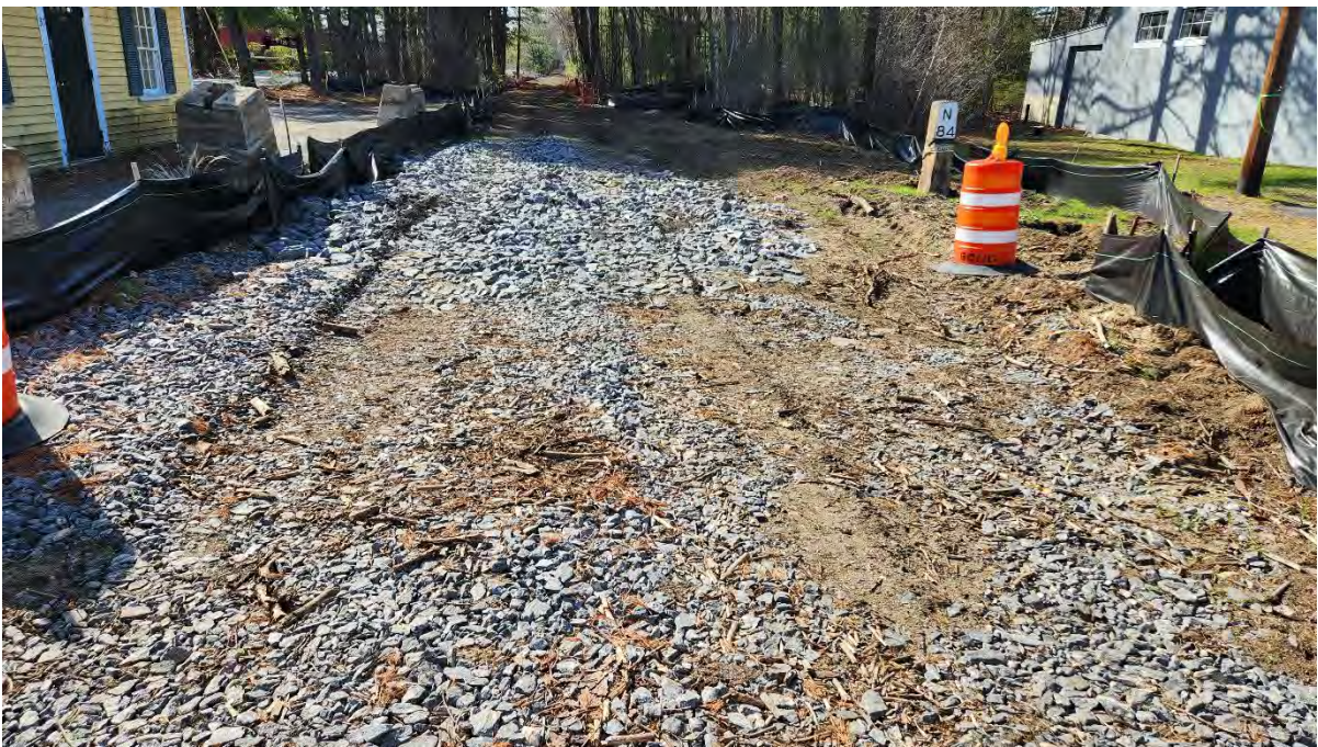
Photo 5: Construction entrance STA407+50 has visible dirt and should be monitored. Photo taken on 4/20/23
