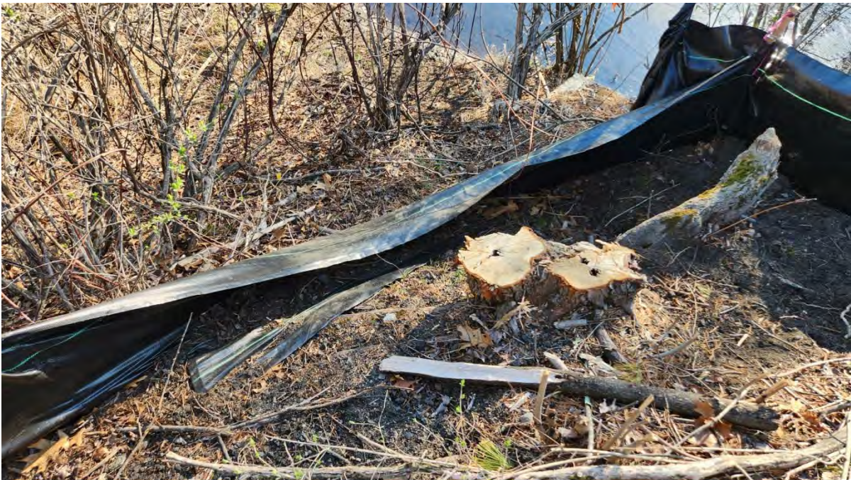
Photo 9: Silt fence sagging at Hop Brook Bridge along segment 7. Photo taken on 4/20/23
