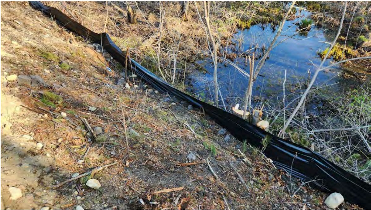
Photo 8: Silt fence sagging at Hop Brook Bridge along segment 8. Photo taken on 4/20/23
