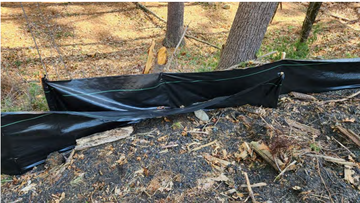
Photo 7: Silt fence sagging along segment 9 near construction entrance STA 335+50. Photo taken on 4/20/23
