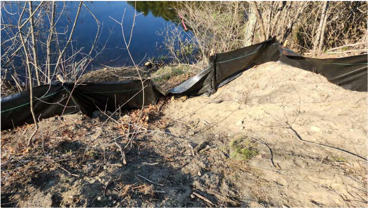
Photo 2: Notable sagging in the silt fence along segment 13 near Hop Brook Bridge. Photo taken on 4/20/23
