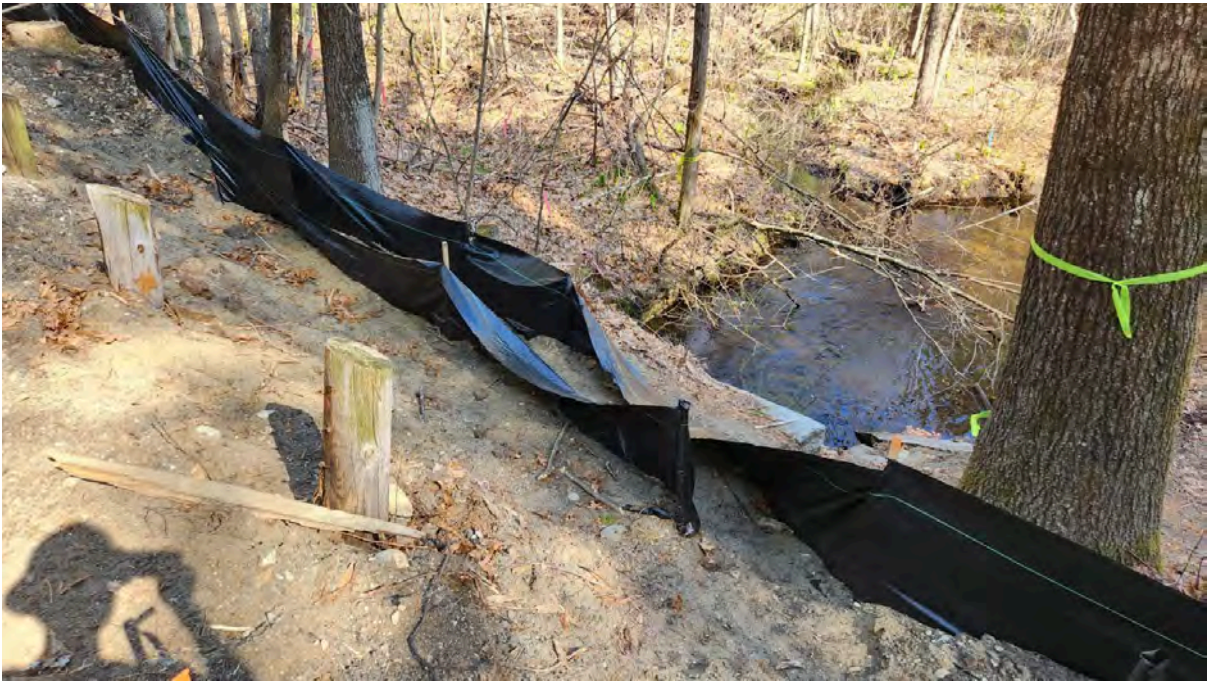
Photo 6: Silt fence sagging along segment 10 near Dudley Brook. Photo taken on 4/20/23
