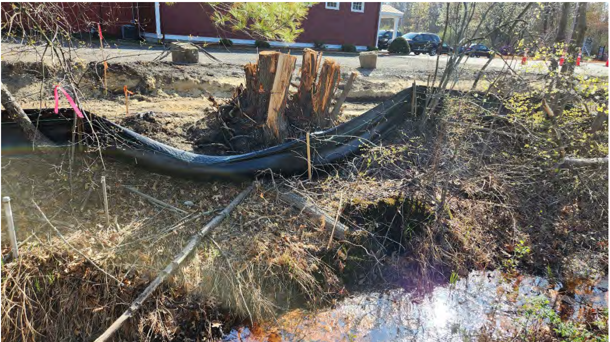
Photo 3: Notable sagging in the silt fence along segment 12. Photo taken on 4/20/23
